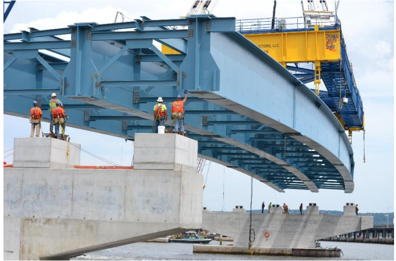
Figure 1. Tappan Zee Bridge steel girder assembly. Photo Credit: New York State Thruway Authority
