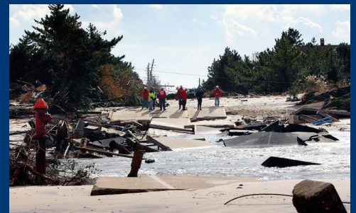
Damage on Route 35 in New Jersey following Hurricane Sandy. Photo credit: NJTPA
