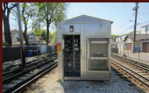
Signal house at Brown Line Rockwell Station that may be vulnerable to overheating during electricity outages. Photo credit: CTA.
