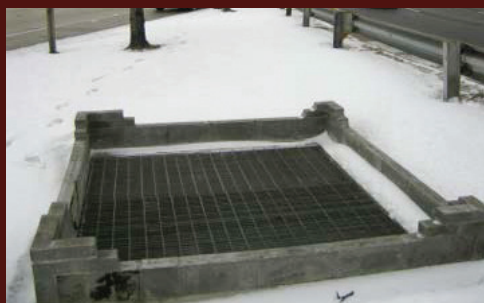
Overflow barrier around the O'Hare subway ventilation shaft to prevent flooding. Photo credit: CTA.
