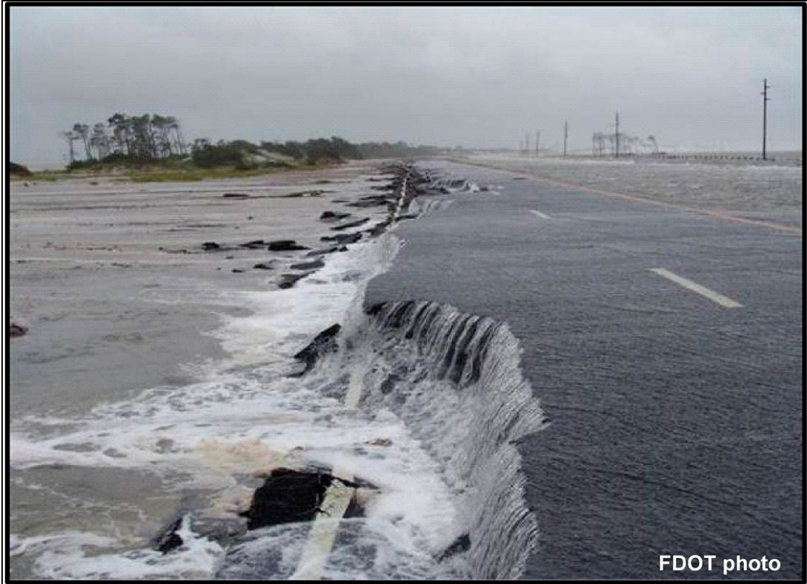
Figure 3.4. Example of the weir-flow damage mechanism as it occurs.
