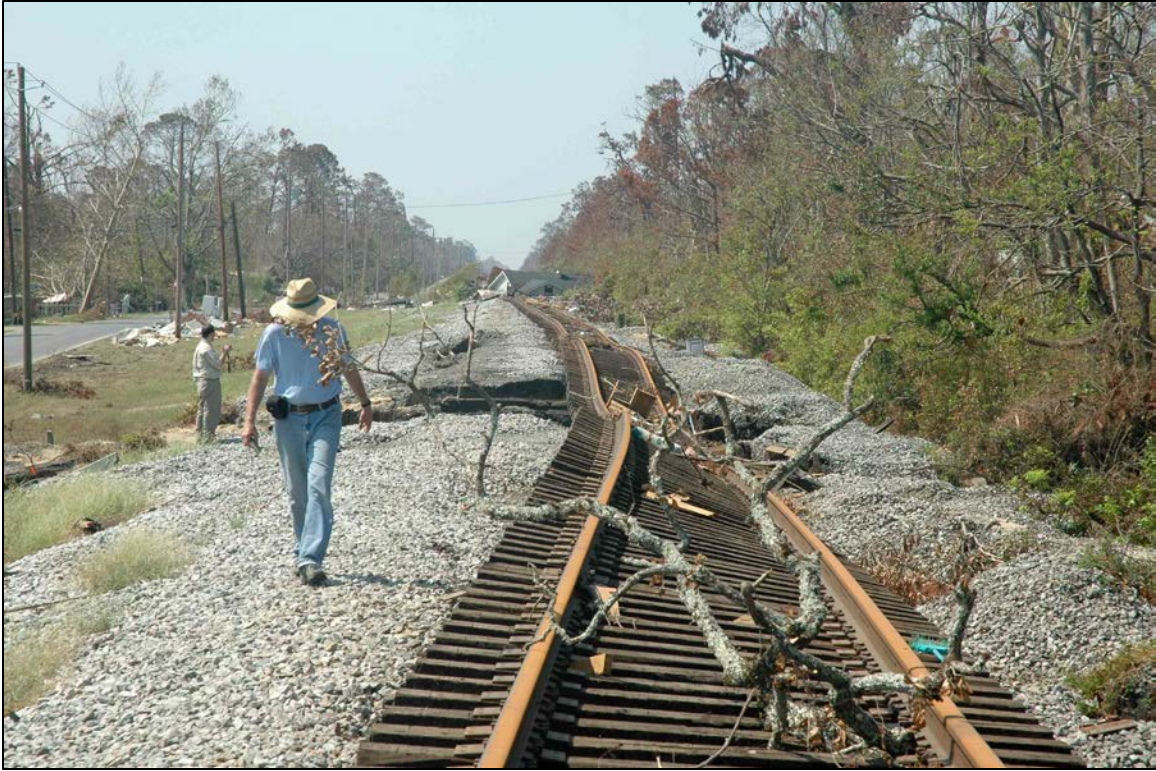
Figure 3.5. Railway embankment damage caused primarily by the weir-flow damage mechanism.
