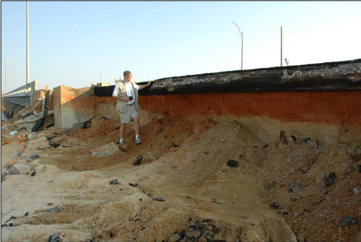
Figure 3.3. Partial embankment damage caused by wave attack.
