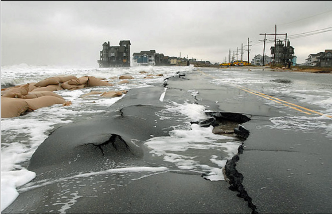
Figure 3.6. Pavement damage due to waves and surge in an extreme event (NC DOT photo).
