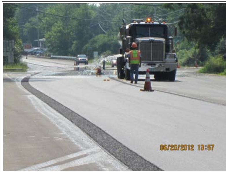
Figure 35. Recently placed WMA being artificially cooled with water to open the lane to traffic faster.
