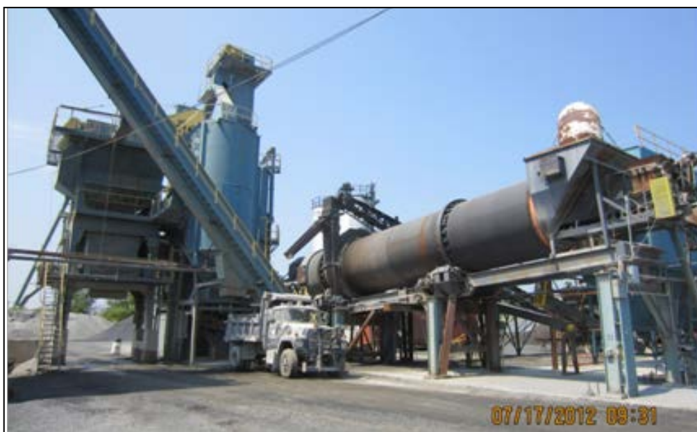
Figure 9. Peckham's drum mix plant in Hudson Falls, NY, used to produce WMA and HMA mixtures.
