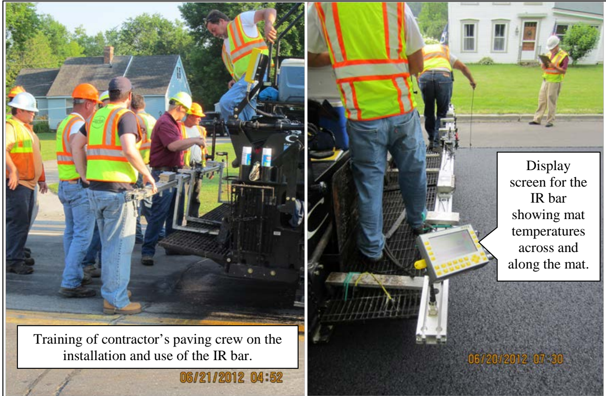
Figure 19. IR bar being installed and used to monitor mat temperatures directly behind the paver.
