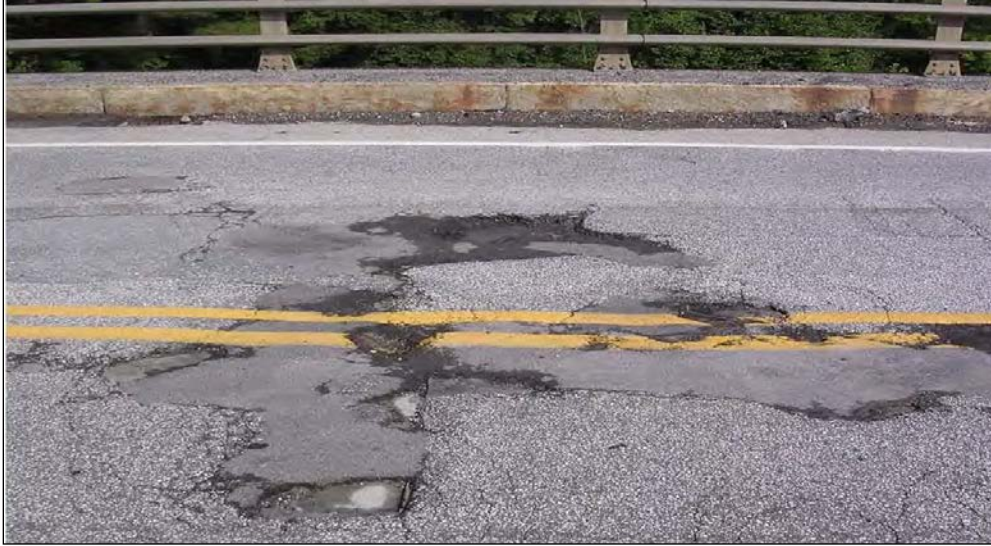
Figure 10. Failed membrane and pavement condition.
