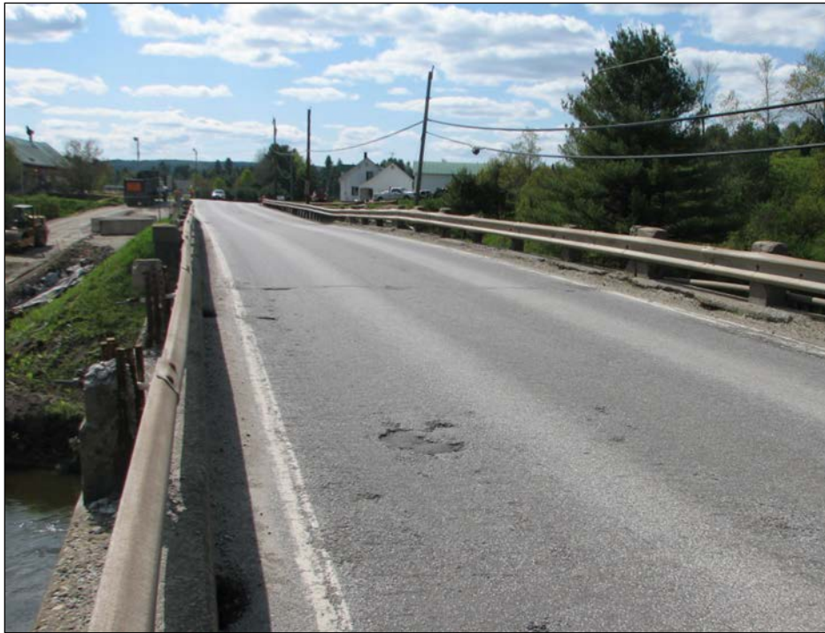
Figure 3. Deteriorated bridge deck.
