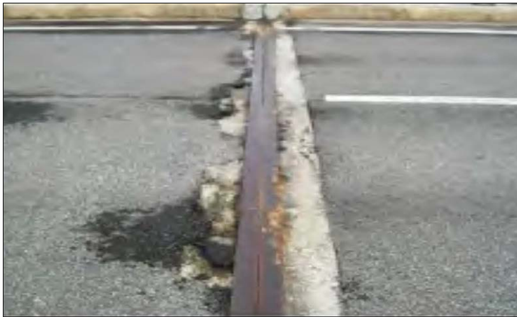
Figure 11. Failed deck joint condition.
