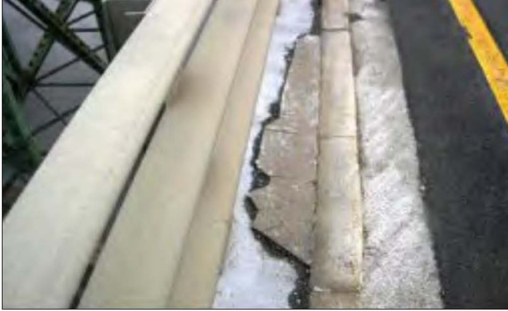
Figure 12. Salt-laden runoff at curb.
