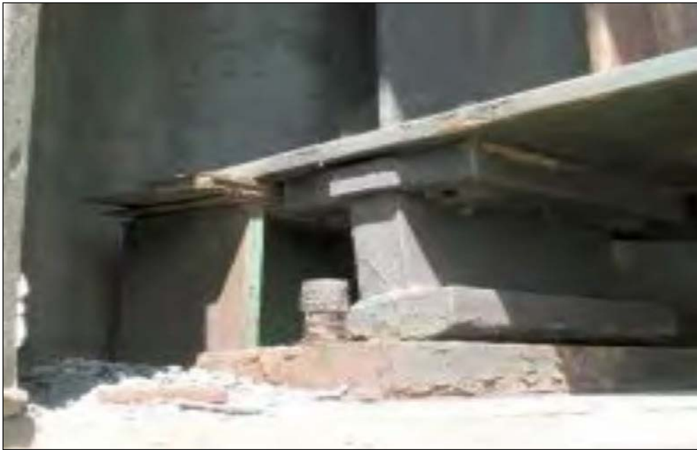
Figure 13. Corroded bearing condition.
