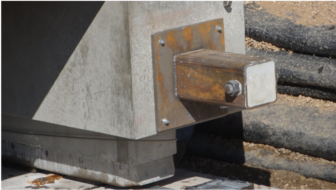
Figure 47. Photo. Cable termination point.
