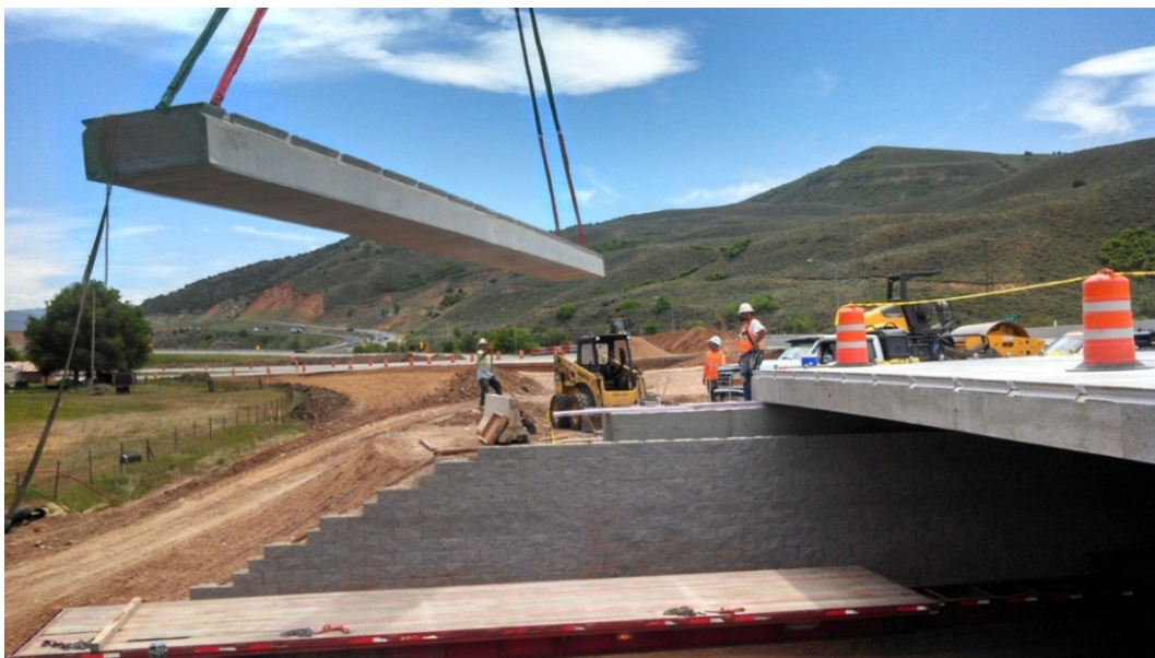
Figure 37. Photo. Bridge deck elements being moved to the bridge location using a crane (courtesy: UDOT).
