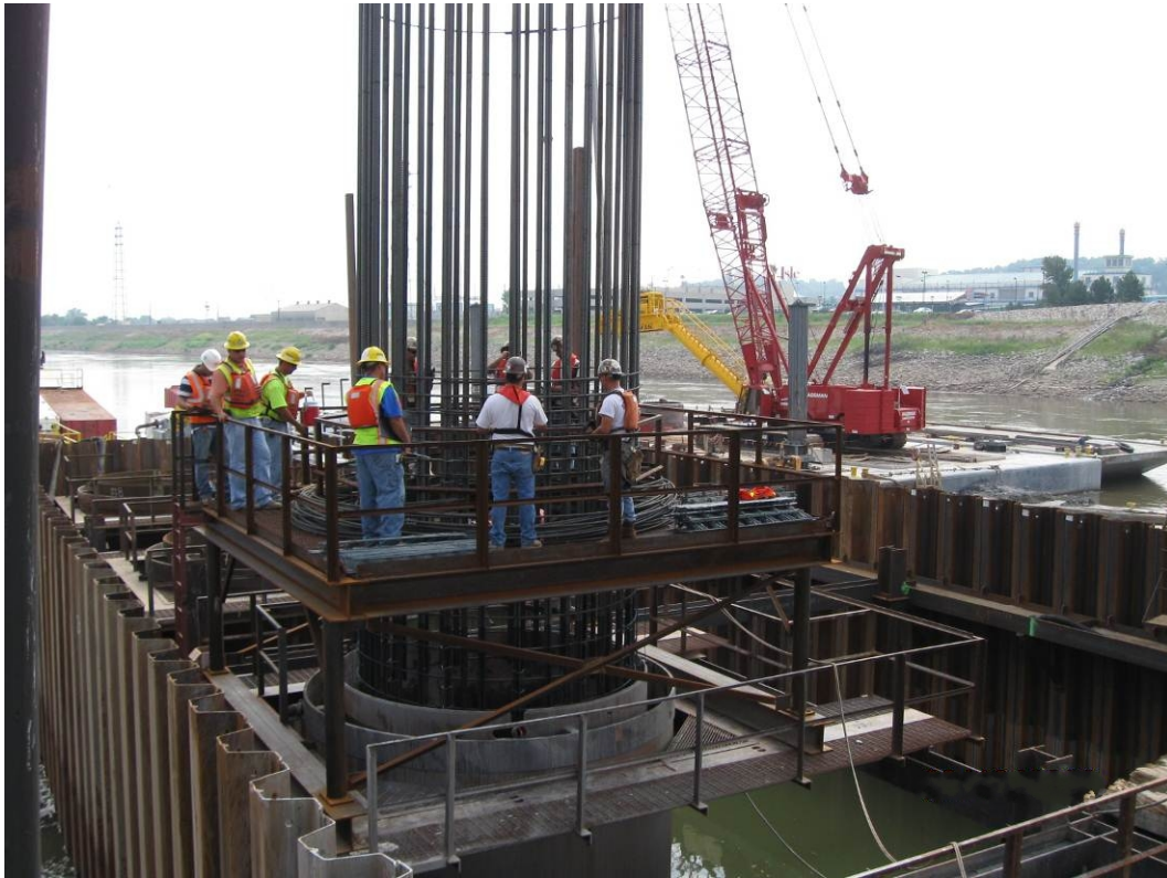
Figure 31. Tying the hoop bars to the cage as it is lowered into the drilled shaft—August 2008.
