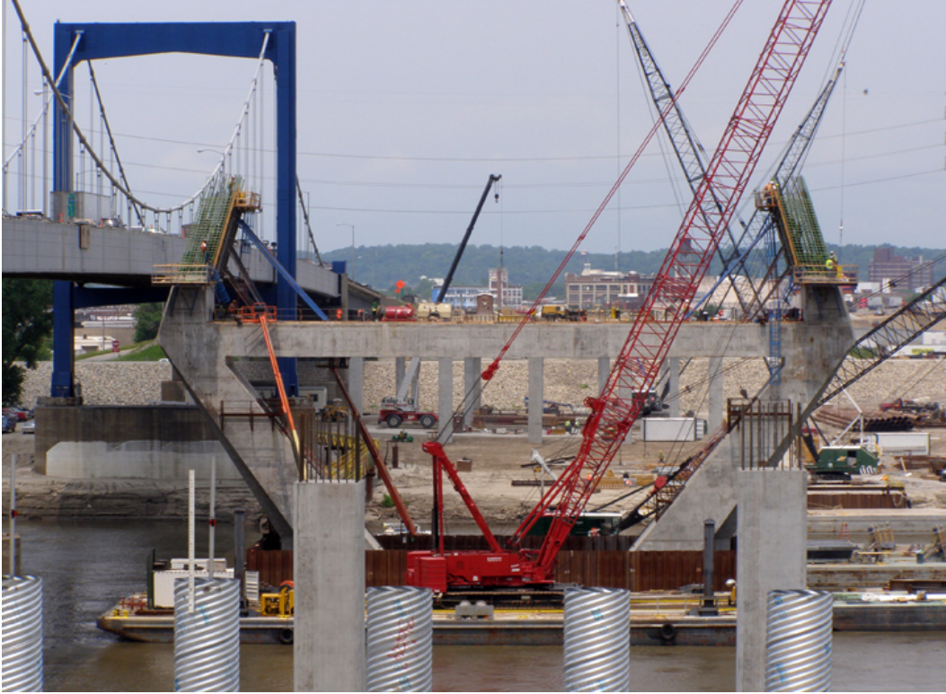
Figure 45. A third of the way to the top in constructing pylon above the roadway strut—May 2009.
