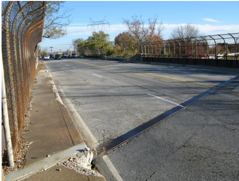
Figure 7. Sidewalk and deck deterioration.
