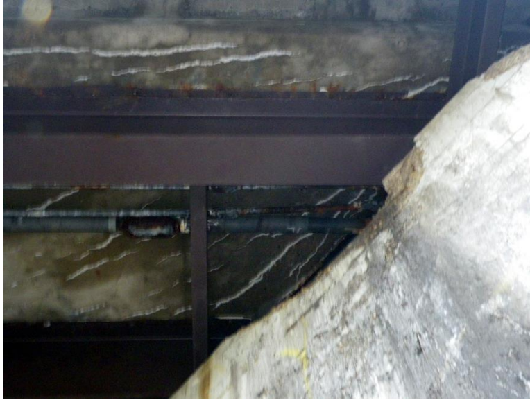
Figure 8. Cracking on underside of bridge.
