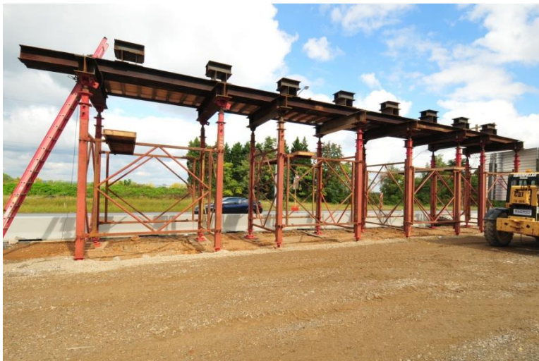
Figure 31. One of two ends of the temporary structure to support removed superstructure.
