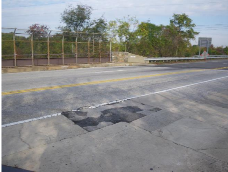
Figure 6. Extensive patches in bridge deck.
