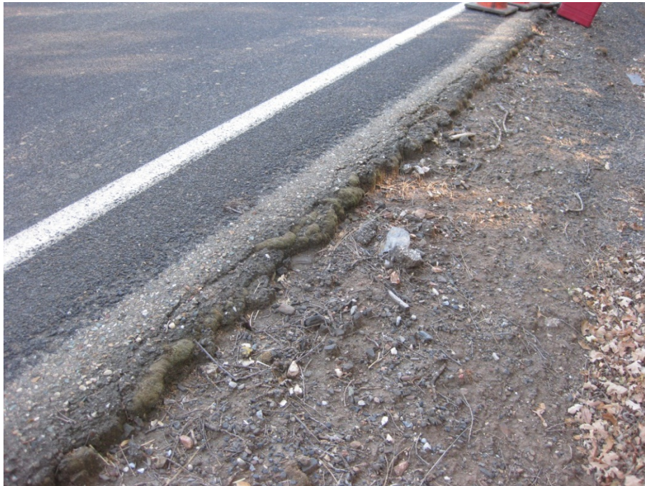
Figure 11. Condition and surface texture of existing pavement surface before milling on Mountain Ranch Road.
