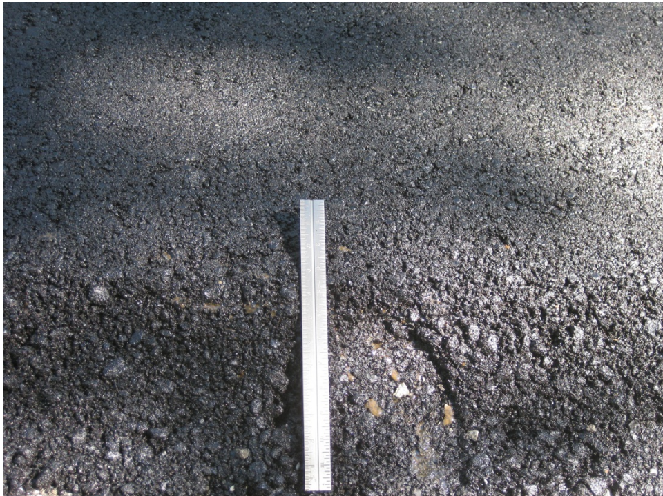
Figure 15. HMA material showing the relatively large (3/4-in nominal maximum aggregate size) aggregates for a surface mix.
