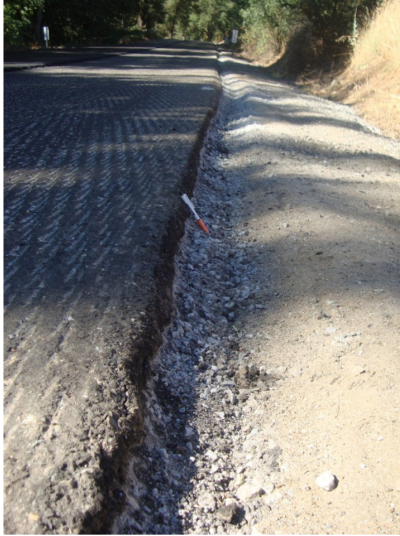
Figure 40. In many locations the shoulder material was clipped below the level of the existing pavement surface, resulting in Safety Edge heights greater than the overlay thickness.
