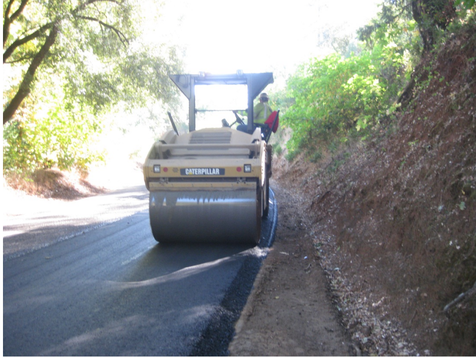
Figure 23. Finish steel-drum static roller leveling the HMA mat to the final finished surface.
