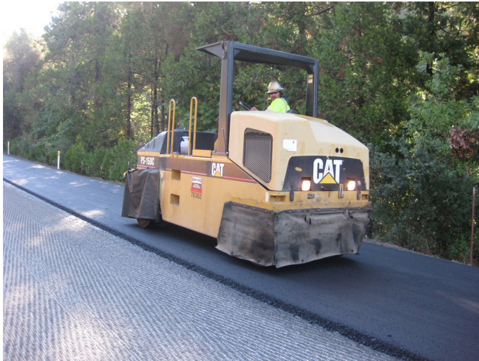
Figure 22. Intermediate pneumatic rubber tire roller was typically confined to the interior of the HMA mat (tires no closer than 6 to 9 in from the edge of the mat).
