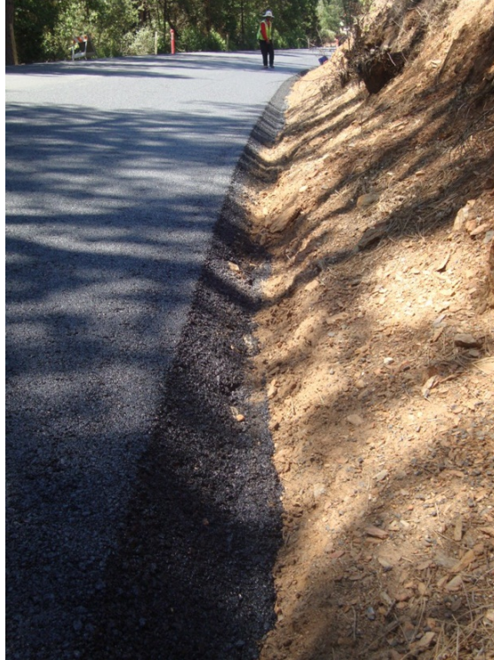
Figure 25. Small clearances between roadway edge and adjacent hillside. Even when the end gate was pulled all the way in, it was not enough to prevent loose material being pulled into the discharge area and mixing with the HMA.
