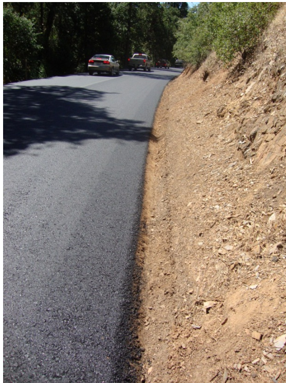
Figure 26. Worst case where hillside is very close to roadway edge and loose material is mixed with the HMA.
