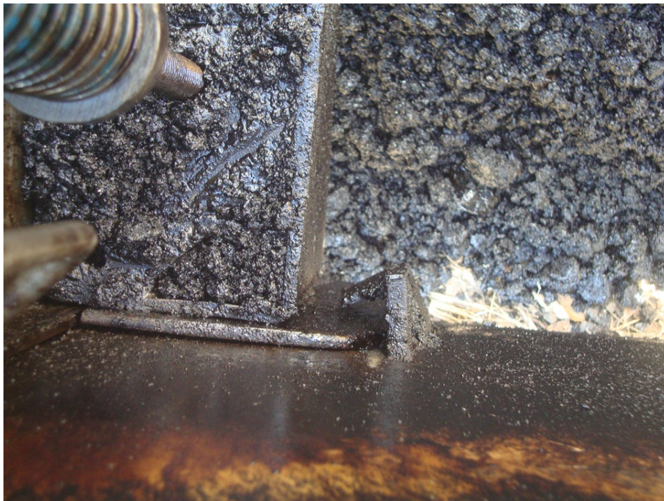
Figure 19. Contractor welded a piece of metal to the Safety Edge shoe and an angled piece to the end gate to prevent HMA from getting between the shoe and the end gate.
