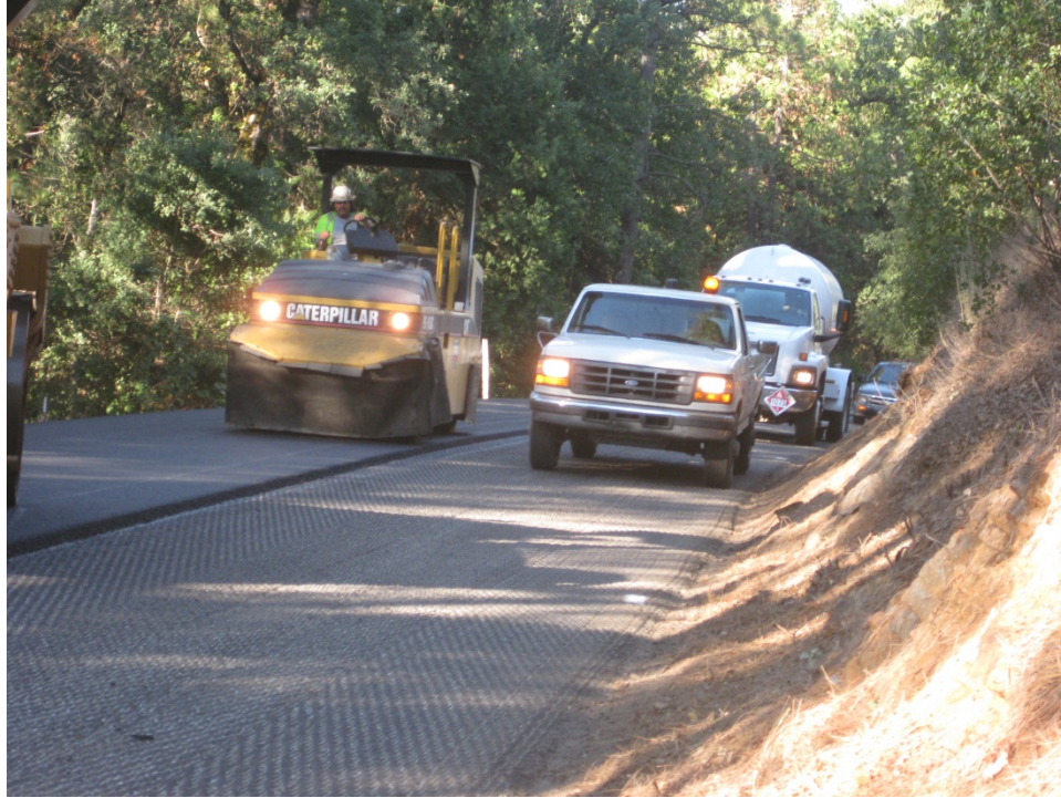
Figure 39. Pilot car leading traffic in a single file through the open traffic lane from one end of the closure to the other end.
