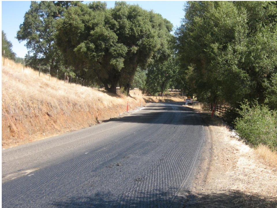
Figure 12. The existing pavement surface was milled (1 in) before HMA overlay and Safety Edge paving on Mountain Ranch Road.
