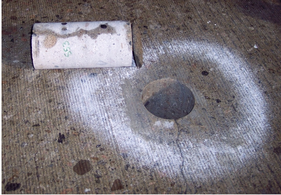
Figure 20. Cracked panel and core.
