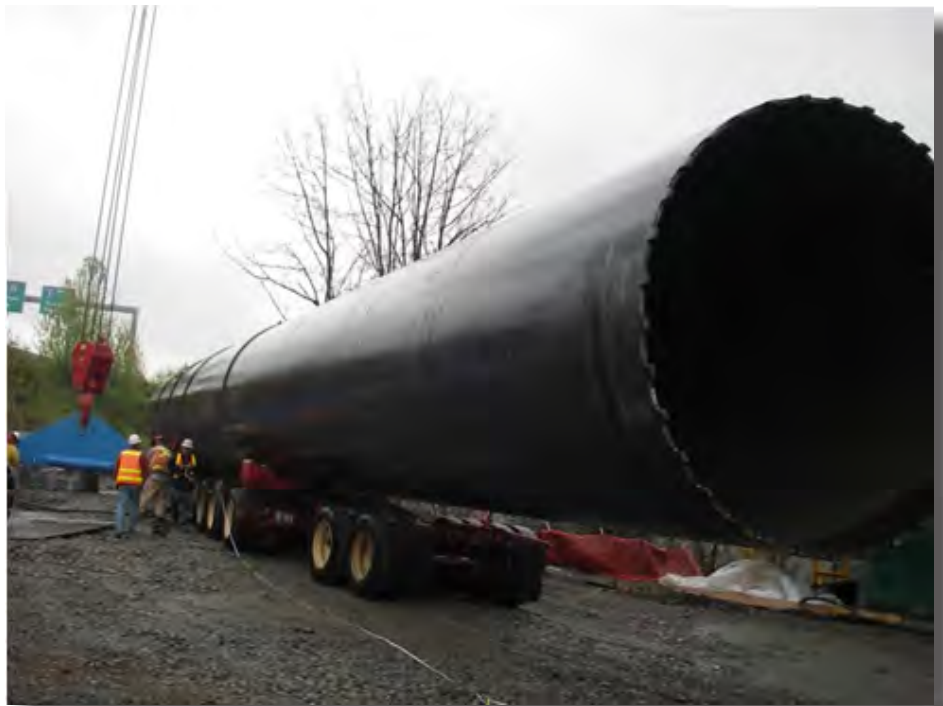
Substandard steel casing manufactured by Appleby
