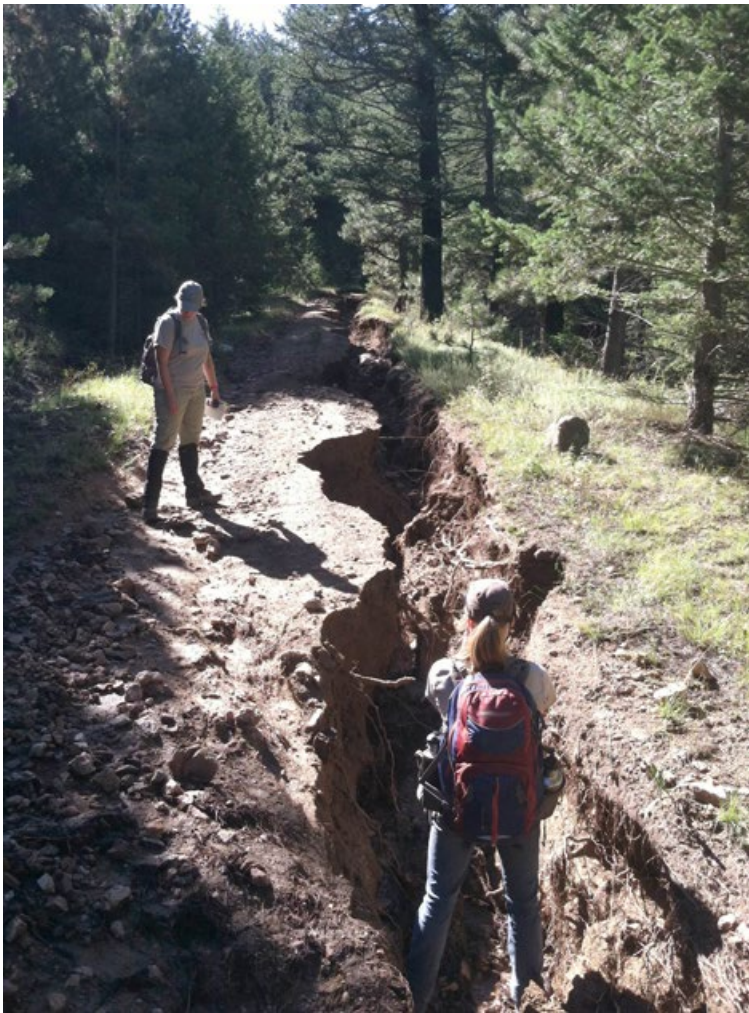
Damage from 2013 Colorado floods to Chapman Drive, now a multi-use trail, originally built by the CCC in 1935; Boulder County Parks & Open Space
