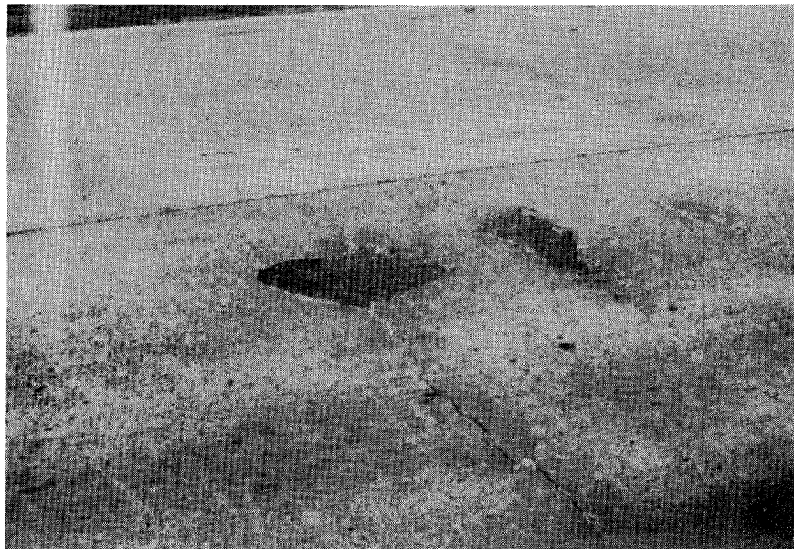
Figure 5.26. Medium Severity Localized Distress.
