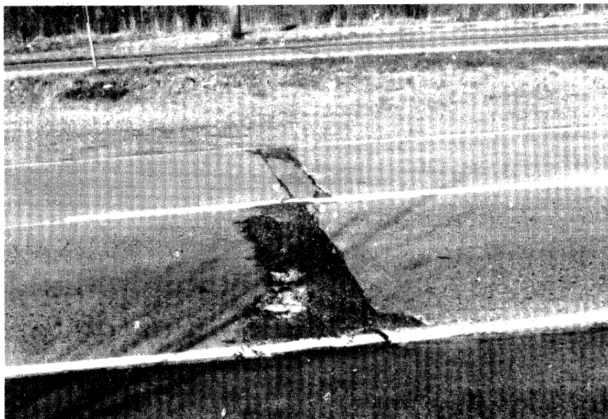
Figure 4.14. High Severity Joint Load Transfer System Associated Deterioration.
