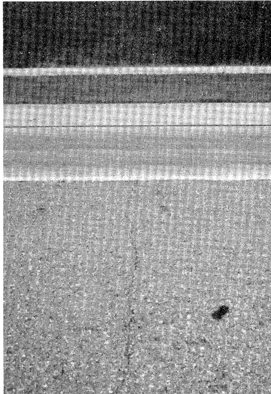
Figure 2.35. Low Severity Transverse Cracking Across Shoulder.
