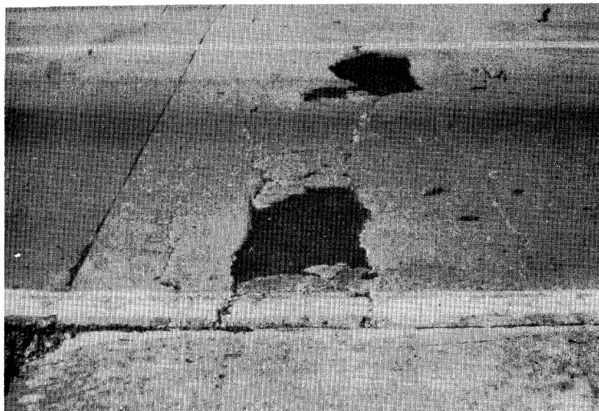
Figure 5.10. High Severity Construction Joint Deterioration.
