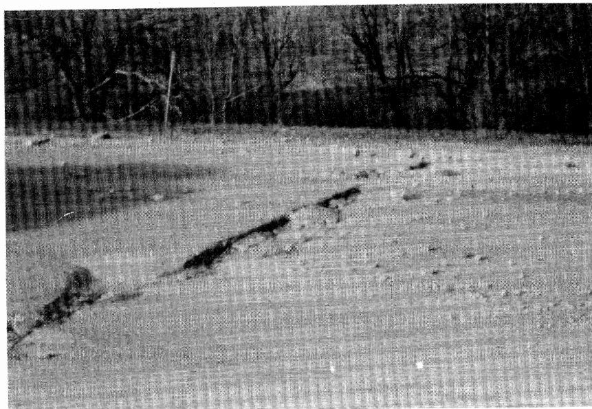
Figure 4.2. High Severity Shattering Type Blow-up.
