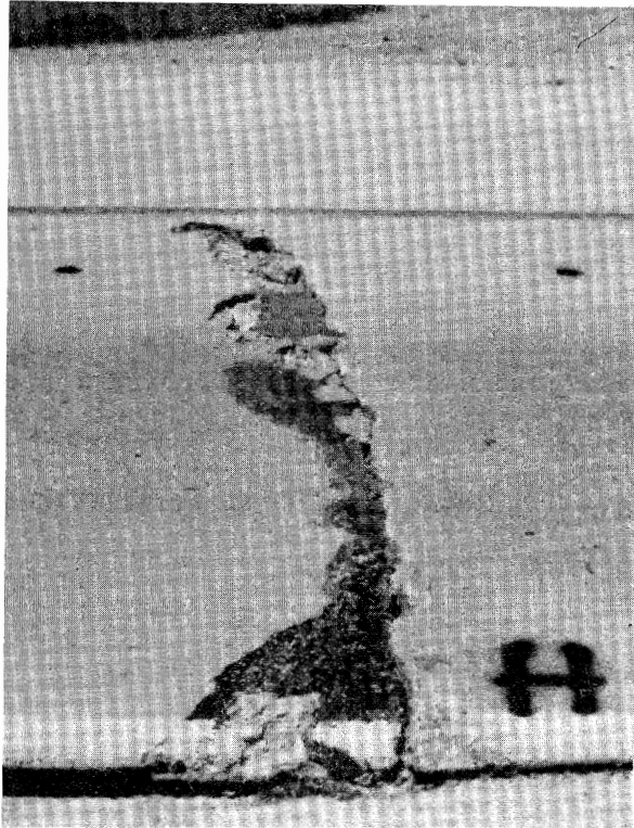
Figure 4.46. High Severity Spalling.
