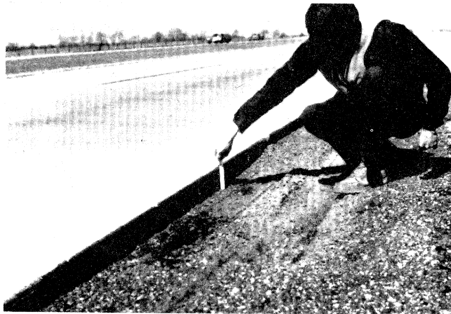
Figure 5.22. High Severity Lane/Shoulder Dropoff.
