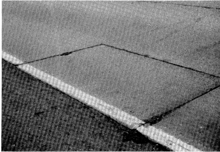
Figure 5.7. Medium Severity Concrete Patch Deterioration.
