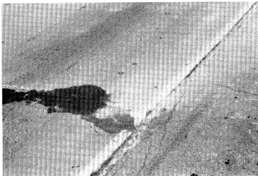
Figure 4.37. Medium Severity Pumping (pumped material like this occurs only at a few of the joints and cracks).
