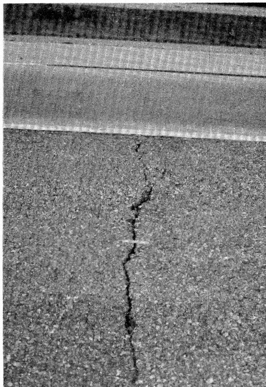
Figure 2.40. Medium Severity Transverse Cracking Across Shoulder.
