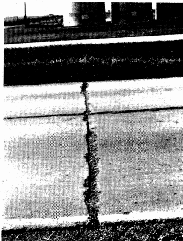
Figure 3.40. Medium Severity Spalling (Transverse Joint).
