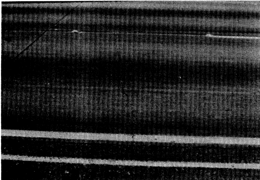
Figure 3.48. Low Severity Transverse Crack.
