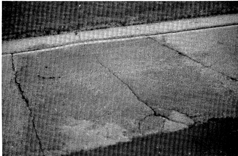
Figure 2.76. Medium Severity Swell Occurring at a Patch Due to Buckling of Concrete Slab Beneath Asphalt Surface.
