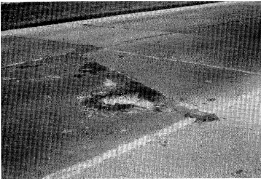
Figure 4.34. Patch Adjacent Slab Deterioration (second patch, spalling, "D" cracking and temporary patching).
