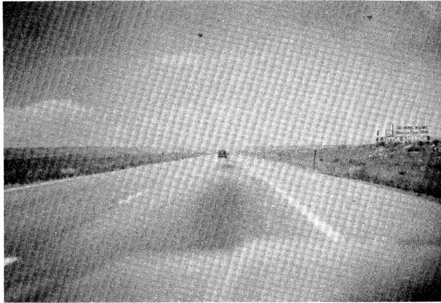
Figure 2.22. Low Severity Depression (identified by oil droppings on pavement surface).
