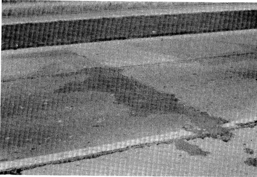
Figure 4.33. Patch Adjacent Slab Deterioration ("D" cracking & temporary patching).
