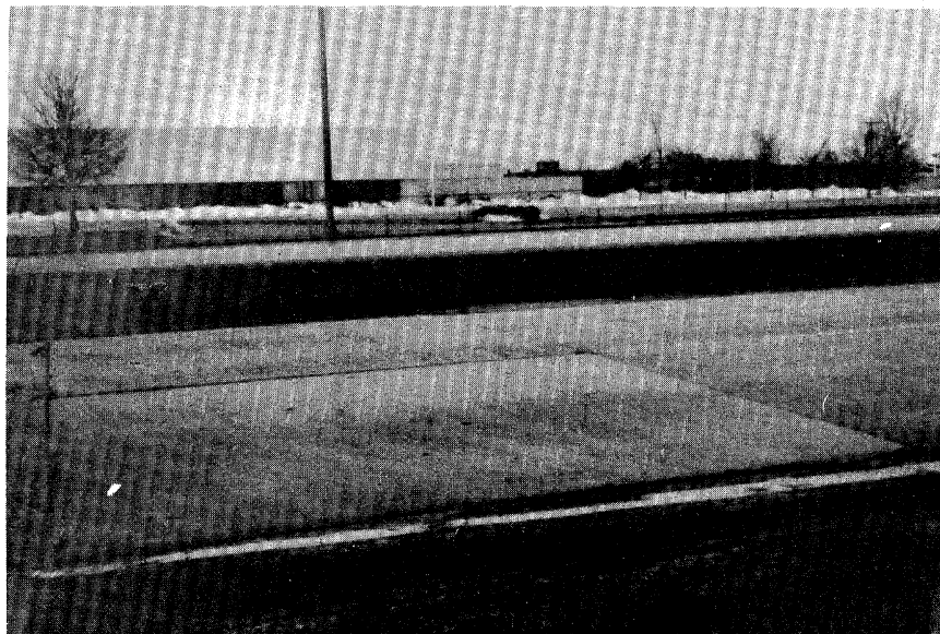
Figure 3.22. Low Severity PCC Patch Deterioration.
