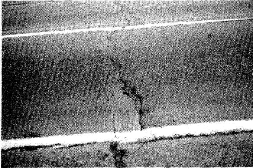
Figure 2.41. High Severity Transverse Cracking.
