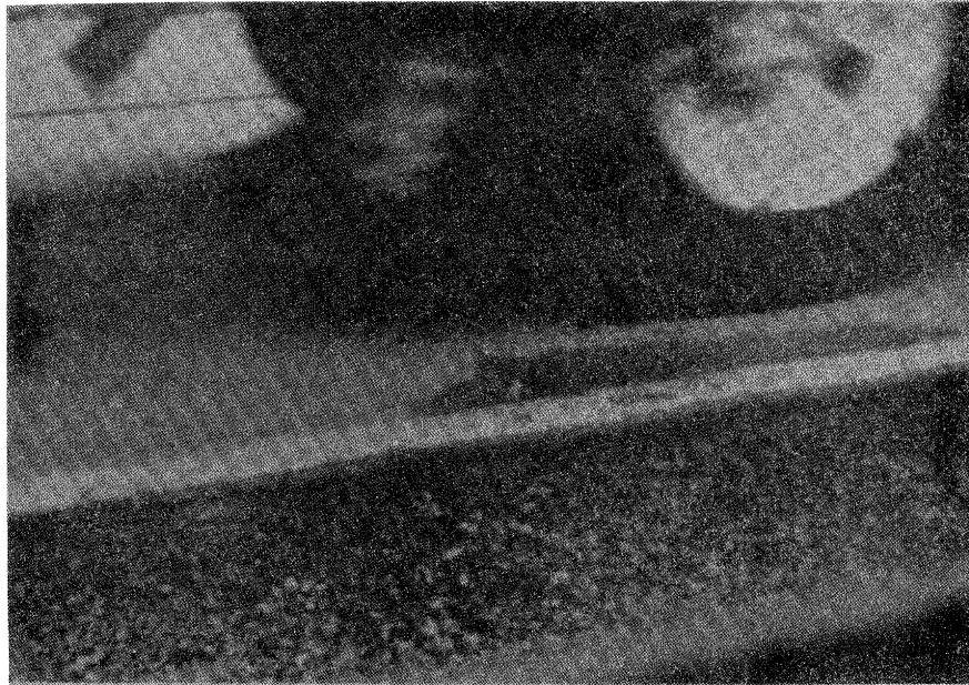
Figure 5.38. Low Severity Pumping (water ejected out of transverse crack under truck wheel).
