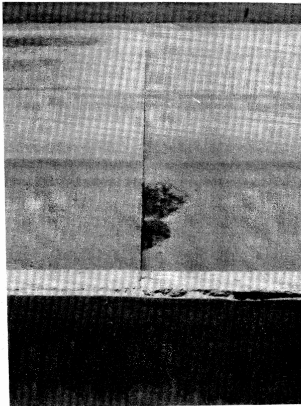
Figure 3.43. High Severity Spalling (Transverse Joint) (safety hazard).
