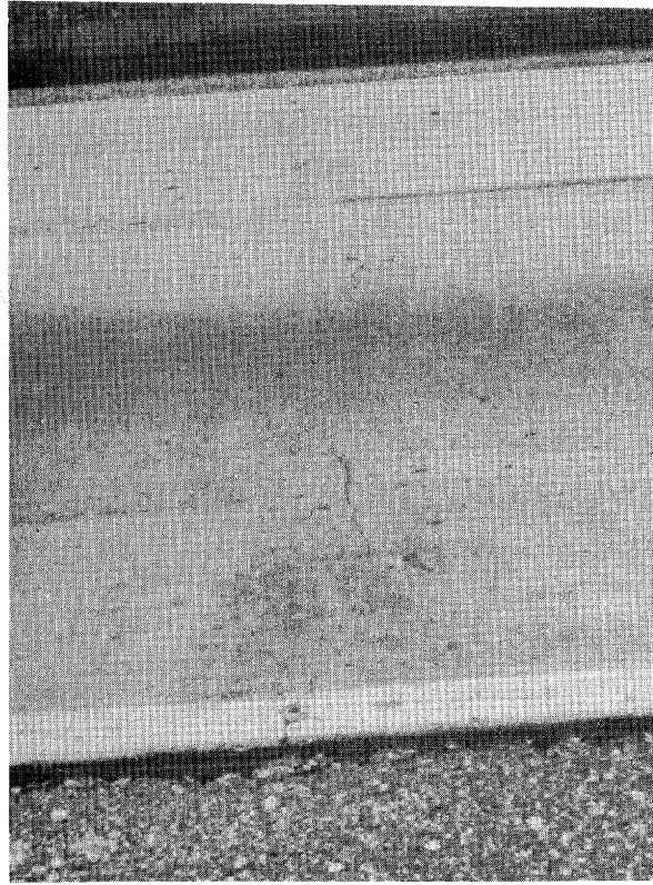
Figure 5.13. Low Severity "D" Cracking.
