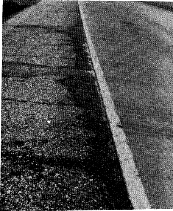
Figure 5.40. Low Severity Water Bleeding.
