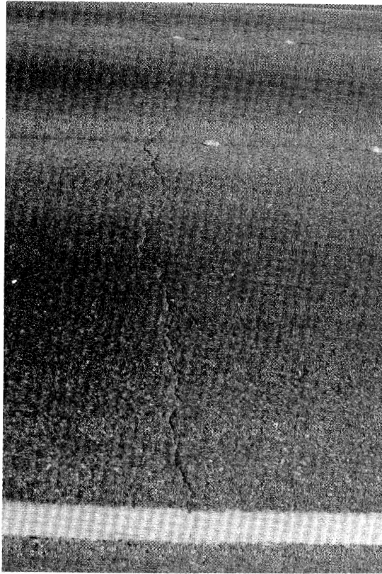
Figure 2.24. Low Severity Joint Reflection Cracking from Transverse Joint in PCC Slab.
