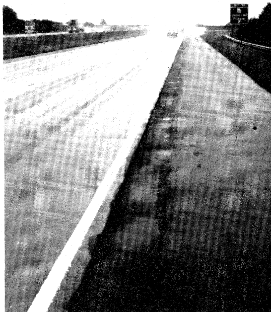
Figure 2.47. Low Severity Patch Along Shoulder Joint.
