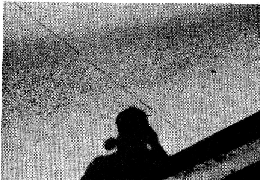
Figure 3.19. Low Severity Longitudinal Crack.
