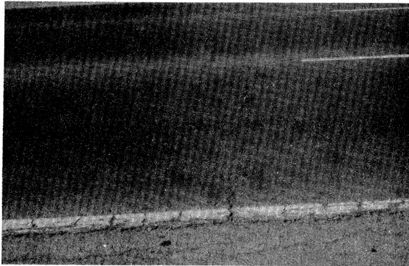
Figure 2.25. Low Severity Joint Reflection Cracking from Transverse Joint in PCC Slab.
