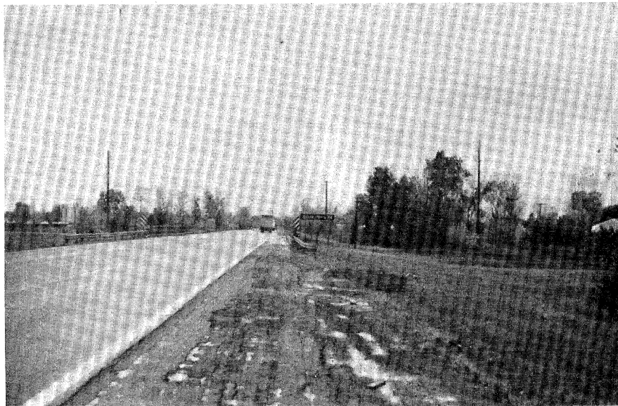
Figure 2.69. High Severity Raveling and Weathering.
