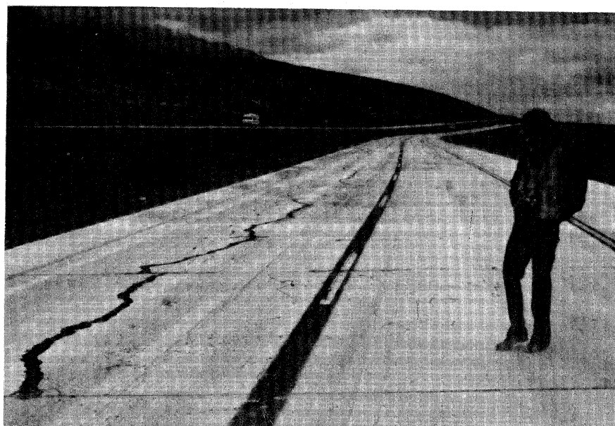
Figure 3.46. Swell Due to Frost Heave.
