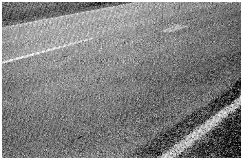
Figure 2.2. Low Severity Alligator Cracking (fine longitudinal cracks in wheel path ).
