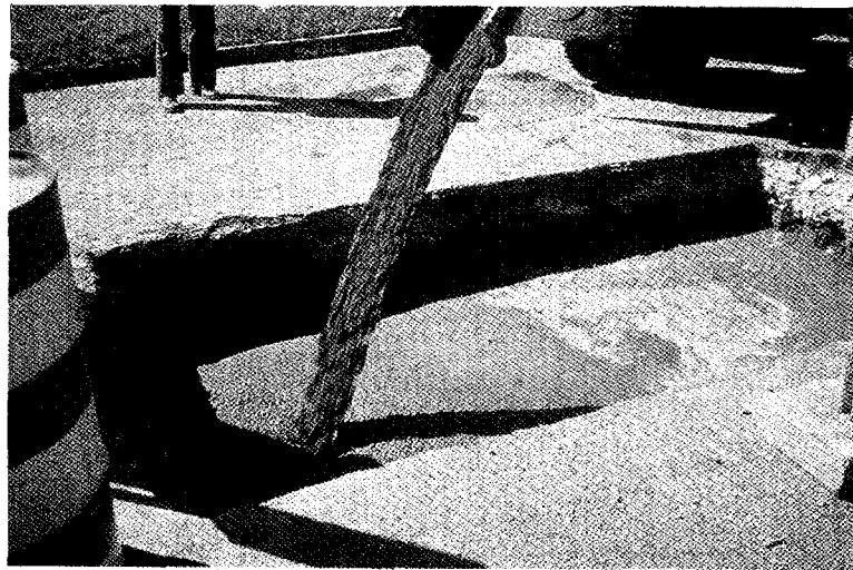
Figure 14. Flowable fill used as backfill material for a utility trench allows rapid return of traffic to the roadway.
