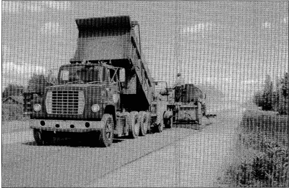
Michigan DOT relies on a wide variety of preventive maintenance treatments to extend the life of its pavements. Here, a chip seal is applied.
