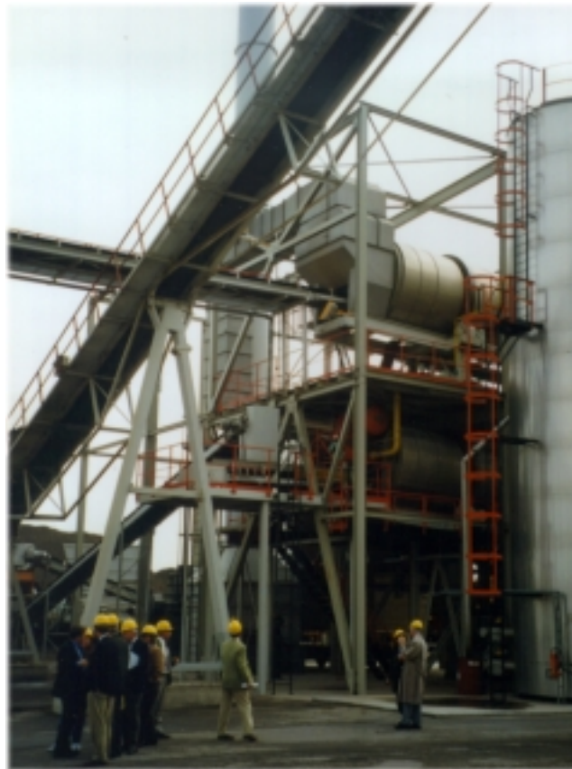
Figure 24. The double drums allow for high introduction of RAP at the Swiss-designed Ammann double drum hot recycling asphalt plant in the Netherlands. RAP is heated in the lower drum and virgin aggregates are heated in the upper drum.
