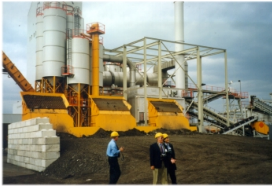
Figure 23. RAP is sorted before introduction into the lower drum at the Swiss-designed Ammann double drum asphalt plant in the Netherlands.
