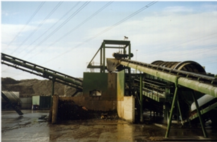
Figure 26. The WTE bottom ash crushing and sieving process at the Jean LeFebvre MSW bottom ash recycling plant in France.
