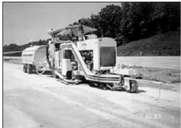
Figure 8. Diamond grinding convoy including grinder, vacuum to pick-up slurry residue and water tank for cooling the blades.
