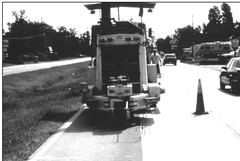
Figure 6. Diamond grinding equipment making multiple passes to grind a full lane width.
