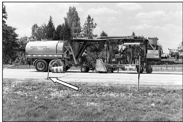
Figure 9. Slurry residue of diamond grinding being discharged to the embankment in a rural area.
