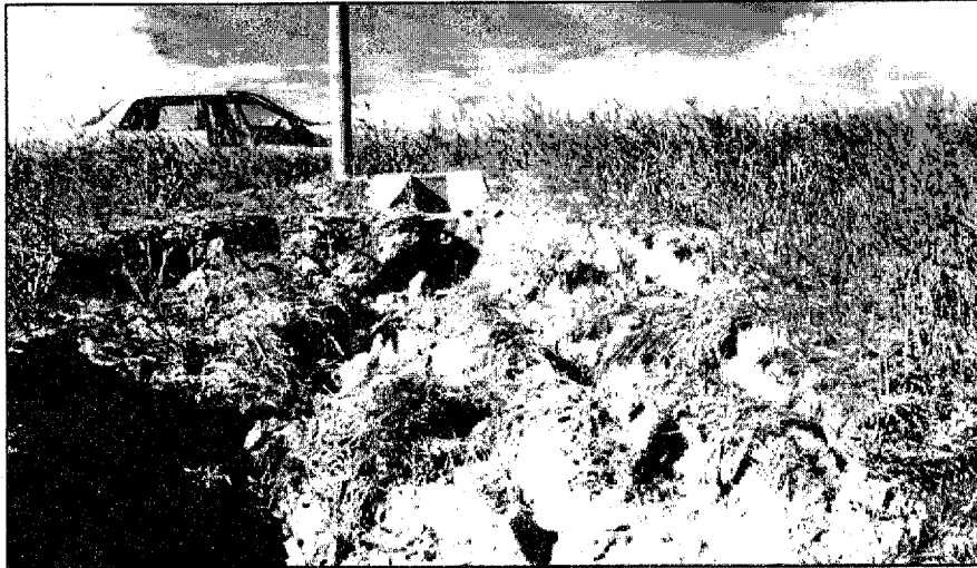
Photo No. 10 Outlet Erosion
