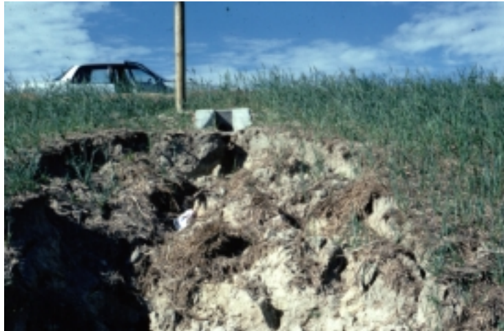
Photo No. 7 Excessive Erosion at the Outlet Pipe
