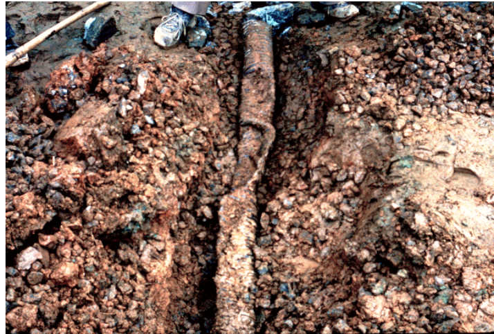
Photo No. 9 Crushed Edgedrain Pipe
