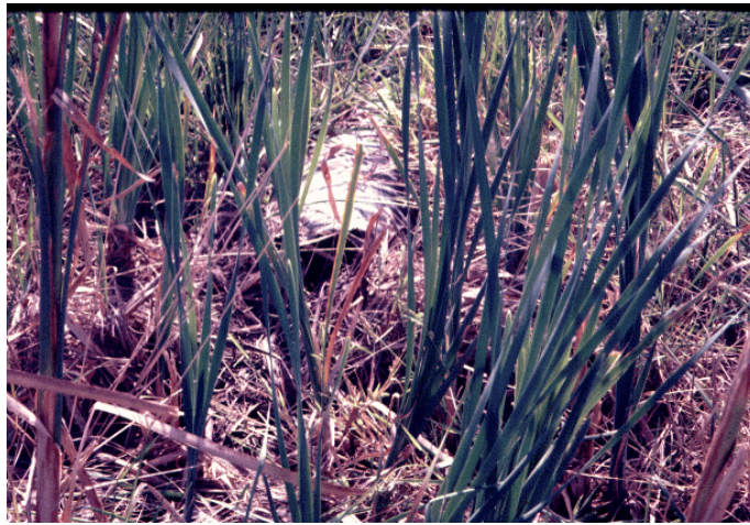
Photo No. 5 Hidden Outlet Pipe
