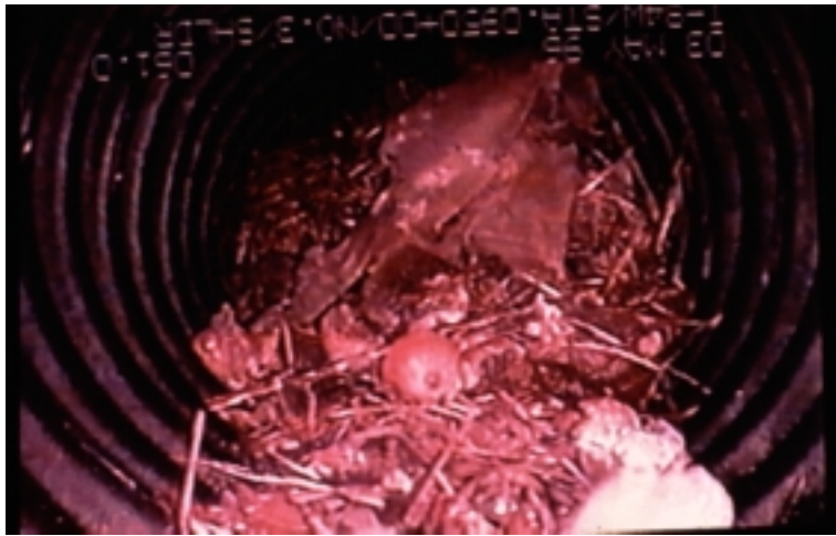
Photo No. 2 Rodent's Nest
