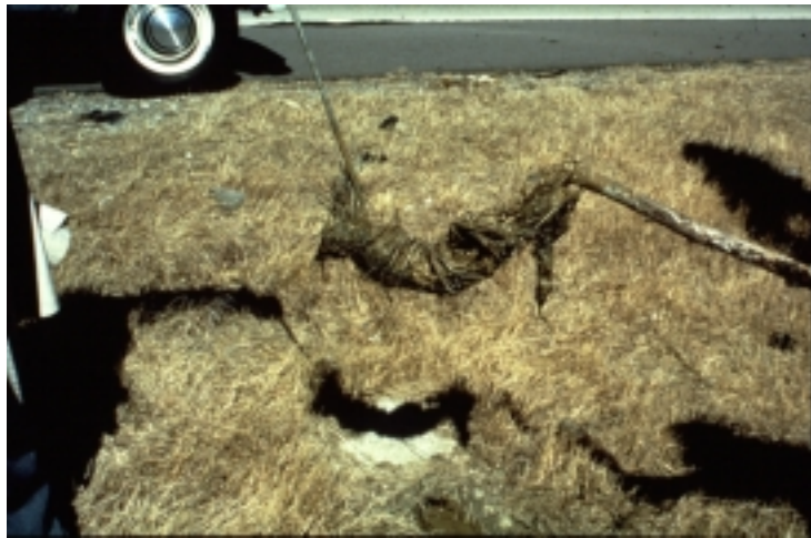
Photo No. 1 Vegetative Material Removed from an Edgedrain System
