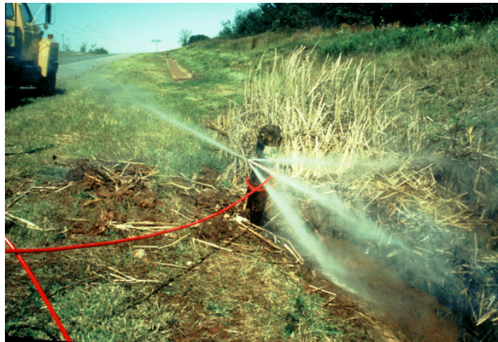
Photo No. 11 Pipe Flushing Unit
