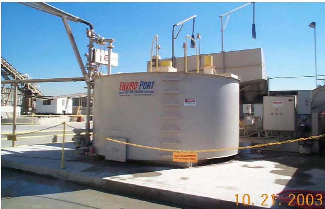
Figure 24. Reclaim System. Red-I -Mix Concrete Inc. Facility Visit. Irwindale, CA
