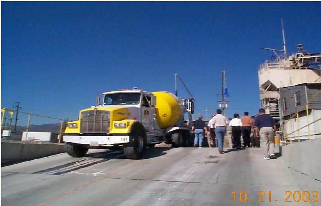
Figure 21. Truck Dumping Plastic Portland Cement Concrete (PPCC) to the Reclaim System. Red-I-Mix Concrete Inc. Facility Visit. Irwindale, CA
