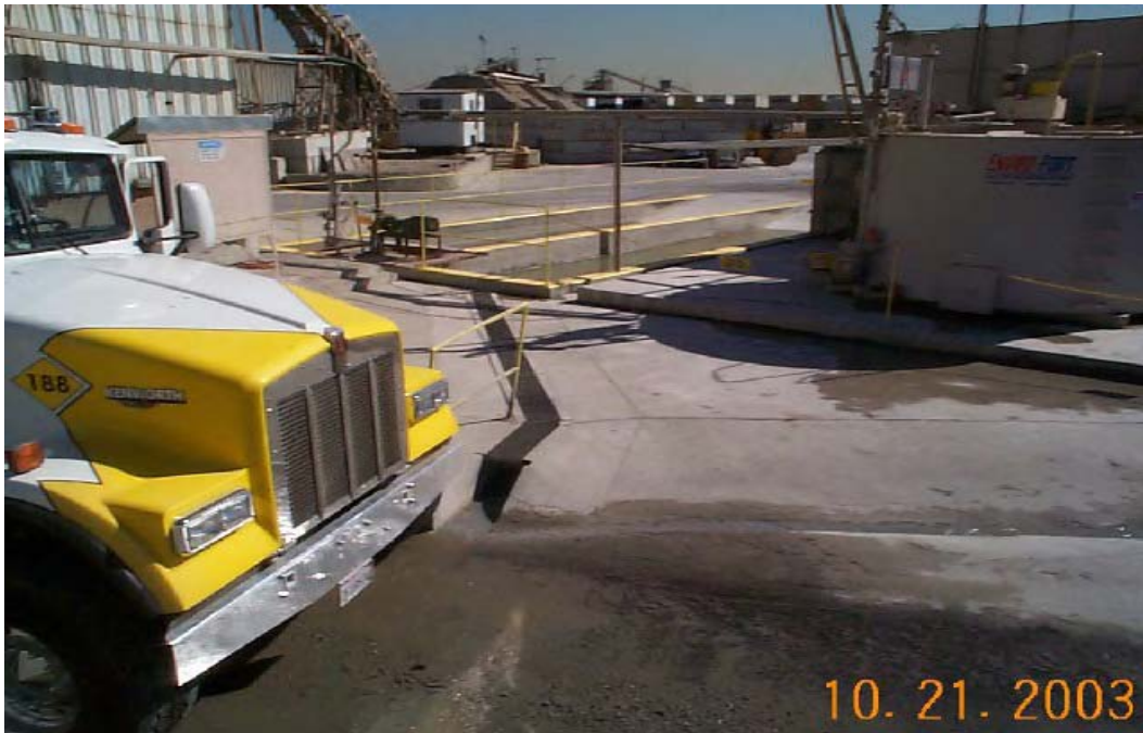
Figure 29. Washout Water Drain System. Red-I -Mix Concrete Inc. Facility Visit. Irwindale, CA.
