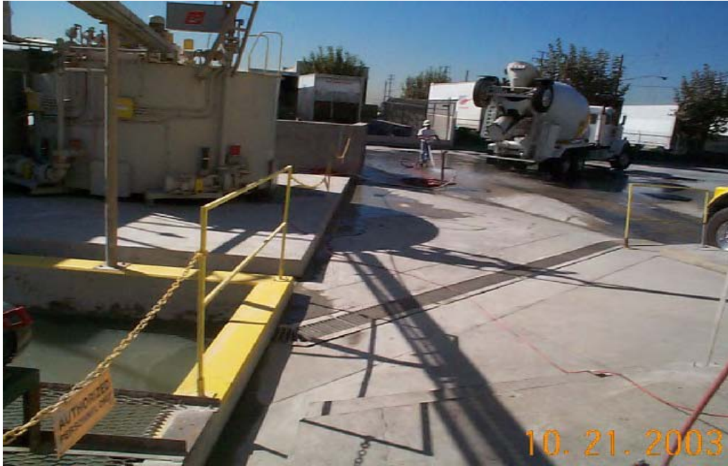
Figure 28. Washout Water Drain System. Red-I -Mix Concrete Inc. Facility Visit. Irwindale, CA.
