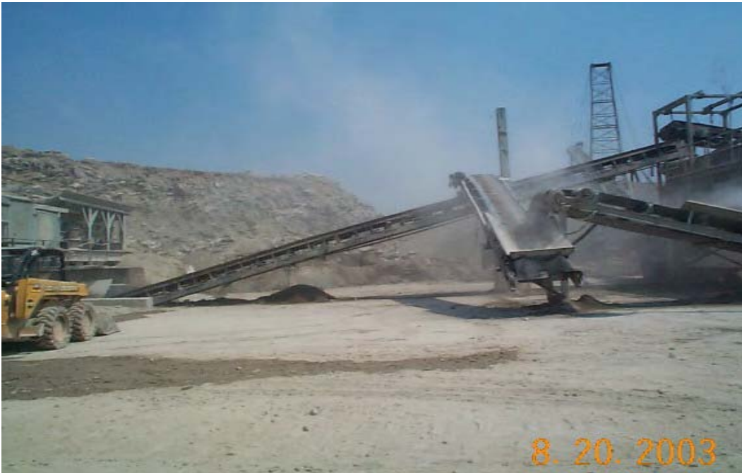
Figure 10. Vibrating-feeder transporting RCA from Primary Crusher to sorting screen. Iafrate Crushing Plant Visit. Taylor, MI
