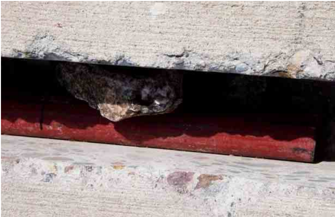
Figure 8. Dowel bar wedged in a slot of the test slab at the MnRoad facility.
