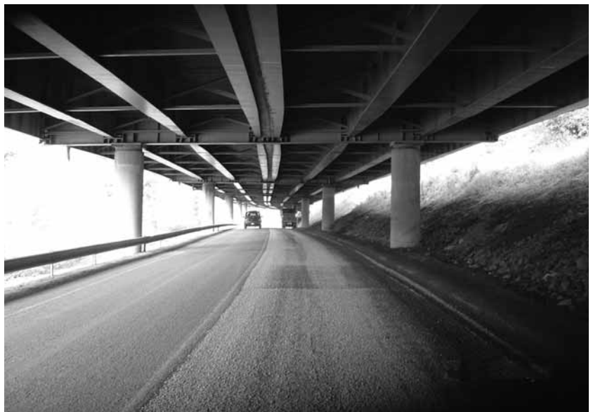
With each application, the county hopes to extend a road's service life another 5 to 6 years.
