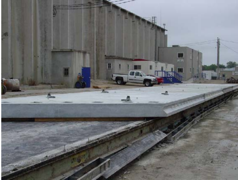
Figure 22. Photo. Trial assembly of precast panels at the fabrication plant (photo by Iowa DOT, reprinted by permission).
