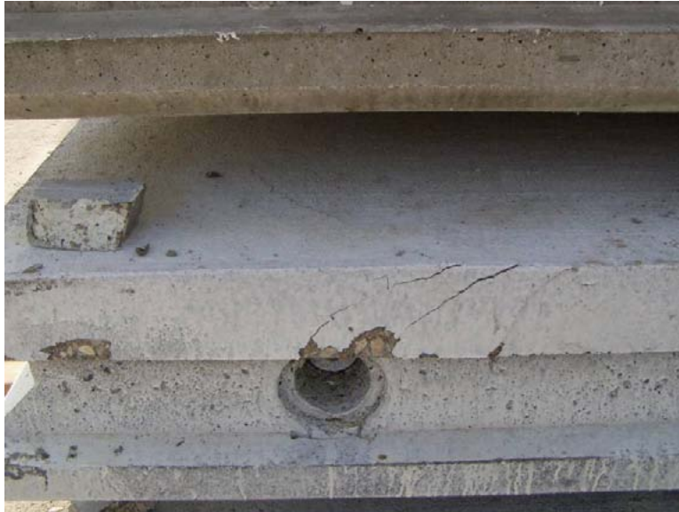
Figure 23. Photo. Damaged panel corner after trial assembly.
