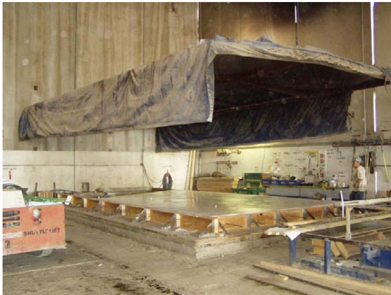
Figure 20. Photo. Curing tent being lowered to cover a precast panel after casting.
