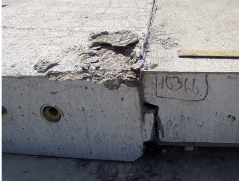
Figure 41. Photo. Minor joint spall that occurred during panel installation.
