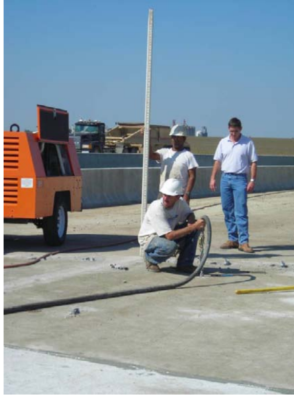
Figure 35. Photo. Rod and level were used to check for slab lifting during the underslab grouting operation. (photo by Iowa State University, reprinted by permission).
