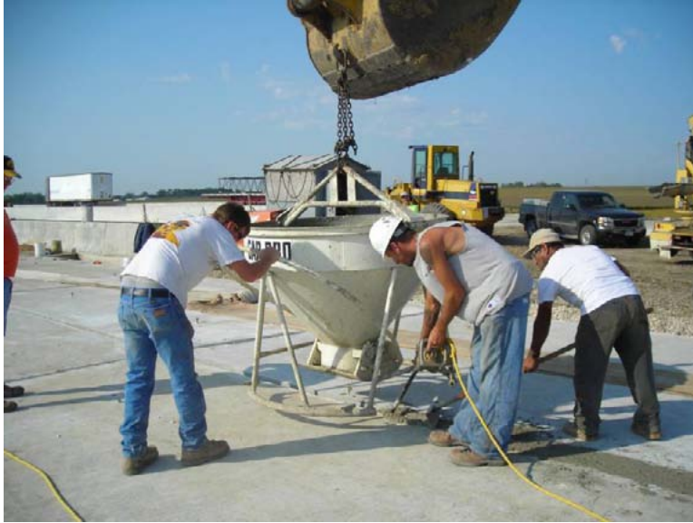
Figure 36. Photo. Filling of the longitudinal joint (photo by Iowa State University, reprinted by permission).
