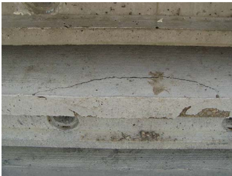
Figure 24. Photo. Damaged keyway after trial assembly.
