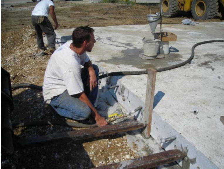
Figure 34. Photo. Grouting of the post-tensioning tendons (photo by Iowa State University, reprinted by permission).
