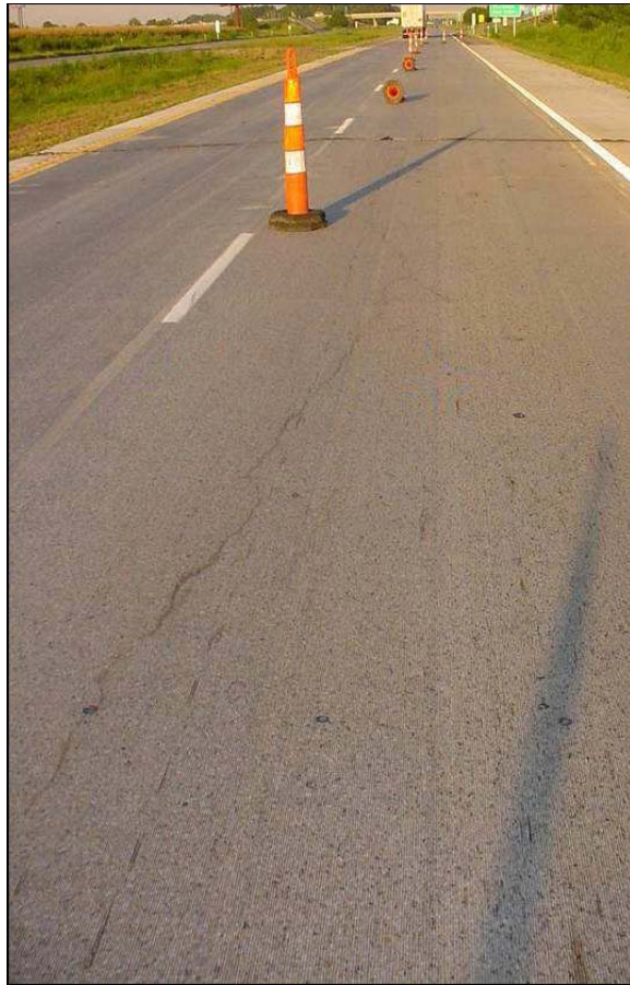
Figure 52. Photo. Longitudinal crack near the pavement centerline extending away from one of the instrumentation blockouts. (18)
