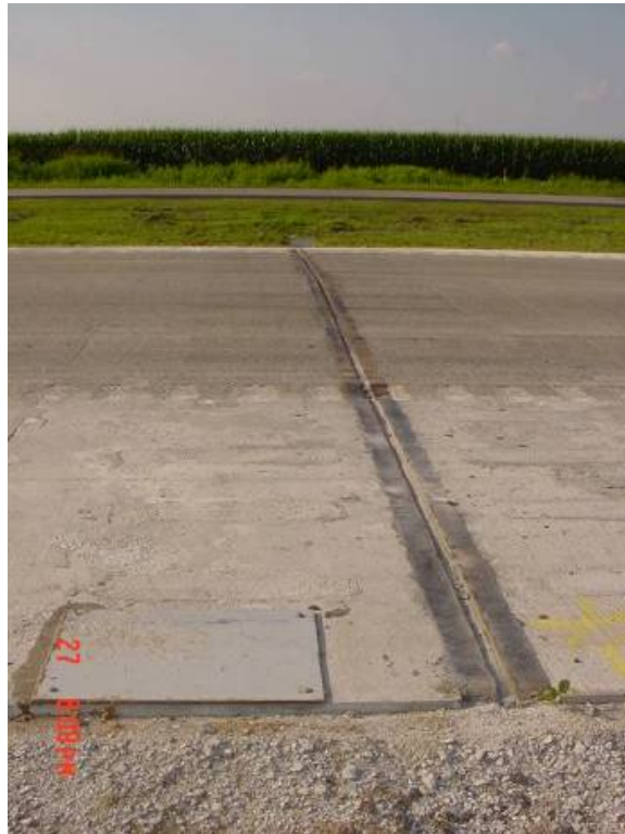
Figure 42. Photo. Good performing header expansion joints. (18)
