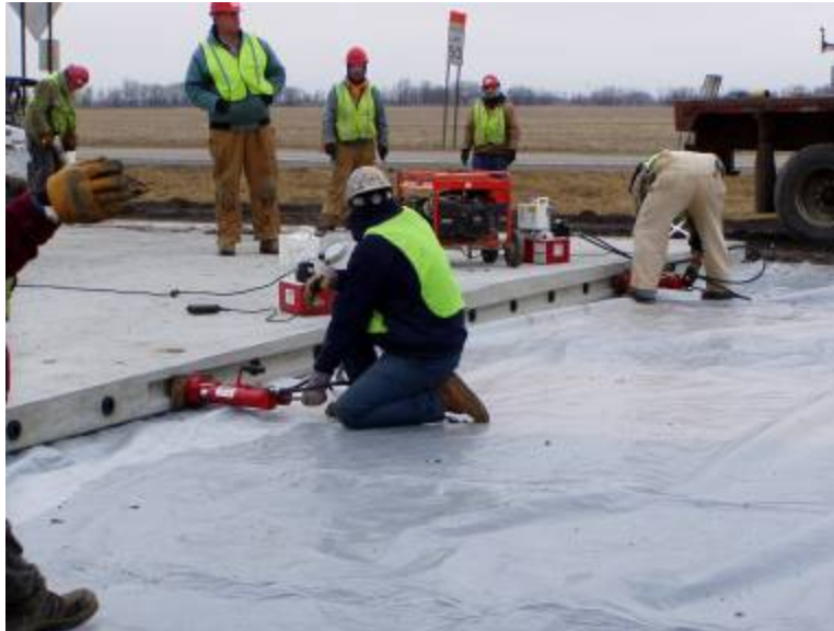
Figure 37. Photo. Temporary post-tensioning was used to close the joints between panels as much as possible during panel installation.
