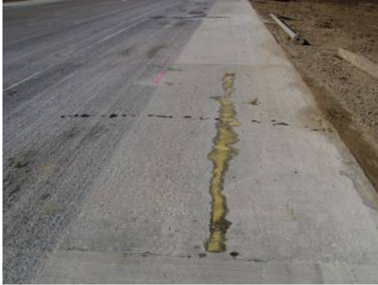
Figure 29. Hairline transverse crack in the shoulder after epoxy sealing (photo taken after panel was installed on site).
