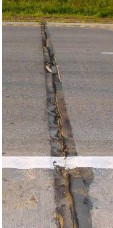
Figure 43. Photo. Deterioration of header material for expansion joint No. 4. (18)
