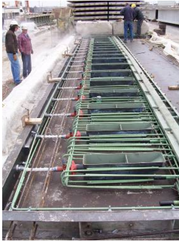
Figure 14. Photo. Joint panel prior to concrete placement, showing post-tensioning pockets, anchors, stirrups and dowels.
