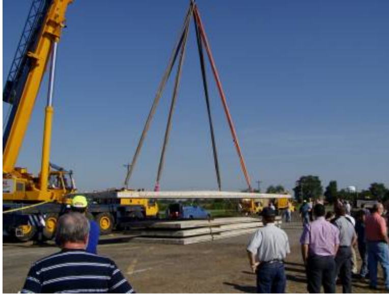
Figure 50. Photo. The workshop participants were able to see a live demonstration of the panel installation process at a MoDOT maintenance yard in Sikeston.
