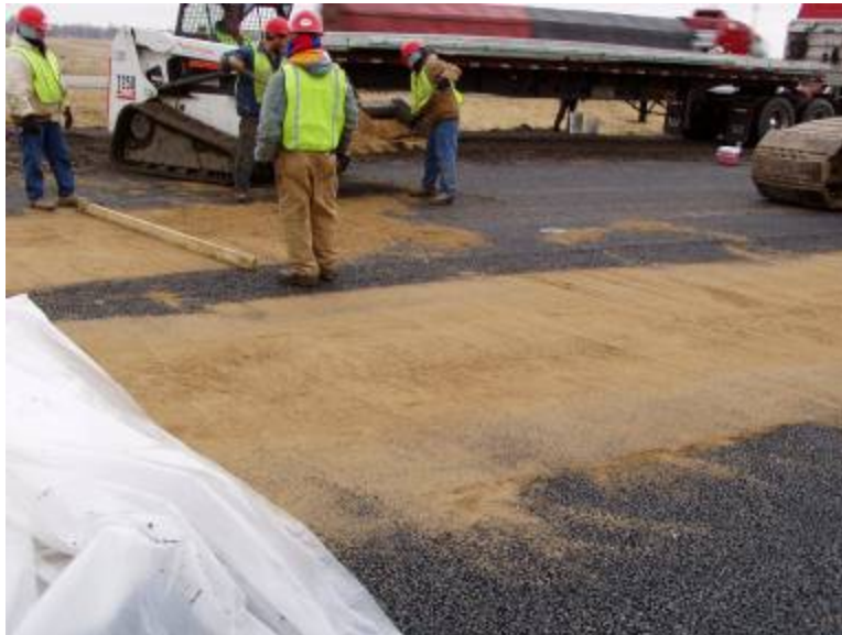
Figure 34. Photo. Sand was used to fill the ruts in the permeable asphalt treated base.
