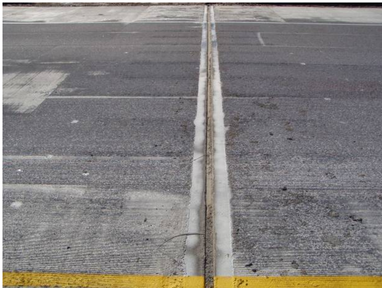
Figure 54. Photo. Typical condition of expansion joints 1,2,3, and 5 in service.
