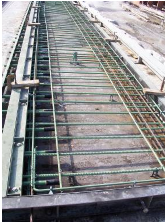
Figure 19. Photo. Reinforcement for the non-post-tensioned half of a joint panel prior to casting.
