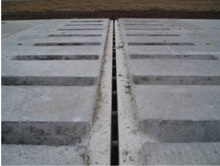
Figure 40. Photo. Expansion joint after being pulled open during the post-tensioning operation. (photo from MoDOT).
