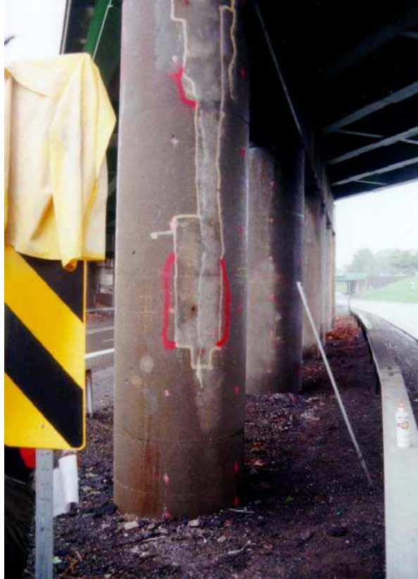
Figure 43. Photo. Second view of a completely delaminated patch (marked in yellow) on a column of the Campus Loop Bridge in Albany, NY.
