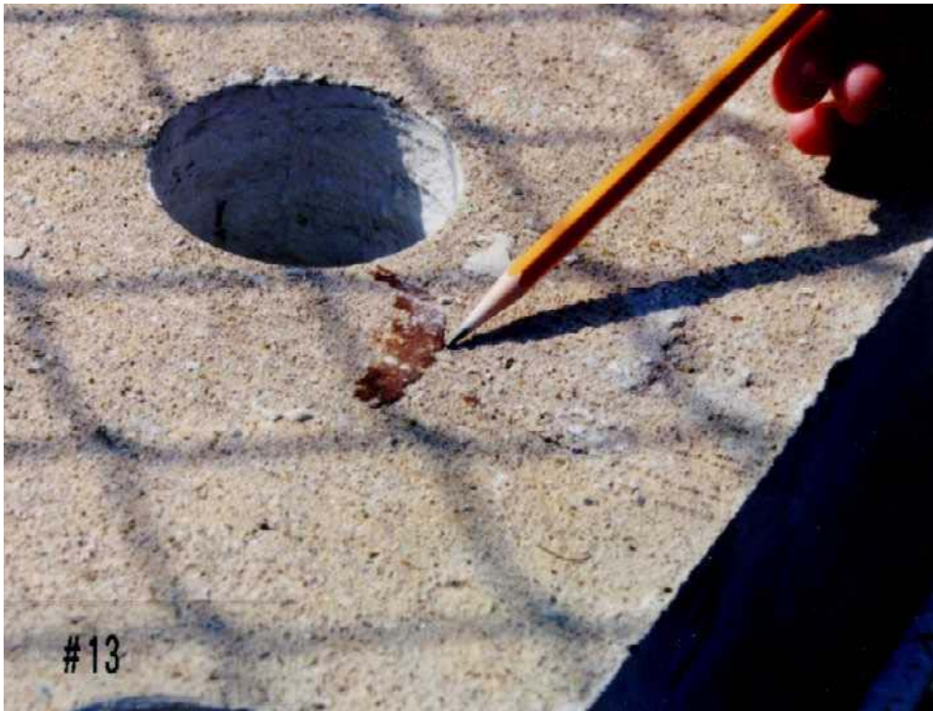
Figure 14. Photo. Rust staining on the top surface of slabs 3 and 4.
