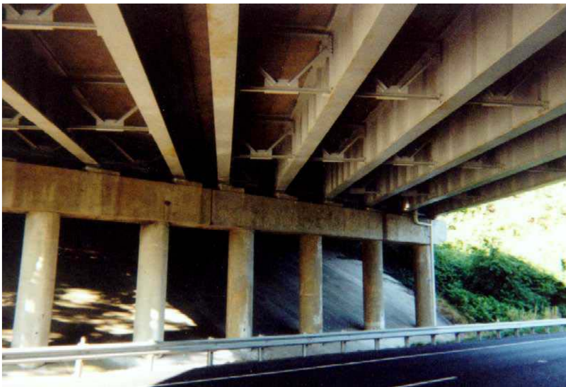
Figure 53. Photo. Soffit, bents, and columns of Route 631 over I-64 bridge in Charlottesville, VA.
