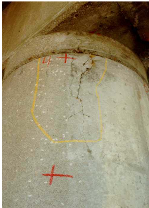
Figure 40. Photo. Cracks and rust staining in a nonpatched area of a column of the Campus Loop Bridge in Albany, NY, during the second visit in 1996.
