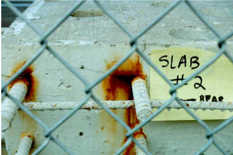
Figure 6. Photo. Cracks and corrosion products on the rear side of slab 2 in August 1998.
