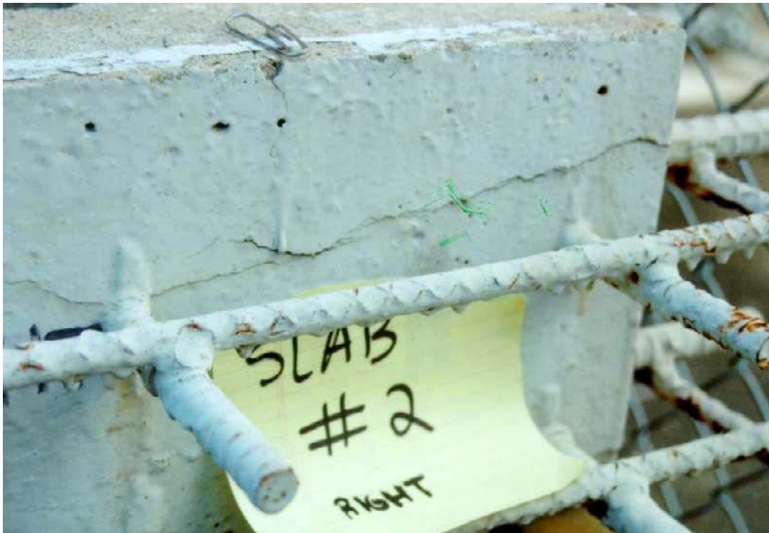
Figure 9. Photo. Crack on the right side of slab 2.
