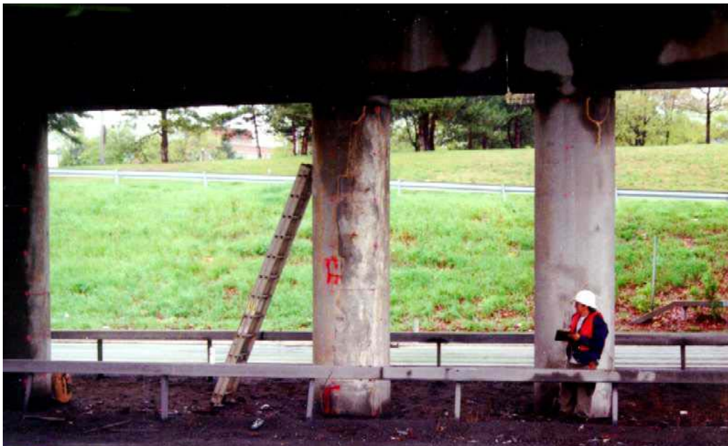
Figure 41. Photo. Water flowing down the pier caps and columns through leaking joints.
