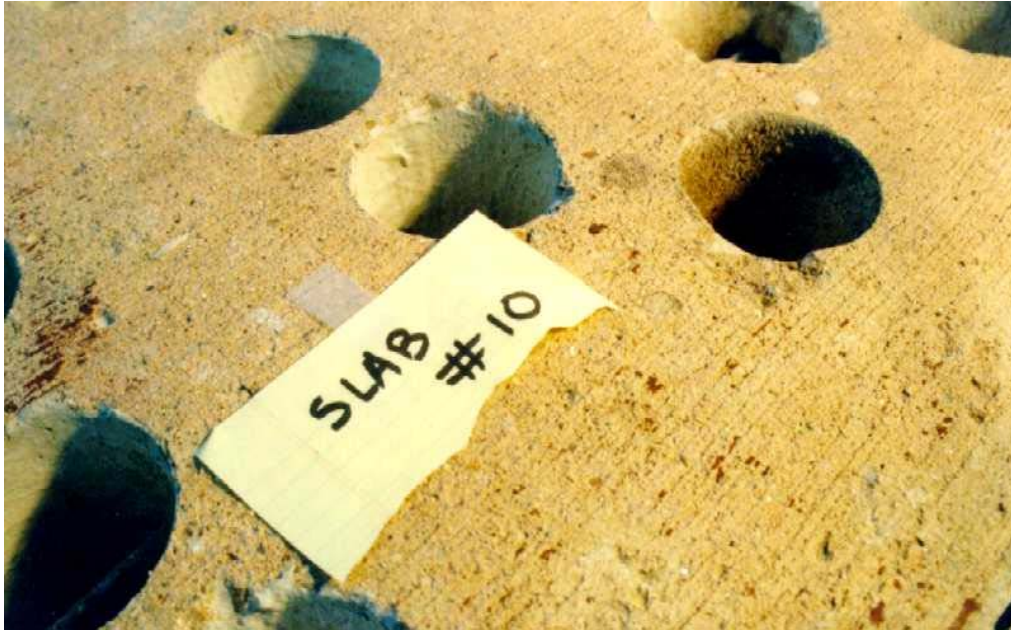
Figure 18. Photo. Rust stains on the top surface of slab 10.
