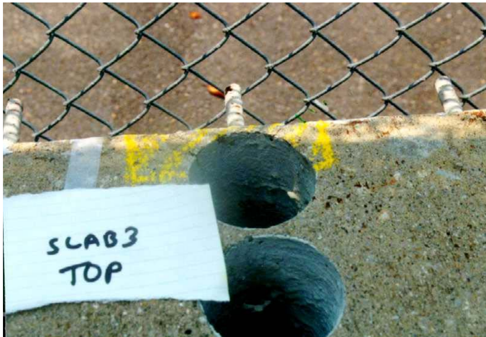
Figure 13. Photo. Delamination (marked in yellow) found on the top surface of slab 3.
