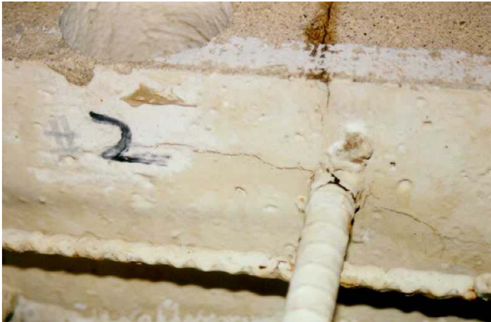
Figure 5. Photo. Termination of the top crack and other cracks on the front side of slab 2 in August 1994.
