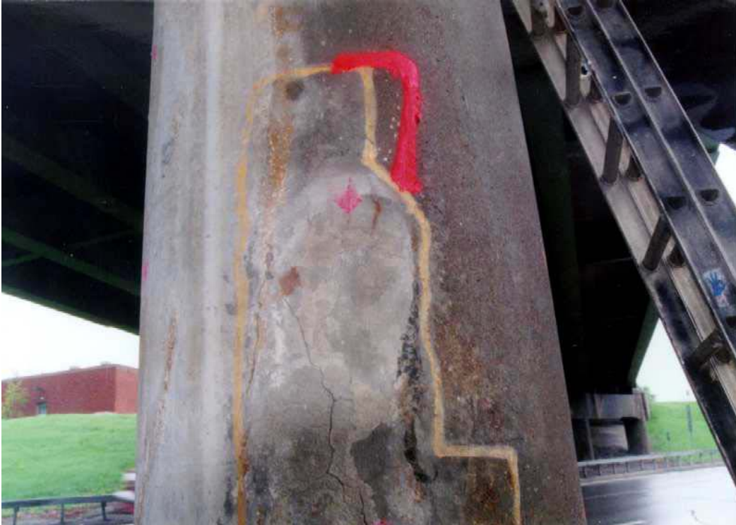
Figure 42. Photo. First view of a completely delaminated patch (marked in yellow) on a column of the Campus Loop Bridge in Albany, NY.
