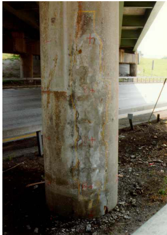
Figure 38. Photo. First view of cracks and rust staining in patched and nonpatched areas of the columns of the Campus Loop Bridge in Albany, NY, during the second visit in 1996.
