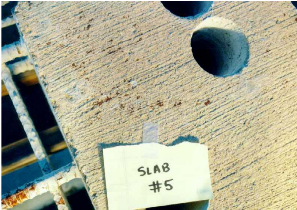
Figure 16. Photo. Rust stains on the top surface of slab 5.
