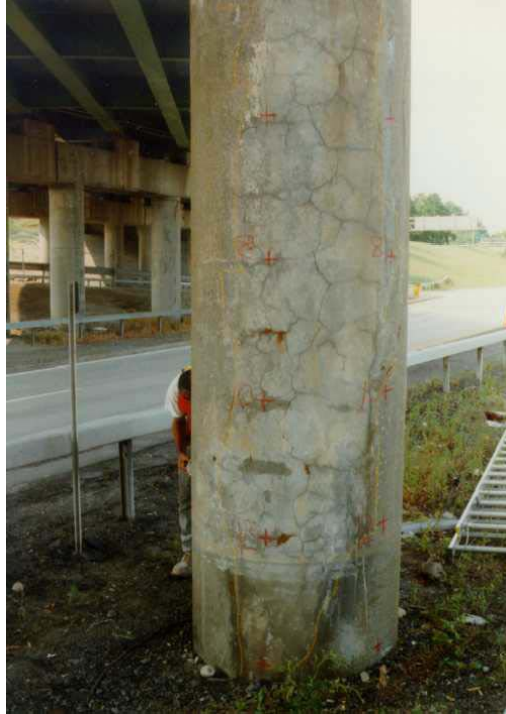
Figure 39. Photo. Second view of cracks and rust staining in patched and nonpatched areas of the columns of the Campus Loop Bridge in Albany, NY, during the second visit in 1996.
