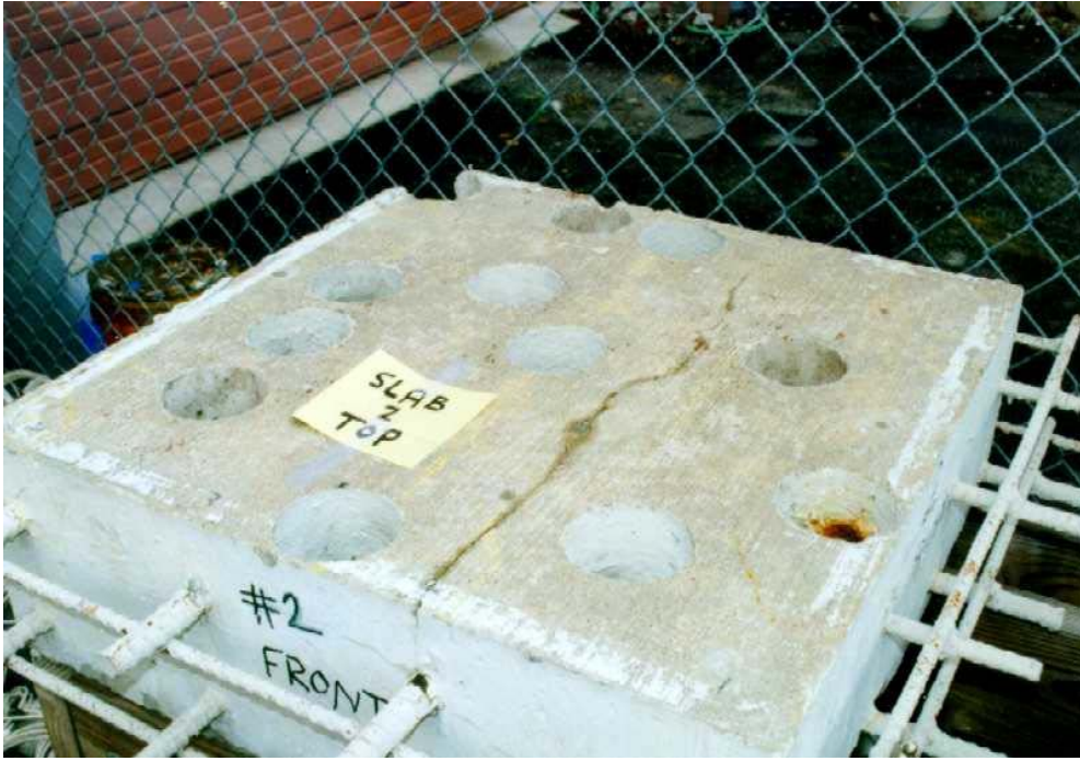
Figure 8. Photo. Corrosion on the ends of rebars exposed in core holes of slab 2.
