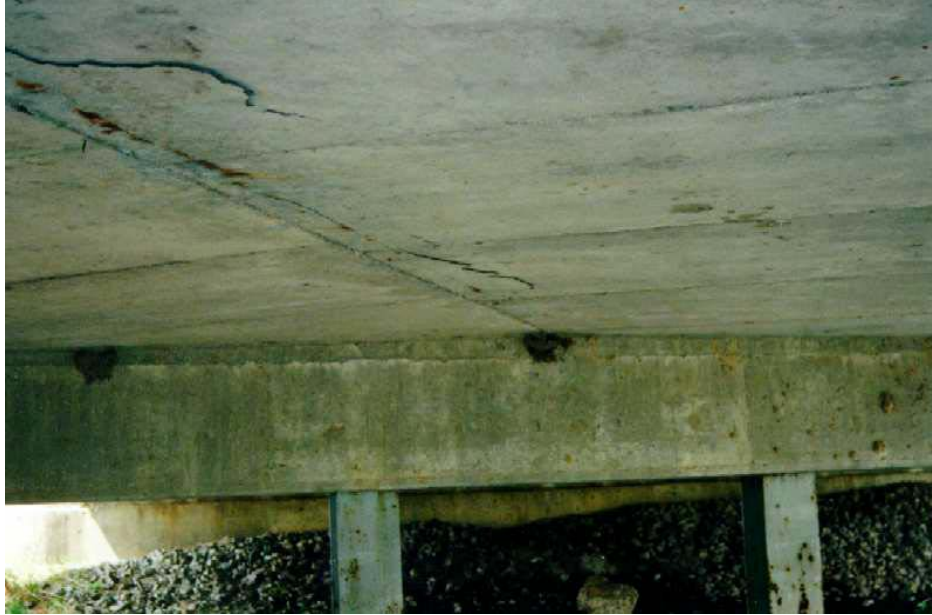
Figure 28. Photo. Cracking, rust staining, and spalling on the soffit of the bridge.
