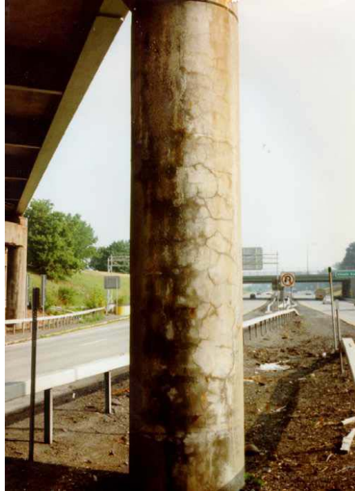
Figure 37. Photo. Cracking on the patched areas on one of the columns of the Campus Loop Bridge in Albany, NY, during the first evaluation in 1995.
