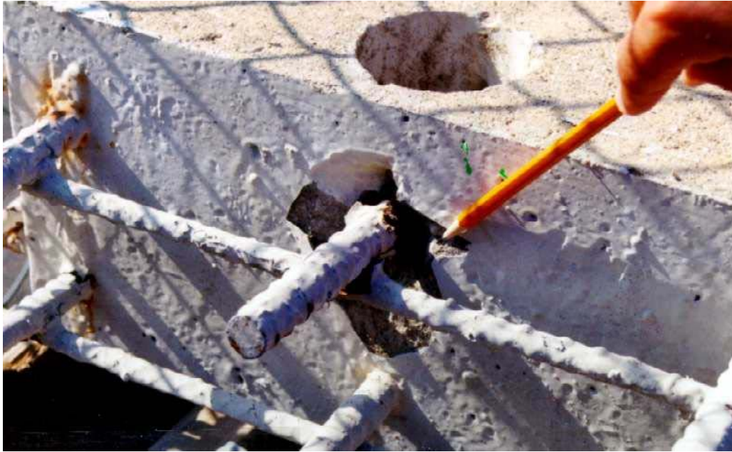
Figure 11. Photo. Corrosion and spalling on one rebar at the concrete-air interface on the side of slab 3 in September 1997.
