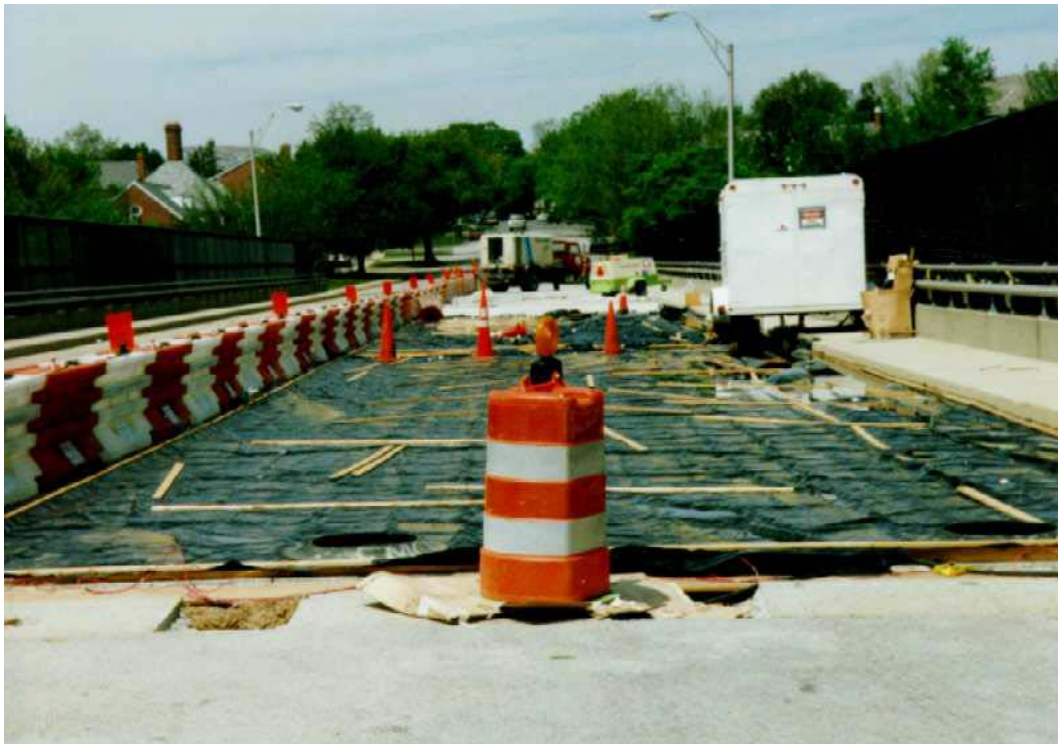
Figure 33. Photo. Northern half of the eastbound lane of 34th Street bridge in Arlington, VA, during ECE treatment.
