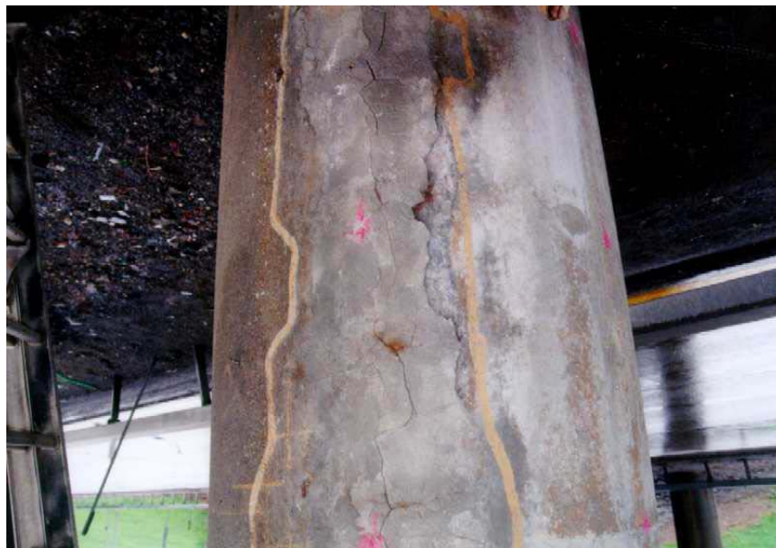
Figure 44. Photo. Third view of a completely delaminated patch (marked in yellow) on a column of the Campus Loop Bridge in Albany, NY.
