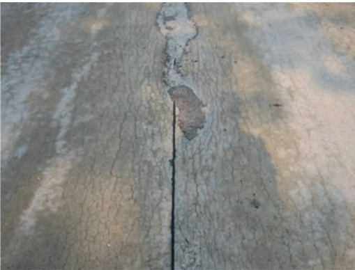
Figure 19. ASR cracking exacerbated by freezing and thawing of concrete pavement.
