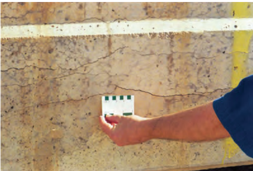
Figure 17. ASR-affected pre-stressed concrete box girder. Cracking became visible after two years.
