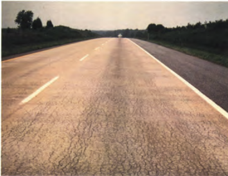
Figure 7. Preferred alignment of cracks in an ASR-affected concrete pavement.
