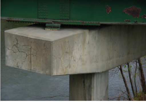
Figure 15. Bent cap showing signs of ASR only where the element has direct access to moisture.
