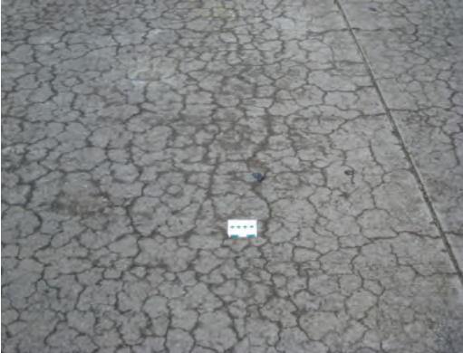
Figure 16. ASR cracks enhanced as the concrete starts to dry following rainfall.
