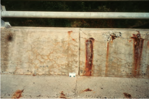
Figure 18. Corrosion of embedded steel in ASR-affected concrete parapet wall.
