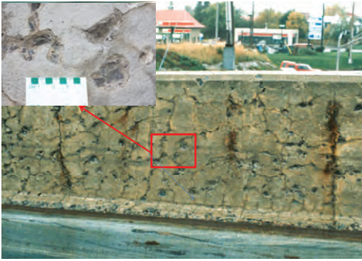
Figure 13. Map-cracking accompanied by numerous pop-outs caused by shaly limestone particles.
