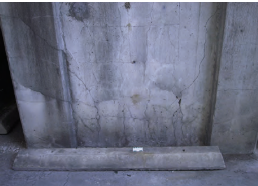
Figure 20. Cracking at the base of a concrete column affected by ASR and DEF.
