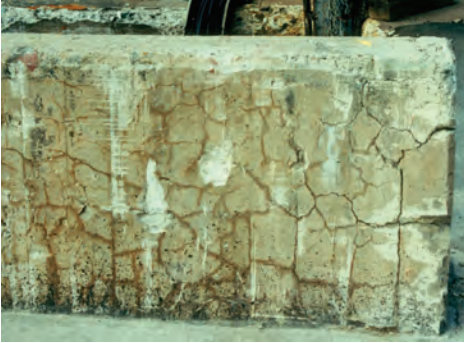
Figure 6. Map cracking (a.k.a. pattern cracking or alligator cracking) in a concrete wall.
