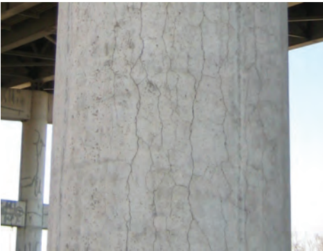
Figure 8. Preferred alignment of cracks in an ASR-affected concrete column.
