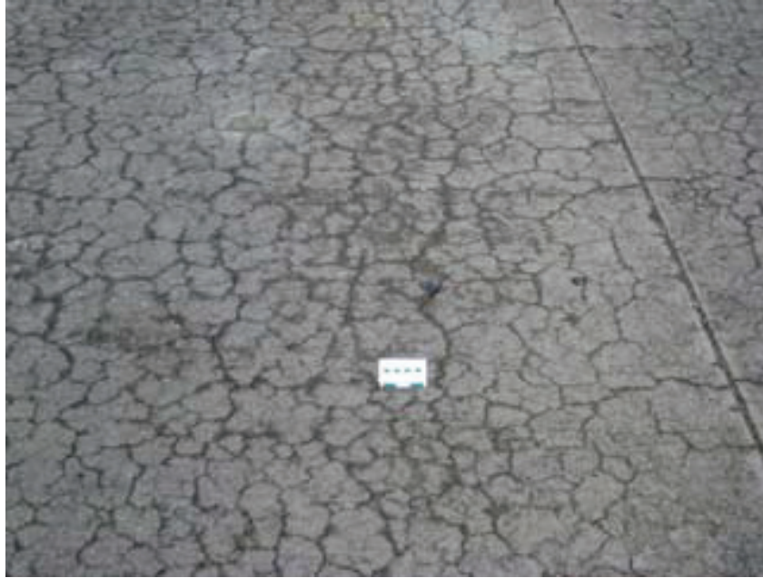
Figure 7 – Map Cracking of Concrete Pavement (Condition State 3)
