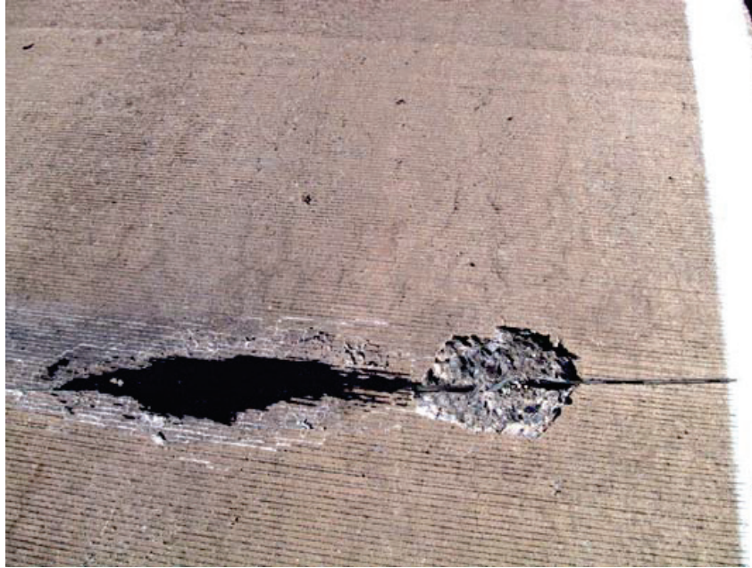
Figure 9 – Joint Deterioration in Concrete Pavement (Condition State 3)
