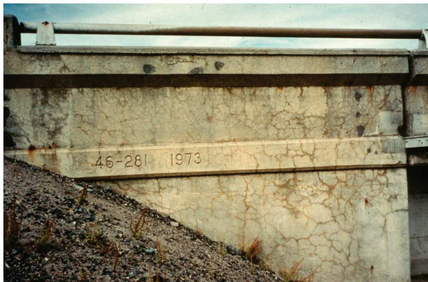
Figure 2 – Map cracking on bridge abutment (Condition State 3)
