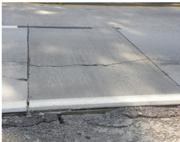
Figure 9. Longitudinal cracking at a jointed FDR location.
