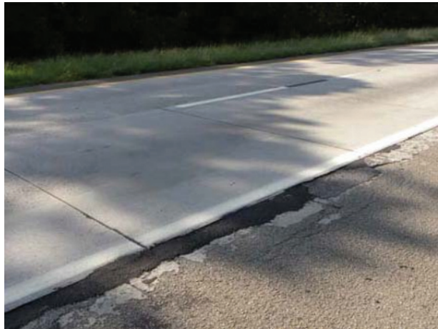
Figure 8. Views of the I-95 jointed FDRs.
