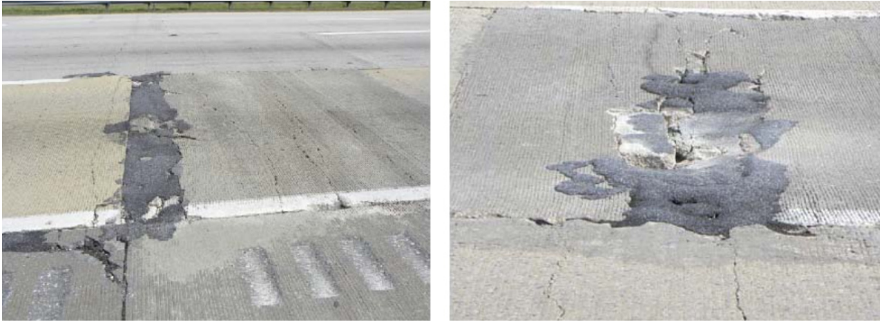
Figure 5. Failed FDRs on CRC pavements.
