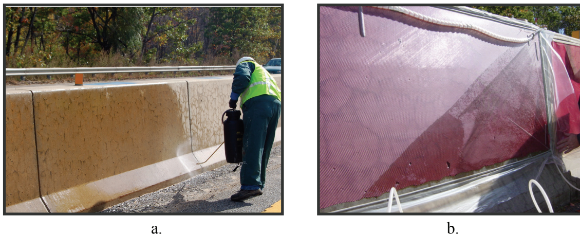
Figure 8.7. Photograph showing topical application (a) and vacuum application (b) of 30%- \text{LiNO}_3 solution to highway barrier in Massachusetts
