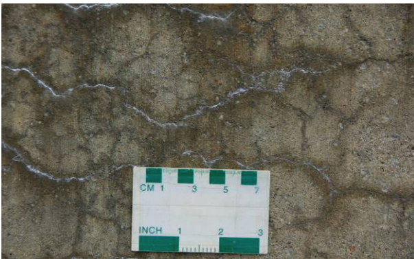
Figure 3.5. (A). Pop-out created by the expansion of a frost-susceptible porous coarse aggregate particle (leached chert). (B). ASR-induced pop-out in a concrete pavement incorporating highly-reactive aggregates; also noted pattern cracking. (C). Efflorescence and exudations of alkali-silica gel at the surface of the concrete foundation of a 25-year-old highway bridge affected by ASR. (D). Efflorescence and exudations of alkali-silica gel at the surface of a small concrete monument affected by ASR. (E). Surface discoloration and exudation associated with cracks.
