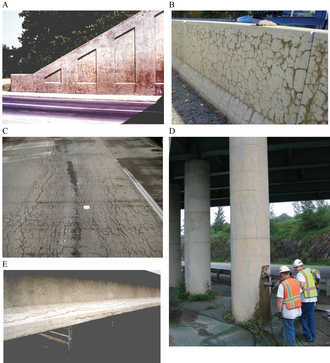
Figure 3.1. (A). Map-cracking in the wing wall of a 30-year-old bridge structure affected by ASR (CSA 2000). (B). Severe map-cracking and associated gel staining around cracks in a median highway barrier affected by ASR. (C). Well-defined crack pattern associated with the development of ASR in highway pavement; the orientation of predominant cracks is longitudinal, while map- or pattern-cracking is also identified. (D). Preferred alignment of cracks in an ASR-affected concrete column. (E). Longitudinal cracking in a precast, reinforced concrete beam affected by ASR.
