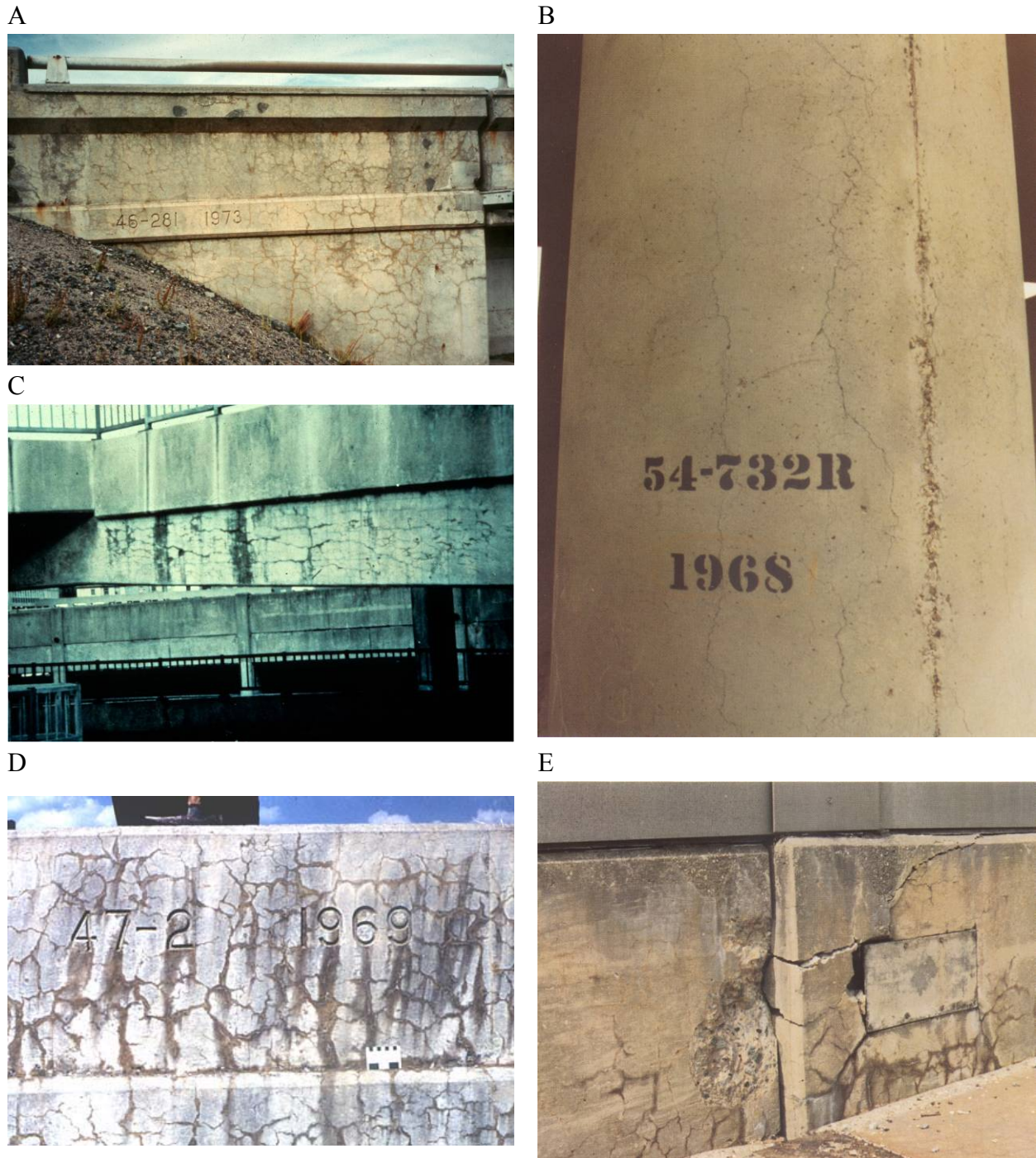
Figure 7.2. ASR-related defects in bridge elements and severity assessment. A. Map cracking on bridge abutment (condition state 3). B. Aligned cracking on column (condition state 2). C. Aligned cracking in beam (condition state 3). D. Gel exudation (condition state 3). E. Relative dislocation/misalignment, leading to loss of clearance and cracking (SHRP C-315 1991) (condition state 3).
