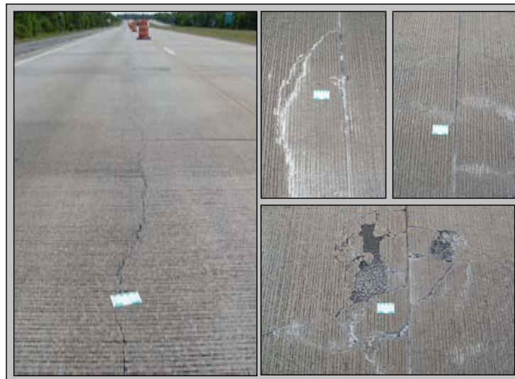
Figure 8. Typical distress observed in concrete pavement near Pine Bluff, AR.
