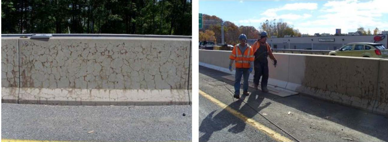
Figure 11. Typical ASR damage on barrier walls (left) and barriers treated with elastomeric coating.
