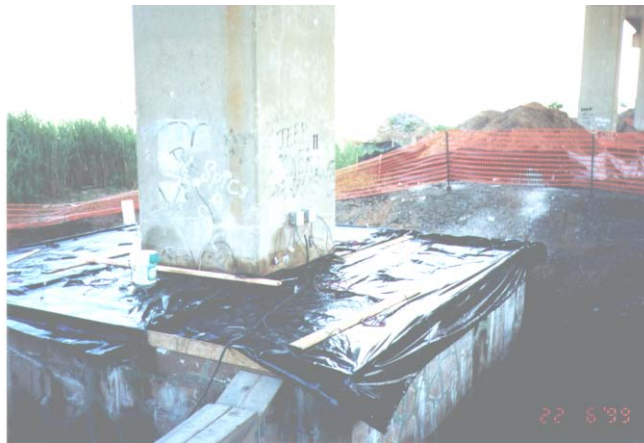
Figure 4. Repair of pier footings of a highway structure suffering from severe cracking and spalling due to ASR using an electrochemical system for lithium impregnation.
