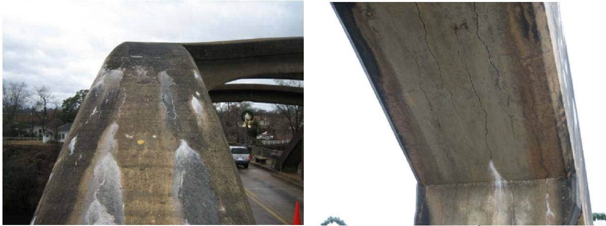
Figure 7. Cracking on top and underside of archway supporting 5 th span.
