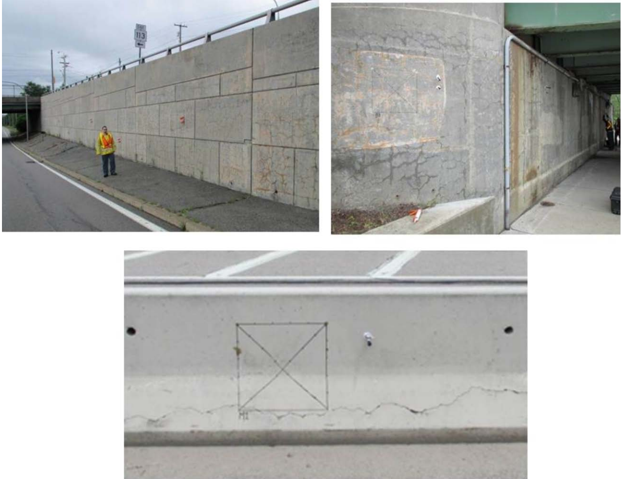
Figure 15. Cracking in retaining wall (top left), wing wall and bridge abutment (top right), and median barrier wall (bottom).
