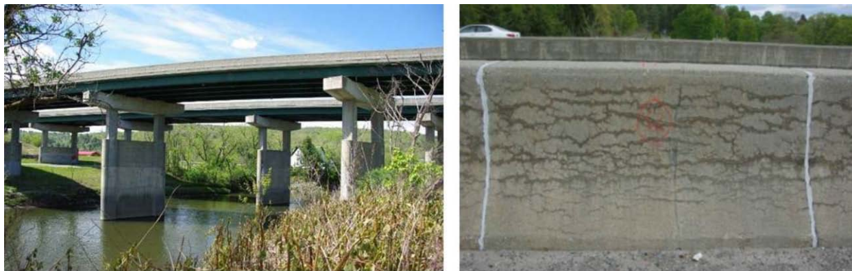
Figure 16. Bridges (left) carrying I-89 over U.S. 2/State St. and the Dog River near Montpelier, VT, and cracking on barrier walls (right).
