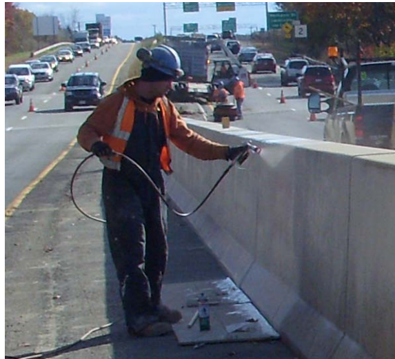
Figure 128. Elastomeric paint sprayed in 2010 onto barrier sections previously treated with 40 percent silane in 2005 by MassDOT.
