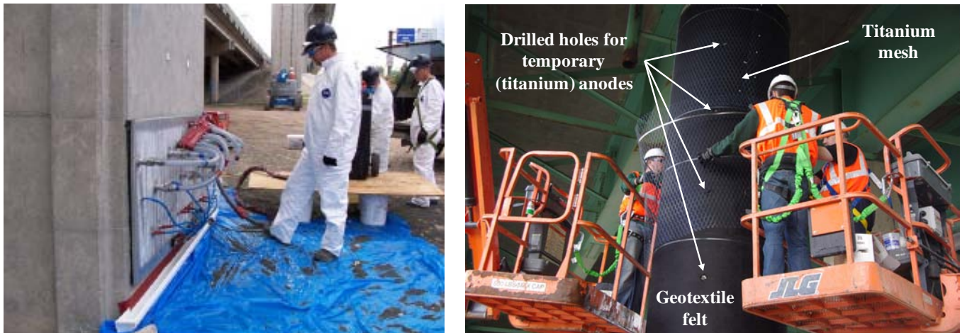
Figure 25. Lithium treatment using vacuum impregnation in Texas (left) and electrochemical migration in Maine (right).
