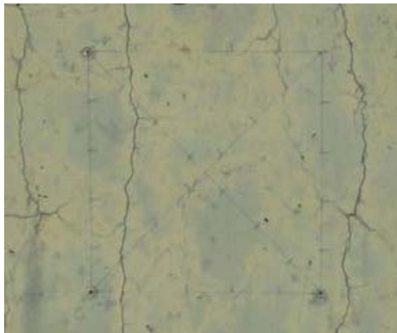
Figure 210. Visual observation of Column 36 West face.
