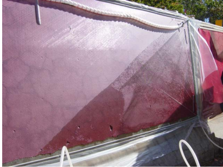
Figure 127. Vacuum impregnation of 30 percent lithium nitrate solution into highway barrier. This photograph was taken shortly after the solution was entered into the system under vacuum. Once a full vacuum was obtained, the vacuum was held for either 15 minutes (short term) or 7.5 hours (long term).
