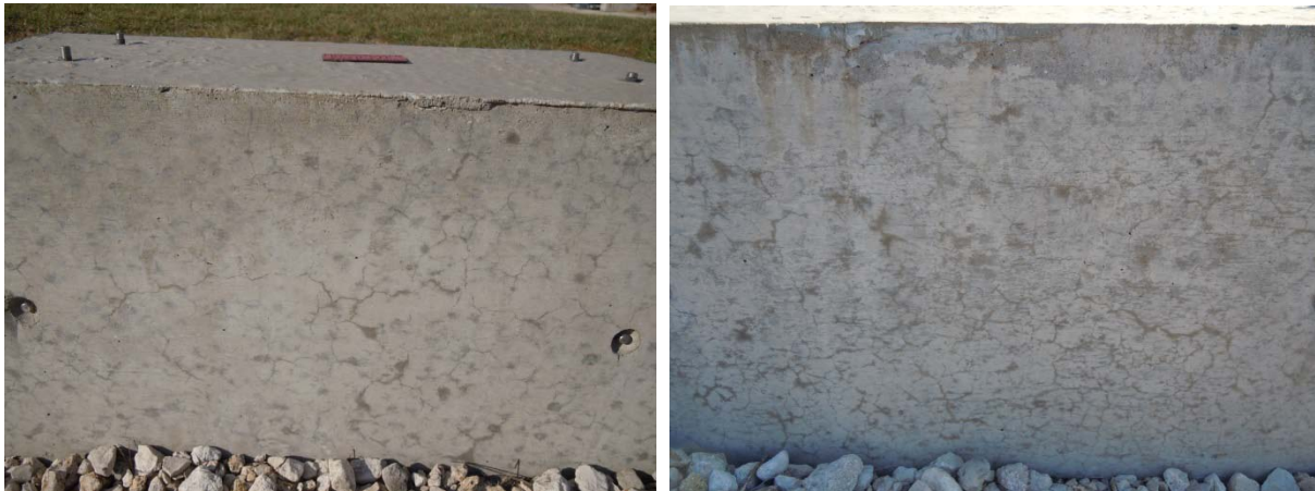
Figure 183. Visible cracking of replicate exposure blocks to beam 3 (with fly ash), on the left, and beam 4 (without fly ash), on the right. It is important to note that both blocks cracked about 1.5 – 2 years after casting without exhibiting measurable expansion.
