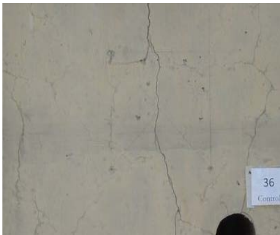
Figure 211. Visual observation of Column 36 North face.
