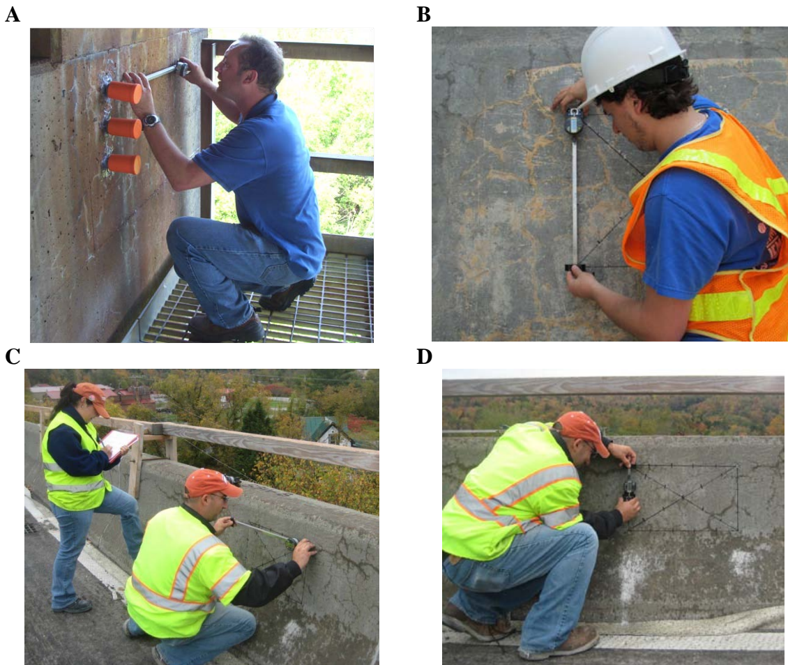
Figure 10. Expansion measurements using DEMEC gauges. A-C: 500-mm (~ 20 in.) gauge length. D: 150-mm (~ 6 in.) gauge length.
