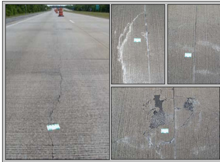
Figure 43. Typical distress observed from visual inspection of pavement.
