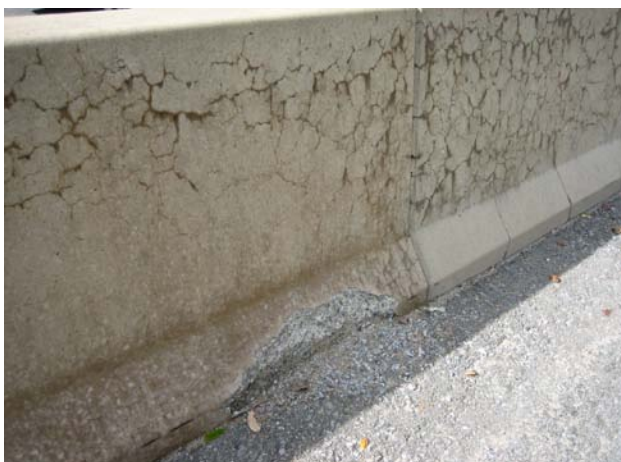
Figure 119. Example of freezing and thawing damage at bottom (haunch) of barrier.
