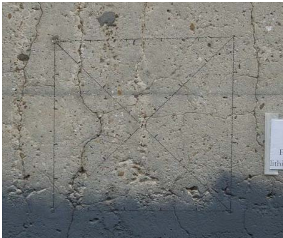
Figure 222. Visual observation of Column 46 Southwest face.
