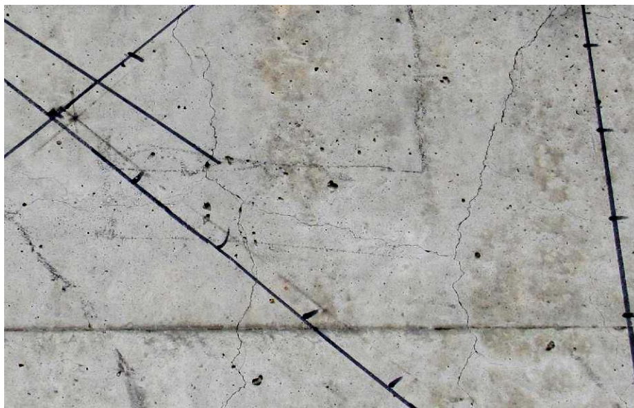
Figure 88. Enlargement of a section of the crack map at Site 1 (external and somewhat exposed to moisture) showing light cracking on column No. 1 of the I-395 bridge over the Penobscot River (2012).
