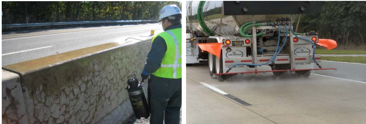
Figure 24. Topical application of lithium on barrier wall in Massachusetts (left) and concrete pavement in Delaware (right).
