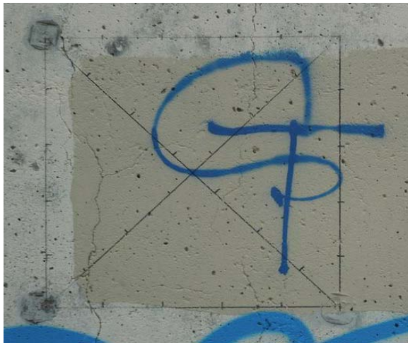
Figure 220. Visual observation of Column 45 Southwest face.
