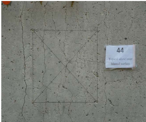
Figure 218. Visual observation of Column 44 Southwest face.
