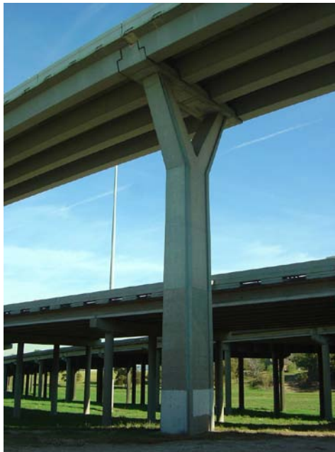
Figure 185. Typical column at Houston, TX test site.
