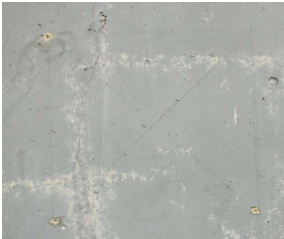
A – Column 43 SW Face 2006
