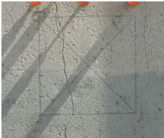
Figure 207. Visual observation of Column 34 North face.
