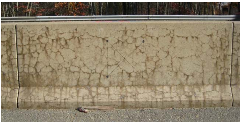
Figure 118. Typical example of cracking and staining observed on highway barriers on Route 2 in Leominster, MA.
