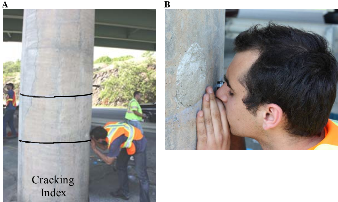
Figure 14. Cracking index measurements on the columns of the South Parkway bridge over I-395 (Maine). The crack mapping operator is measuring crack widths using a magnifying hand lens.
