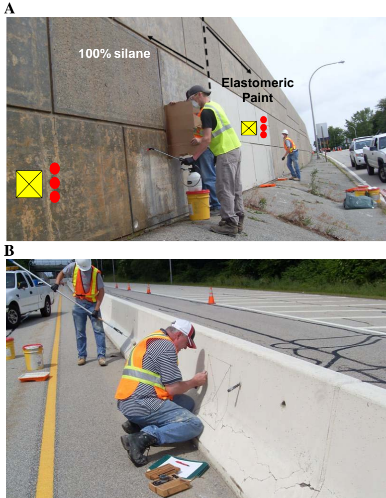
Figure 232. Examples of treatment and monitoring plans for different structures on Post Road in Warwick, RI.
