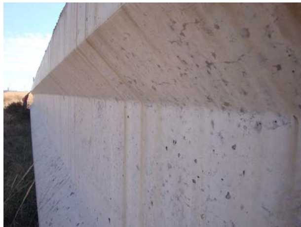
Figure 172. Typical cracking observed on the precast beams.
