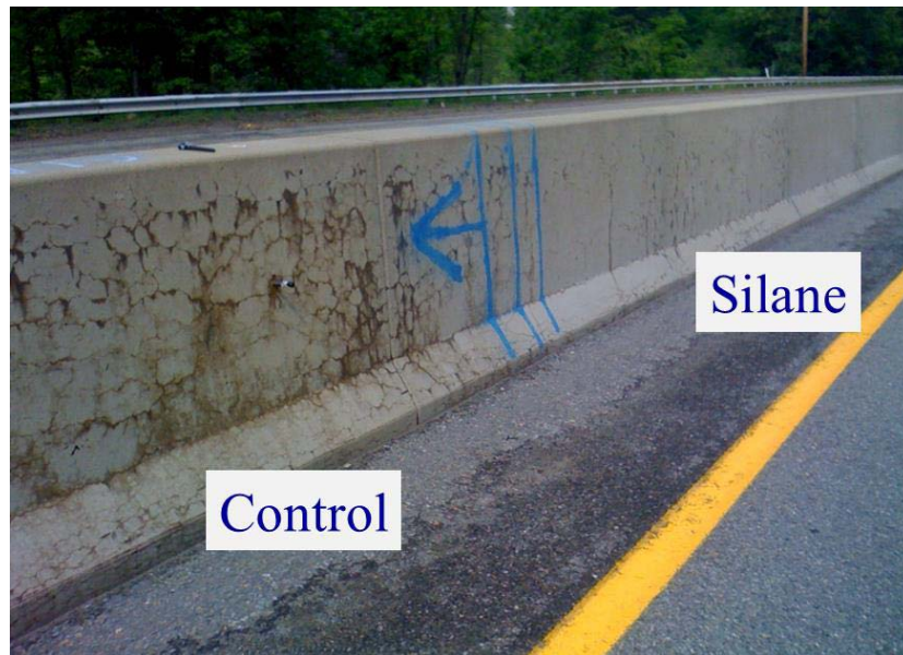
Figure 169. Significant reduction in visible cracking for the barriers treated with 40 percent silane (right), compared to untreated barriers (left).
