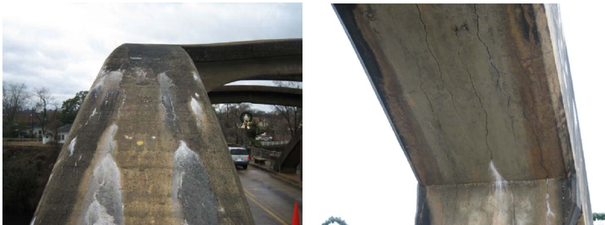
Figure 29. Cracking on top and underside of archway supporting 5 th span.
