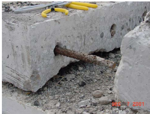
Figure 10. Lack of bond between inserted rebar and concrete. (20)
