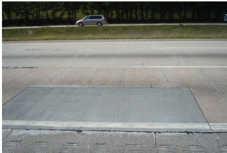
Figure 13. Half-lane-width FDR on I-77 in South Carolina.
