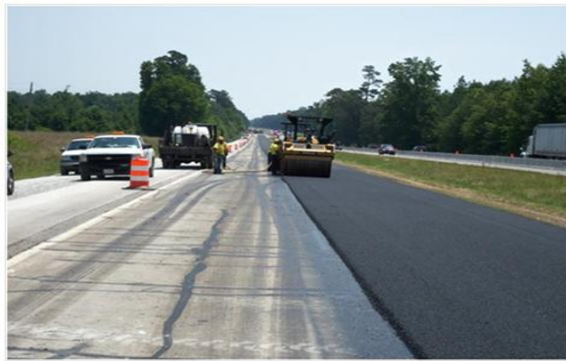
Figure 20. Unbonded overlay on U.S. Route 58 in Virginia. Placement of AC porous friction course.
