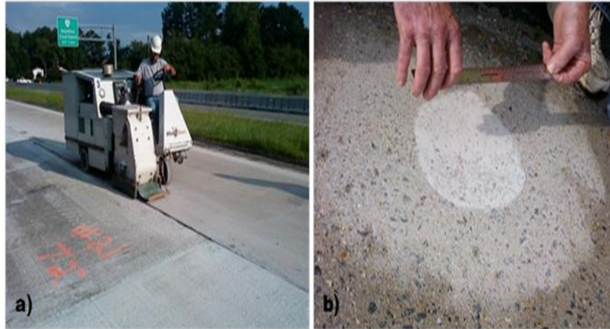
Figure 18. a) Surface preparation for bonded overlay on U.S. Route 58 in Virginia; b) Closeup view of surface after preparation.
