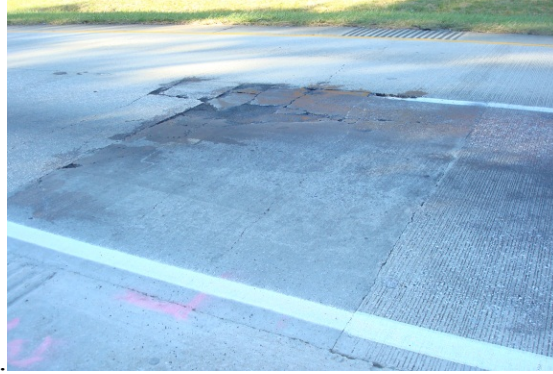
Figure 14. Failure of FDR.
