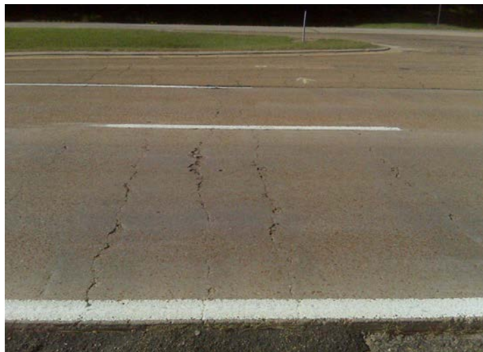
Figure 3. Spalling at CRCP transverse cracks.
