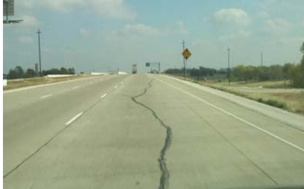
Figure 1. Longitudinal crack in CRCP.
