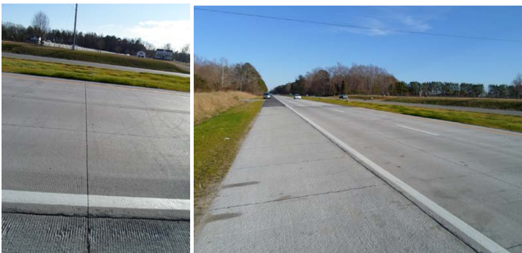
Figure 21. Unbonded overlay on U.S. Route 58 in Virginia, as constructed, with 6 ft by 6 ft joint layout.
