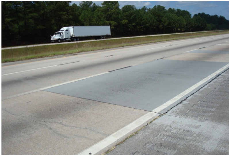
Figure 12. Full-lane-width FDR on I-77 in South Carolina.
