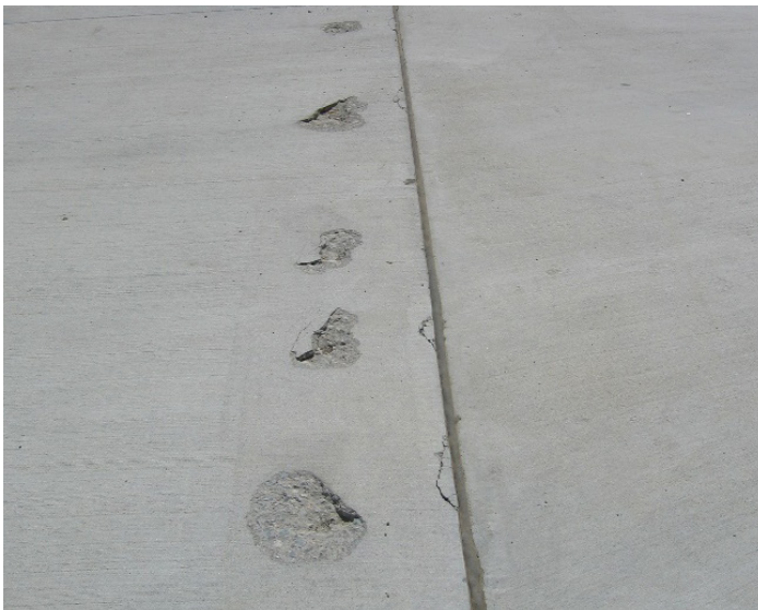
Figure 3. Misaligned dowel bars causing surface distress
