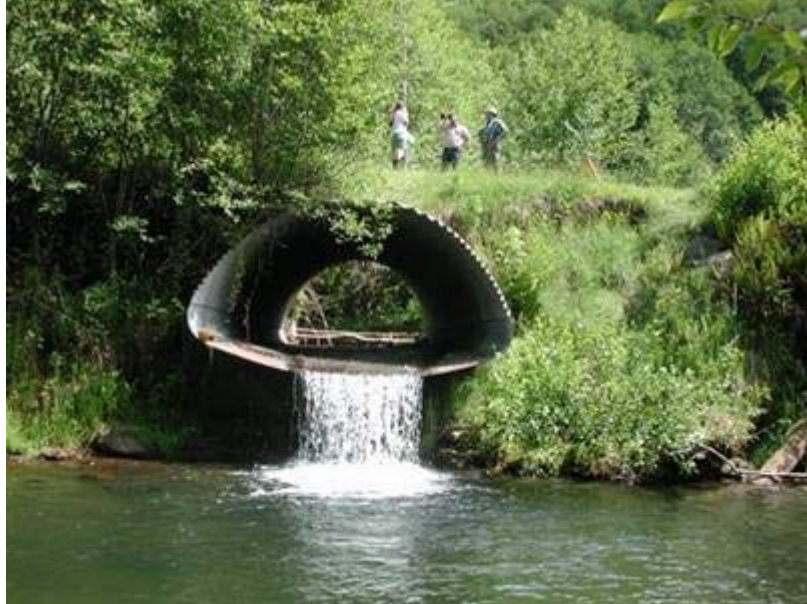
Figure 1.2 Downstream channel degradation causing culvert to become perched, and presenting a low flow barrier to fish passage (Furniss 2006)
