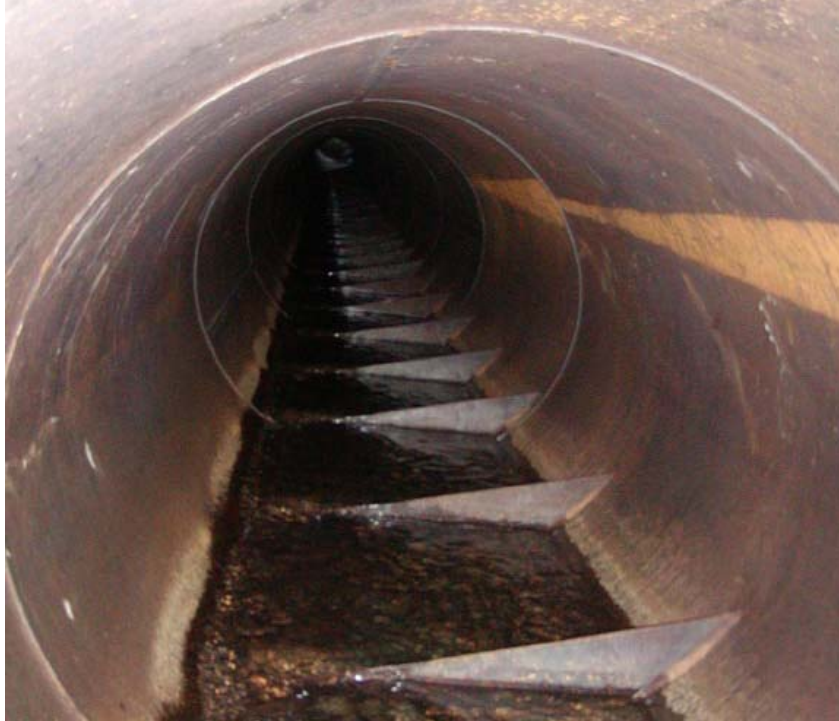
Figure 8.14 Steel corner baffles welded to the pipe and spaced 1.22 m (4 ft) apart, John Hatt Creek
