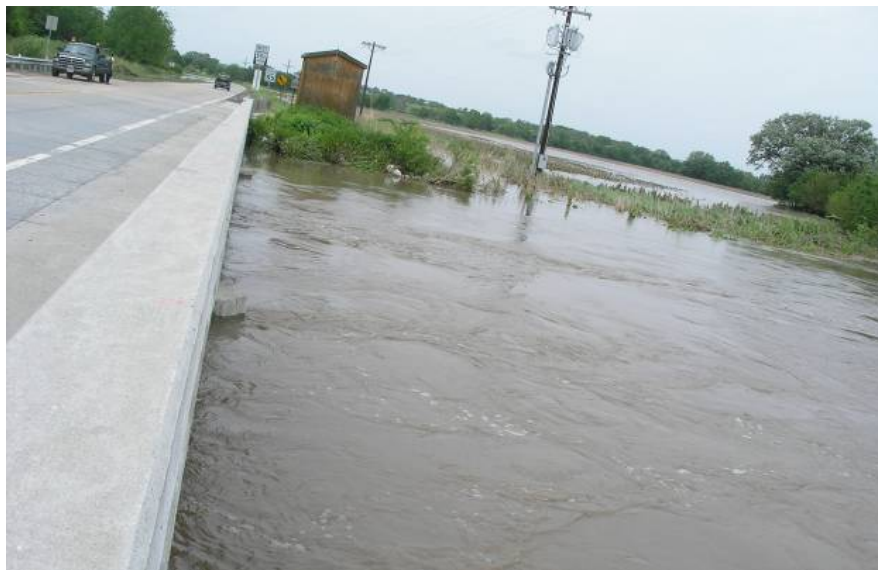
Figure 1. Photo. Partially inundated bridge deck at Salt Creek, NE.
