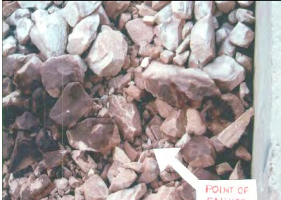
Figure 5.9. Riprap failure in 1997 tests ( d_{50} = 0.89 ft (271 mm)).
