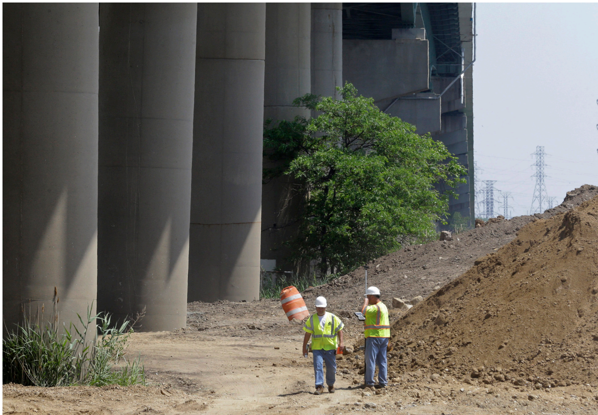
Figure 3-14 Tilting columns adjacent to stockpile (courtesy DeIDOT).
