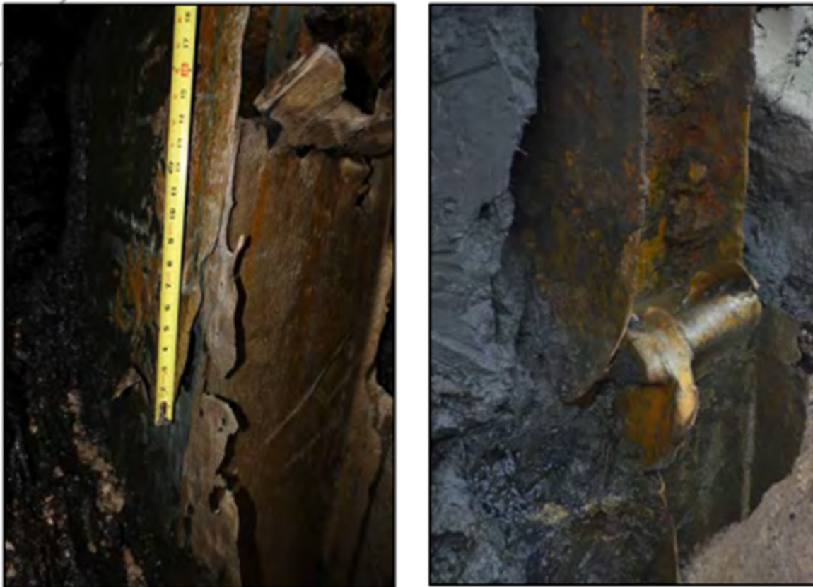
Figure 3-10 Corrosion and resulting buckling of foundation pile (courtesy Wisconsin Department of Transportation).
