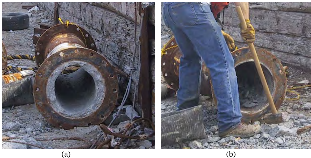
Figure 9-7 Tremie Must be Clean; (a) Tremie Contaminated with Hardened Concrete; (b) Worker Cleaning Tremie
