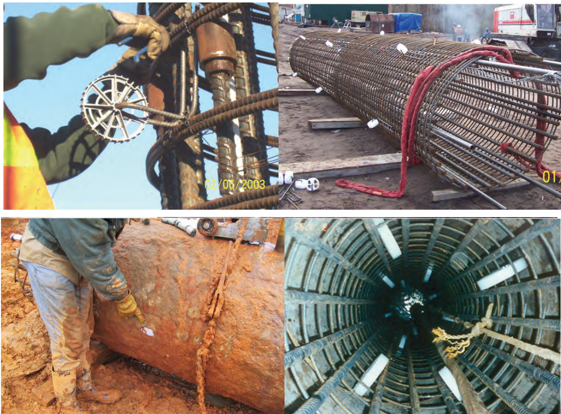
Figure 8-16 Roller Centralizers on Reinforcing Cage. Clockwise from top left: mounting external roller centralizer on the cage; completed cage with centralizers; rollers attached to hoop reinforcement; extracted shaft revealing centralizer on surface.
