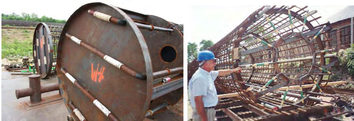
Figure 9-19 Sleeve Port Systems for Distribution of Grout to the Base of the Shaft
