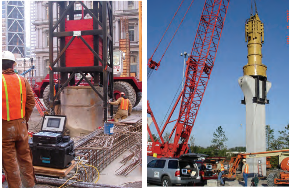
Figure 17-35 Dynamic Load Test of Drilled Shafts using Drop Weight (left) and Pile Hammer (right). [Photos courtesy of Pile Dynamics, Inc. (left) and Ross McGillivray (right)]
