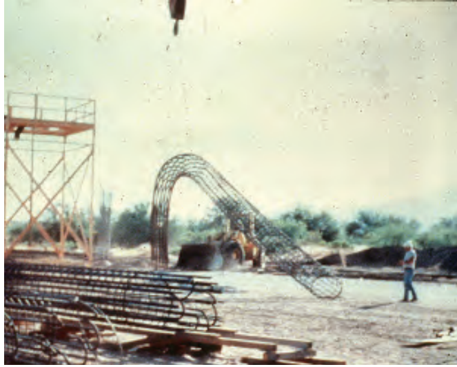
Figure 8-20 Photograph of Rebar Cage Being Lifted Improperly (Photo courtesy of Barry Berkovitz, FHWA)
