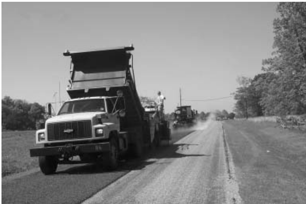
State and local highway agencies are applying more and more preservation treatments to their roads, such as the chip seal shown here.
