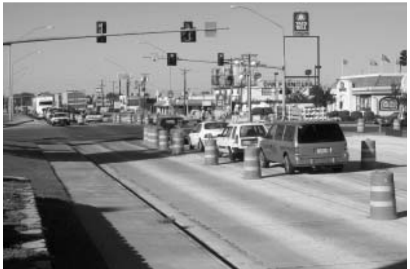
Three intersections in Kennewick, Washington, were completely closed to traffic for 3 days, allowing for uninterrupted reconstruction work.
