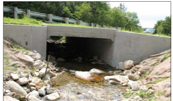
Figure 10: Hydraulically, geomorphically, and ecologically compatible structure that withstood Hurricane Irene and other flood events. (Readsboro VT 8 Bridge, VTrans photo).
