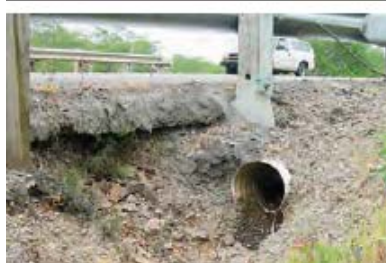
Fig. 7: Field Examples of Culvert Conditions from Oregon DOT's Culvert Assessment Guide
