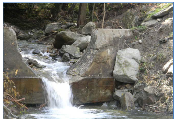
Figure 9: Culvert washed out by Hurricane Irene. (VTrans photo).
