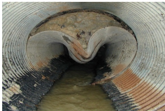
Figure 4: Culvert Collapse on I-480 in Cleveland in 2001. (Ohio DOT)
