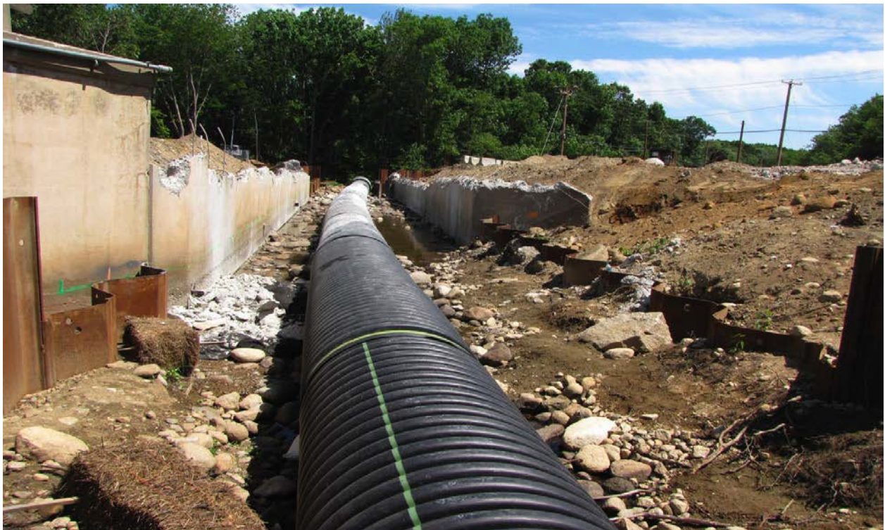
Figure 9. Abutment walls of old bridge left in place so work does not impact stream.
