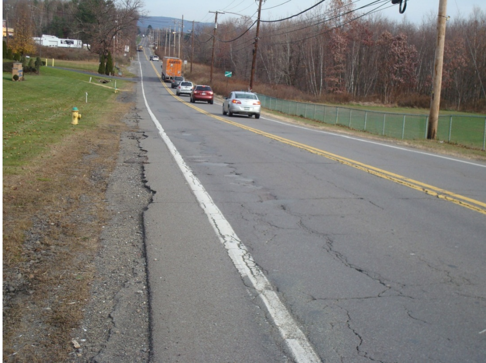
Figure 4. Photo. Existing roadway showing severe fatigue cracking and other distresses.
