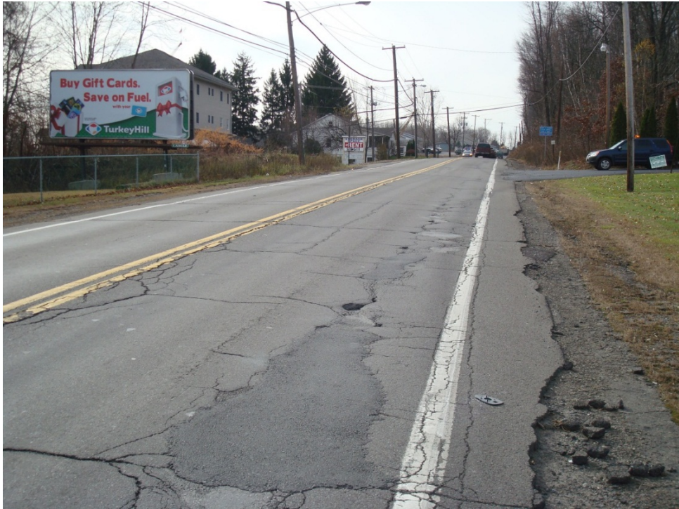
Figure 5. Photo. Close-up of existing roadway showing severe fatigue cracking and other distresses.
