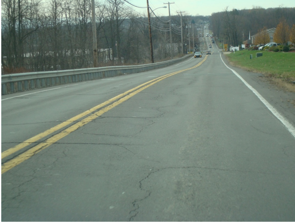
Figure 2. Photo. Existing roadway showing deteriorated condition.
