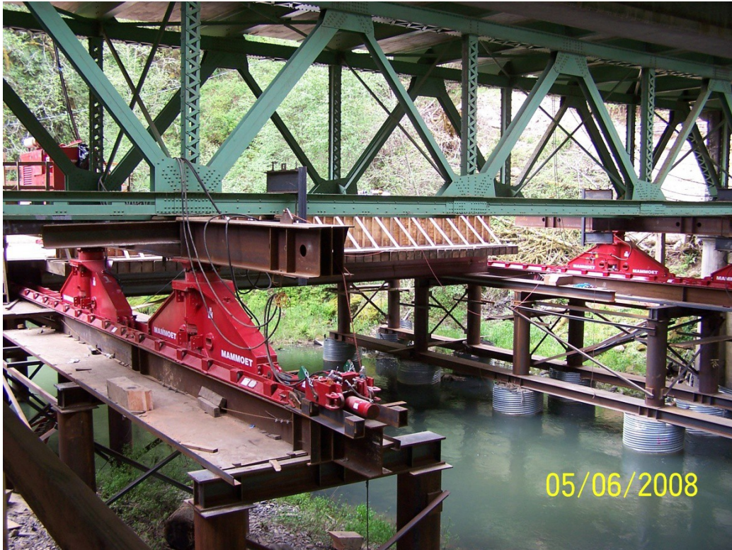
Figure 19. View of a complete hydraulic sliding system, including hydraulic jacks, hydraulic pumps, and the railing system.
