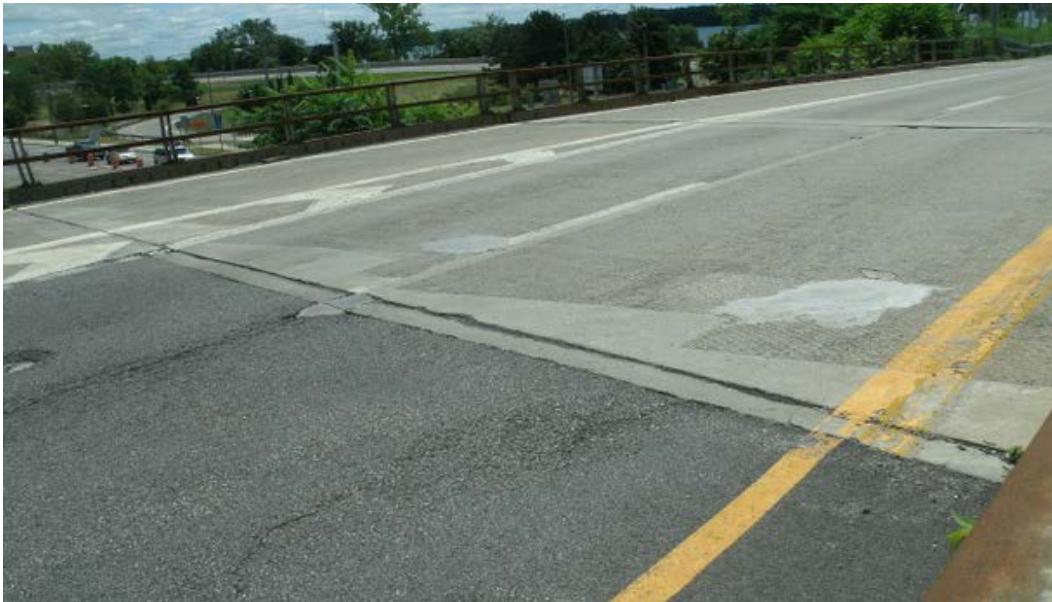
Figure 3. Photo. View of deck over end joint showing patched cracks and spalls.
