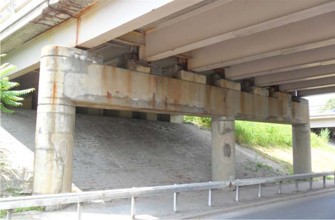
Figure 5. Photo. Delamination and spalling at pier columns and cap.
