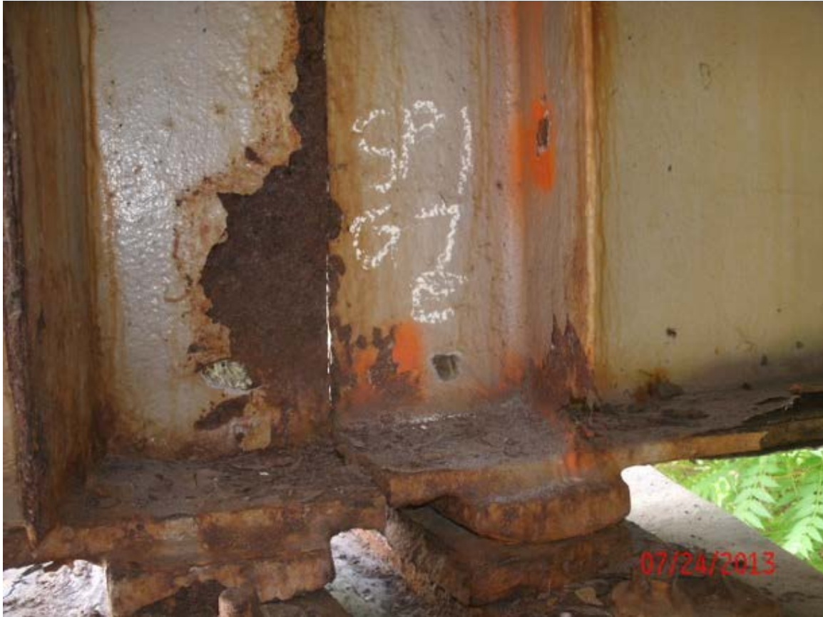
Figure 7. Photo. Severe section loss at end of girders.
