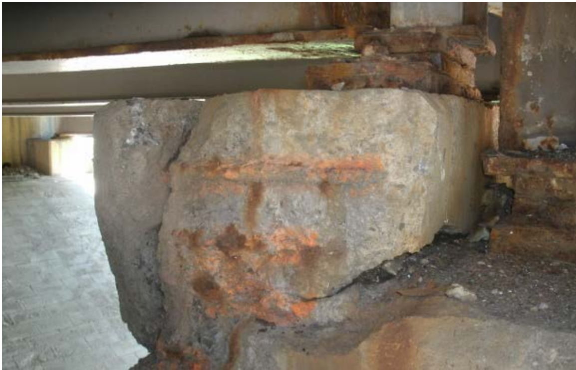
Figure 6. Photo. Cracked concrete under bridge seat.
