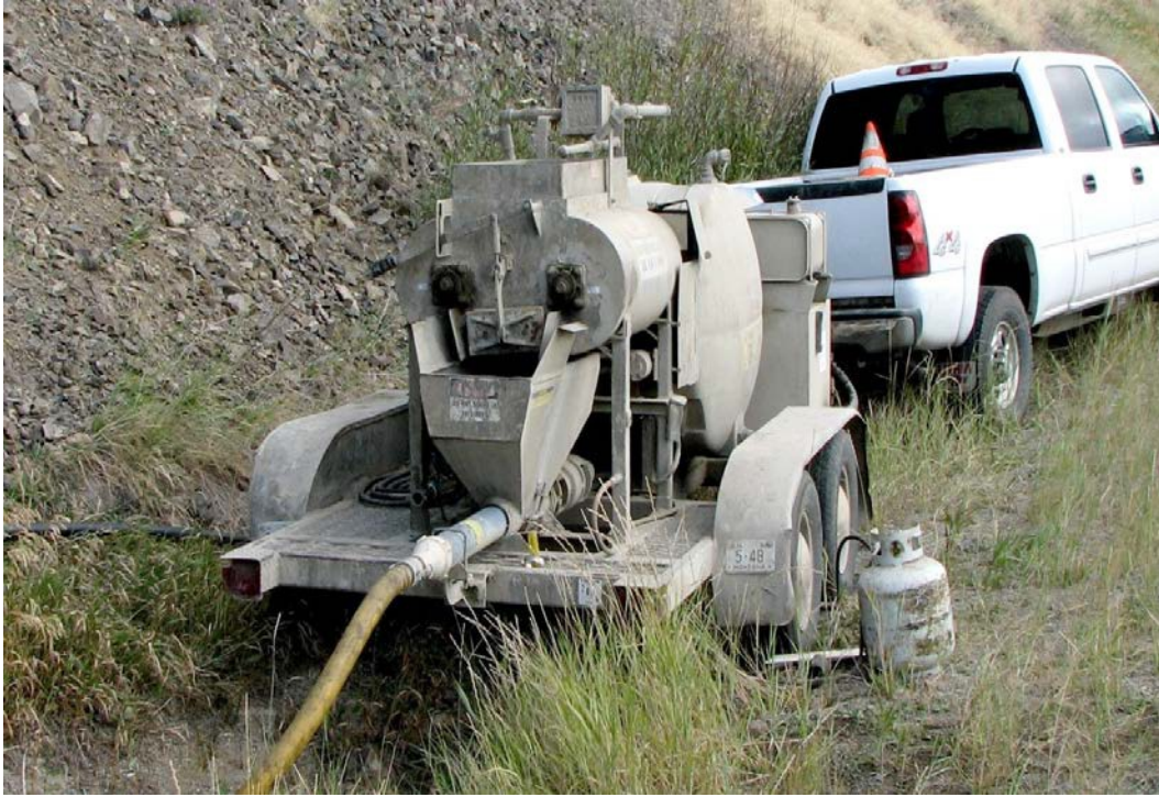
Figure 9. View of the pumping apparatus.
