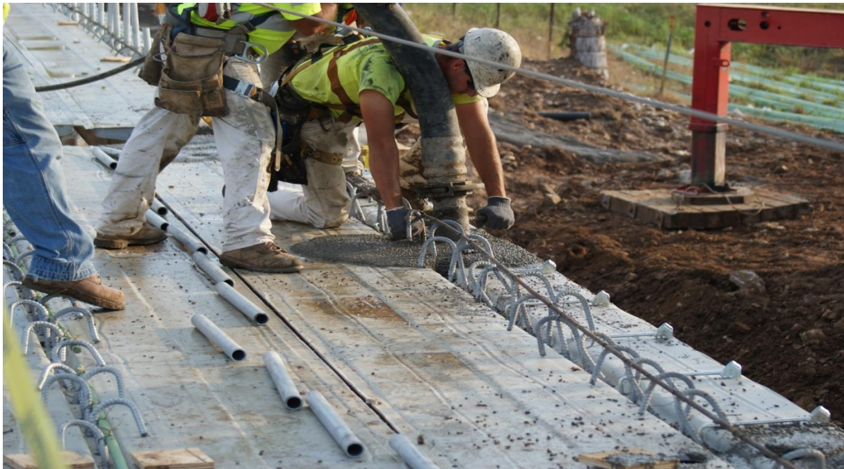
Figure 34. Self-consolidating concrete is pumped into place. Note removal of paving rail bars to allow increased flow around shear steel.
