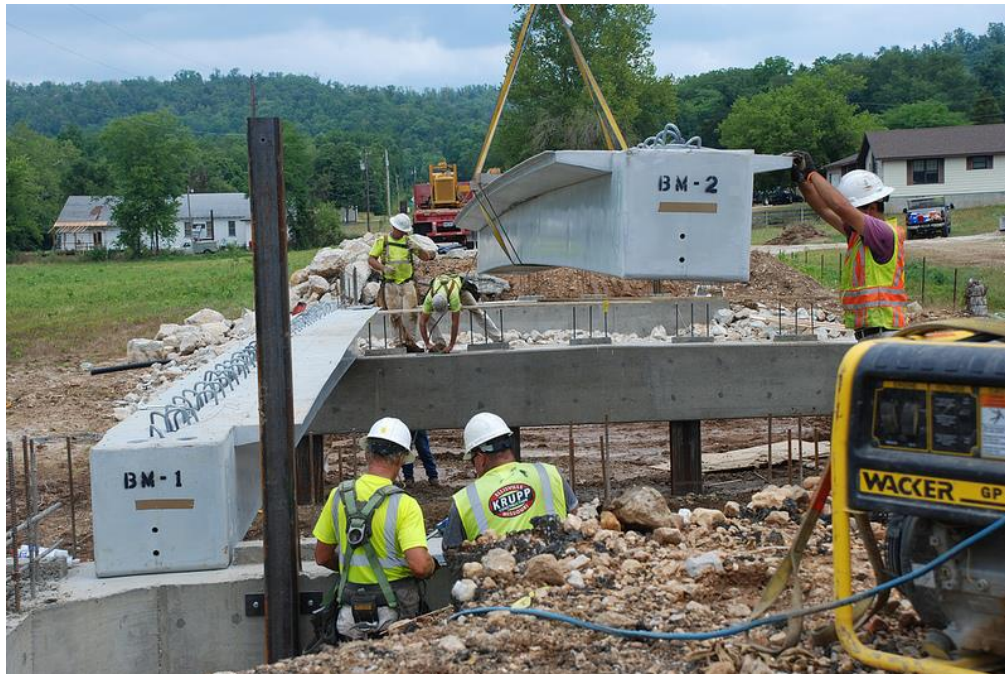
Figure 31. First beams lifted into place over Ottery Creek Overflow. (Photo courtesy of MoDOT)
