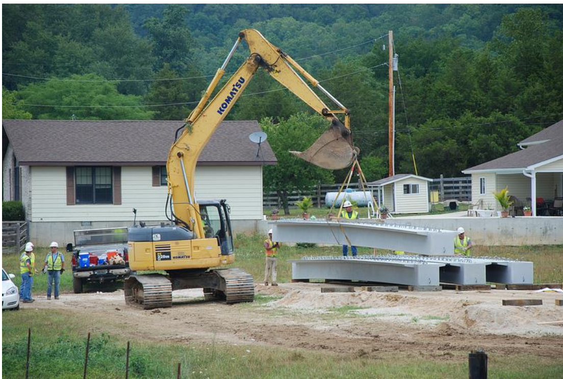
Figure 30. Beams moved to construction site using track hoe. (Photo courtesy of MoDOT)
