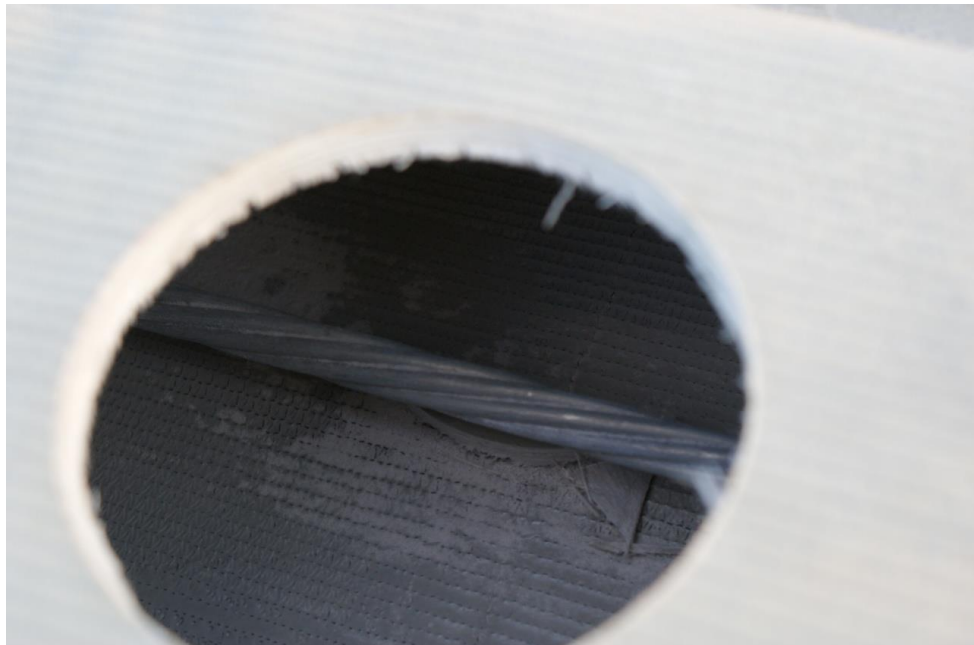
Figure 9. Filler openings located at one-quarter points along the beam top with steel reinforcing strand visible.
