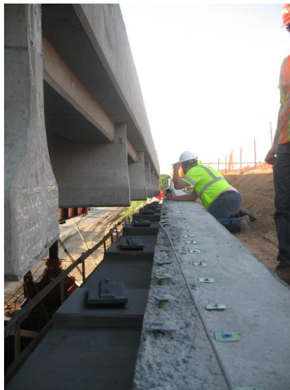
Figure 71. Photo. Another view of the girders before the span was carefully positioned on to the pre-positioned bearing plates on top of the abutment wall.
