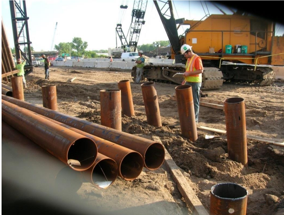
Figure 44. Photo. Steel casing driven into the foundation for CIP concrete piles. Forty 12-inch-diameter CIP concrete piles (75 ft minimum length) were used for each abutment, while six to eight 12-inch-diameter CIP concrete piles (60 ft minimum length) were used for each of the six columns supporting the midspan pier.
