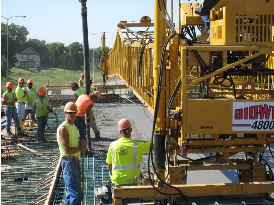
Figure 33. Photo. Close-up view of placing and paving the fiber-reinforced bridge deck concrete.
