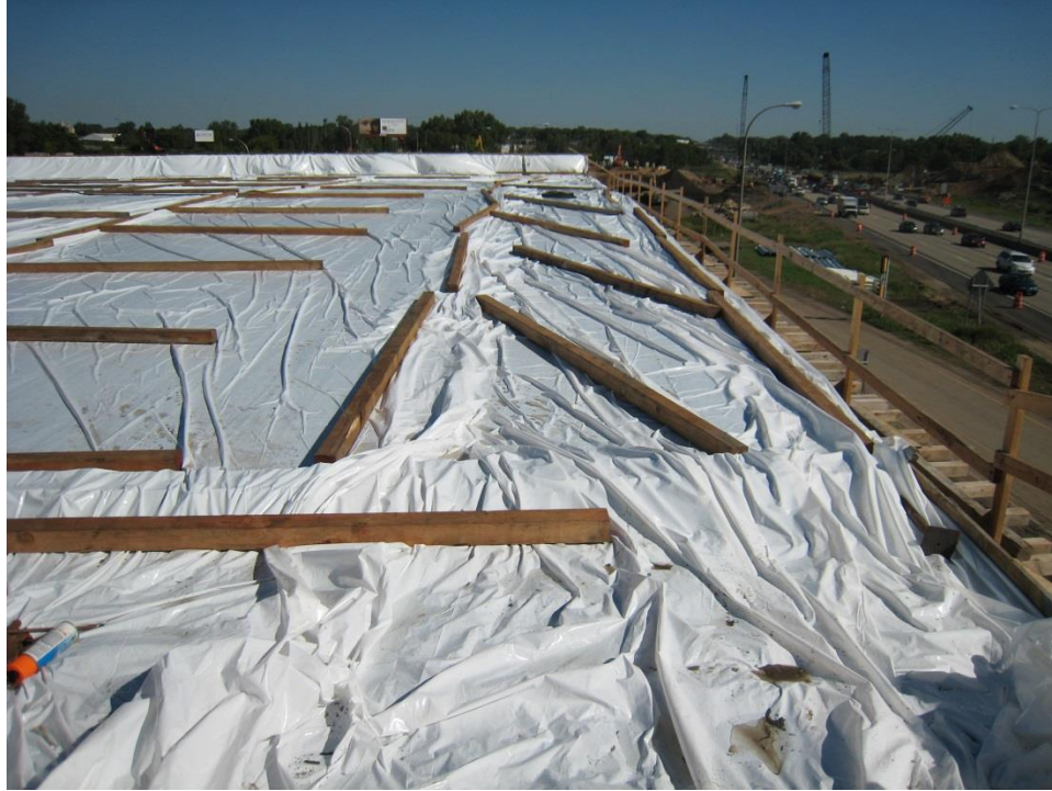
Figure 35. Photo. The concrete was cured by covering with wet burlap when fresh followed by polyethylene sheets after hardening to minimize water evaporation and shrinkage cracking. Note in the background that the Maryland Ave. bridge 6513 has now been demolished and concurrent substructure construction activities are taking place.
