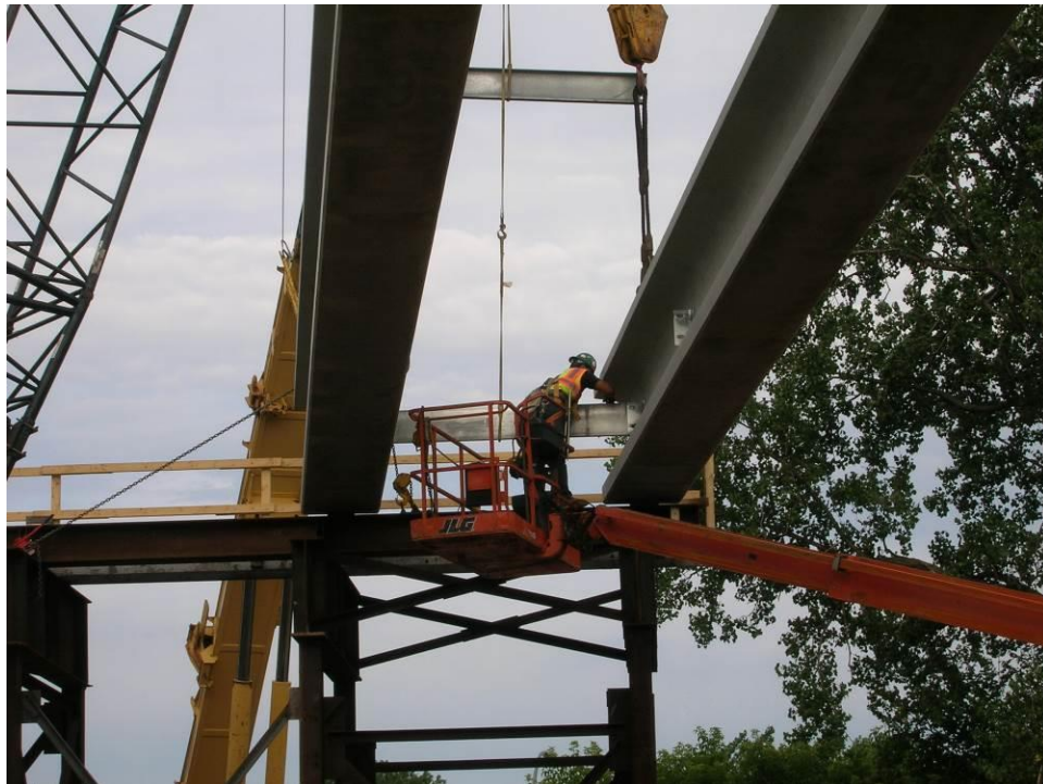
Figure 20. Photo. The girders were braced to each other using steel braces to minimize stresses during transport of the bridge superstructure using the SPMT.
