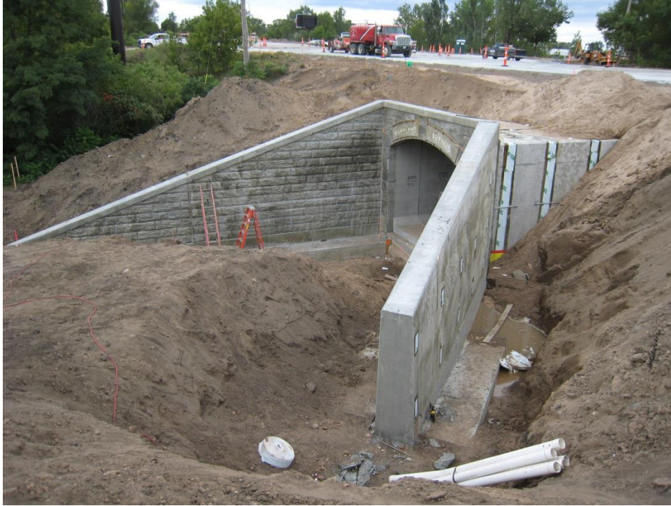
Figure 57. Photo. Close-up view of the box culvert bridge tunnel beneath Maryland Ave. before finishing the earthwork.
