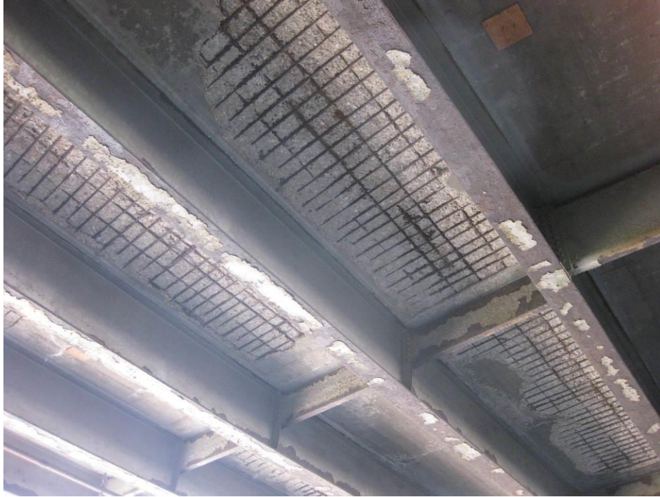
Figure 2. Photo. Delaminated bottom of bridge 6513 deck.
