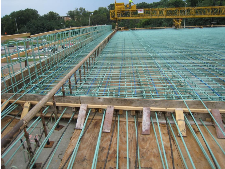
Figure 31. Photo. During paving of the bridge deck, the paver rolled over supported steel tubes.
