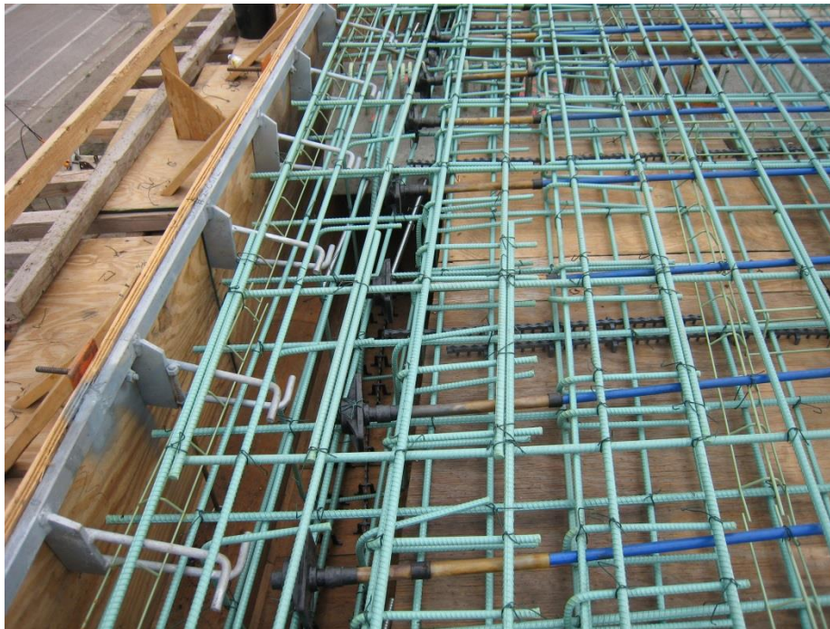
Figure 79. Photo. Forms and reinforcement for the end diaphragm and the expansion joint device hardware.
