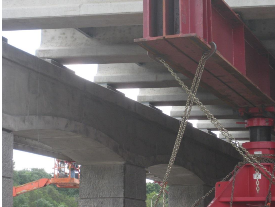
Figure 72. Photo. The girders of the first span resting on the bearing plates above the pier while still being supported by the SPMT.
