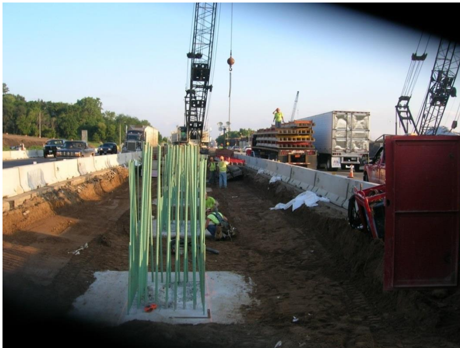
Figure 45. Photo. Construction of the six 10-ft by 10-ft CIP columns (spaced 23 ft apart) supporting the midspan pier. Traffic lanes on I-35E were open to traffic except for the occasional closure of the inside lane for construction equipment and delivery.
