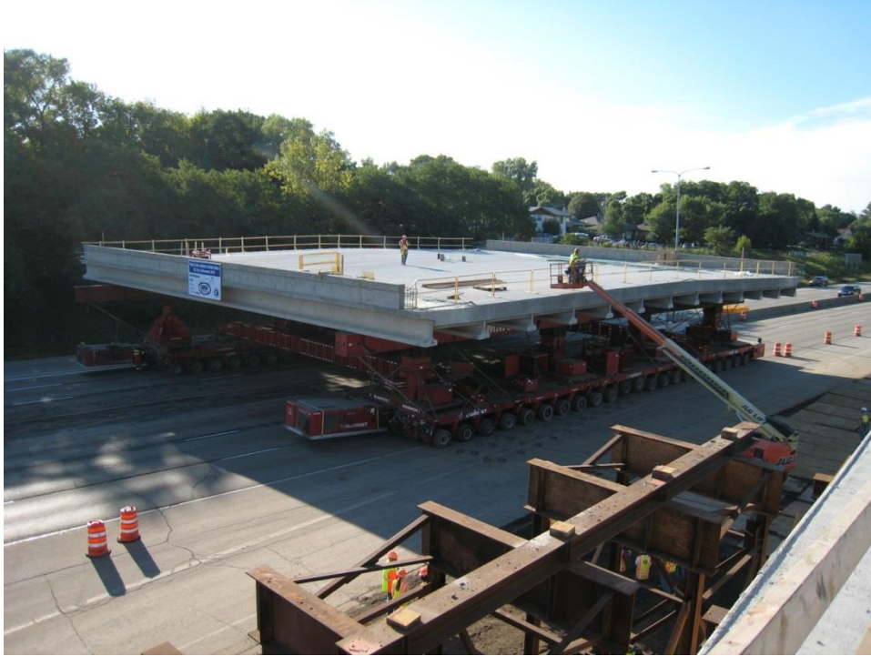
Figure 68. Photo. Another view of moving the first span of Maryland Ave. bridge 62626 on I-35E using the SPMT.
