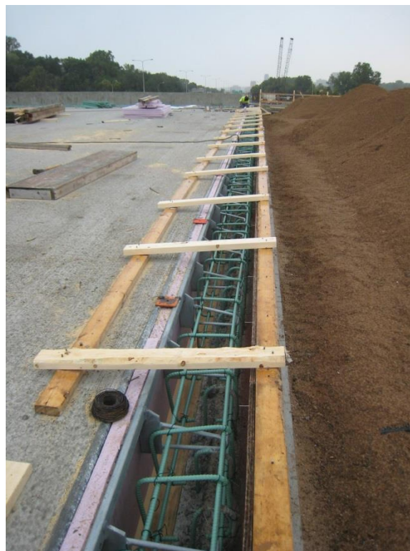
Figure 80. Photo. The end block and expansion joint gland were placed after the bridge was moved into place. This figure shows setting the reinforcing steel and forms for the abutment end block concrete.
