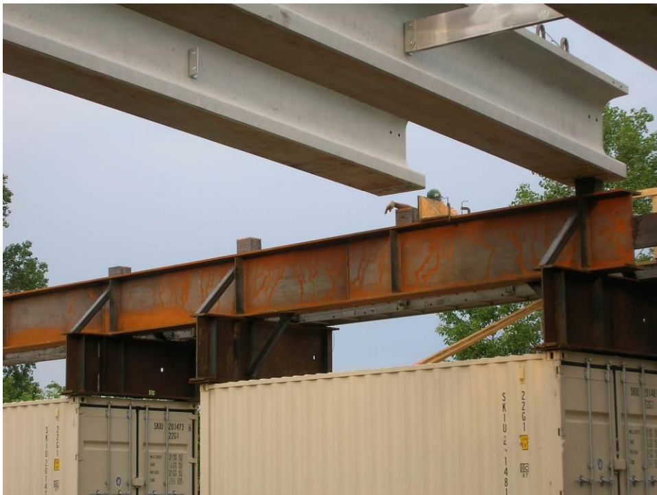
Figure 18. Photo. Each girder was positioned into place as per plans onto the bearing pads using a reference plate.
