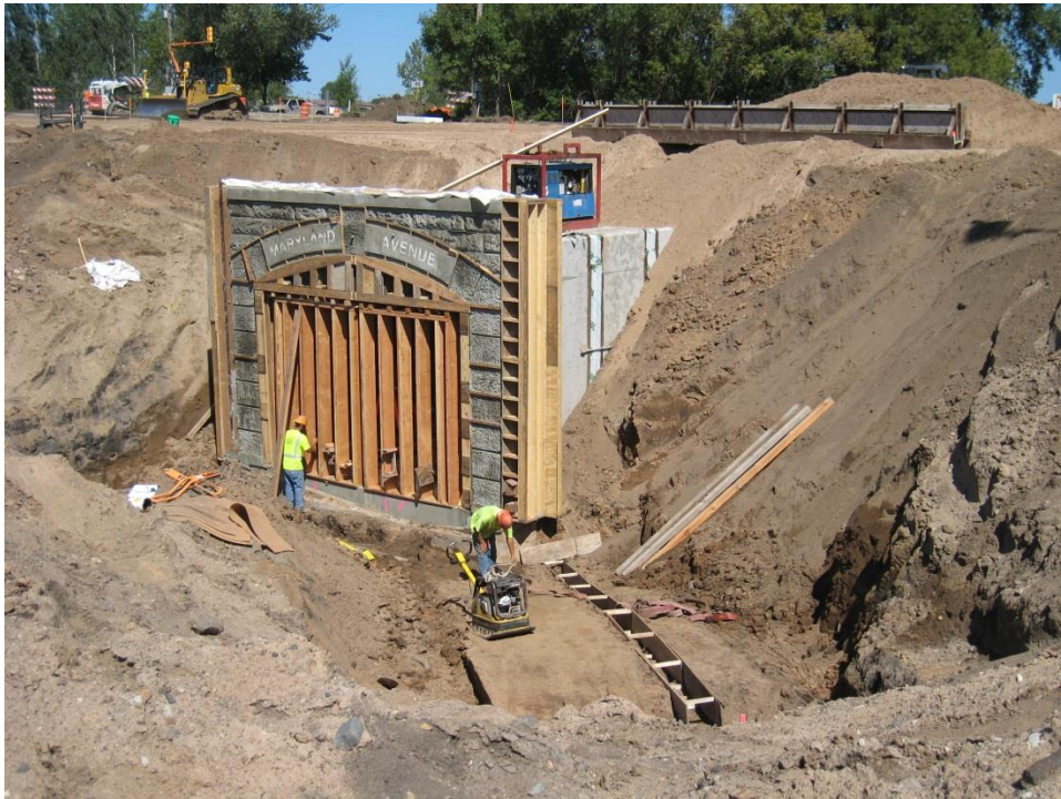
Figure 56. Photo. The north and south facades and the wingwalls for the box culvert bridge tunnel beneath Maryland Ave. were cast in place using wooden forms.
