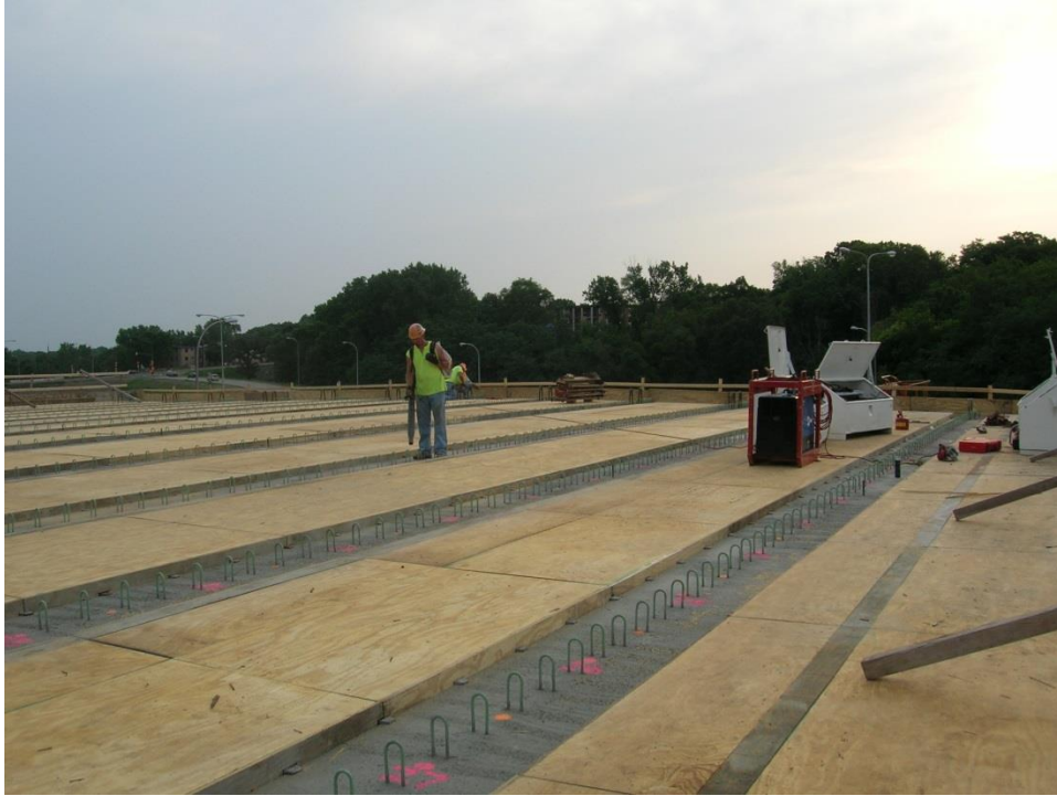
Figure 27. Photo. Finished view of the wooden forms placed between the concrete girders to form the concrete bridge deck and the concrete haunches.
