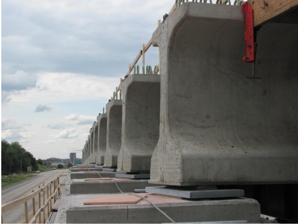
Figure 74. Photo. All girders of the first span resting on the bearing plates supported by the pier after removal of the SPMT support.
