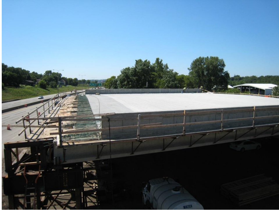
Figure 39. Photo. Completed view of span 1 of the bridge superstructure after placement and curing of the bridge deck and curb concrete. Note the reinforcing steel that will be used to reinforce the closure pour between the two deck spans.
