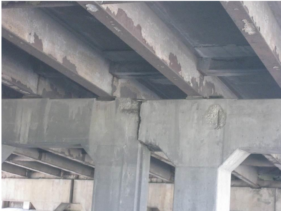
Figure 3. Photo. Delaminated and spalled bent caps of bridge 6513.
