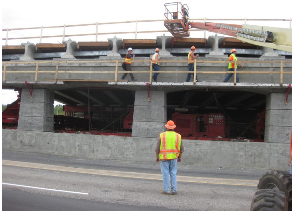
Figure 73. Photo. Checking the final position of all girders before the SPMT released the first span load on to the pier and the abutment.
