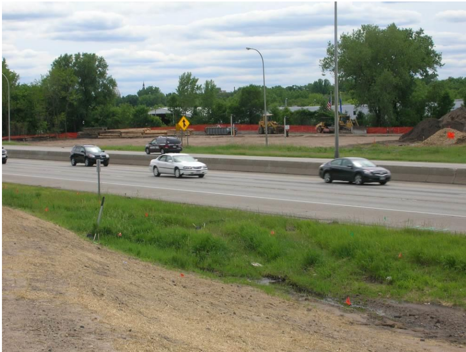
Figure 10. Photo. View of staging area (from across I-35E) for bridge 62626 superstructure construction alongside southbound I-35E.
