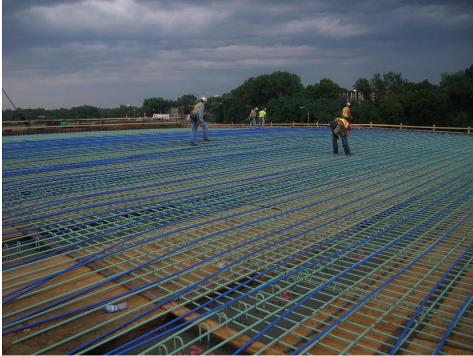
Figure 29. Photo. Placing the post-tensioning cables above the first layer of reinforcing steel.
