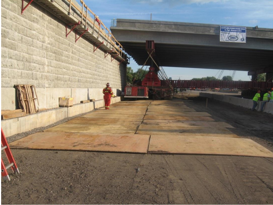
Figure 76. Photo. The problem of the soft soils was resolved during the move of the second span by using 0.5-inch-thick steel plates above the soil to support the SPMT wheels.
