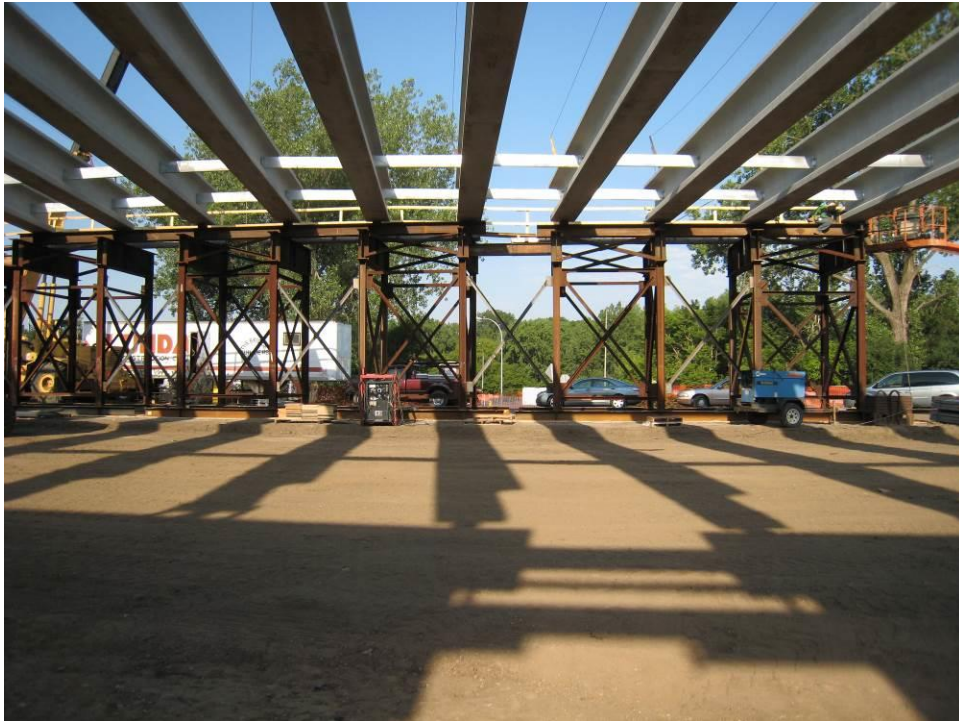
Figure 22. Photo. View of span 1 of the bridge superstructure from beneath following placement of the girders before construction of the deck.
