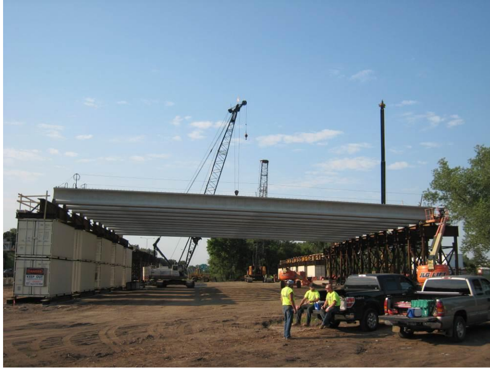
Figure 23. Photo. Side view of span 1 of the bridge superstructure following placement of the girders before construction of the deck.
