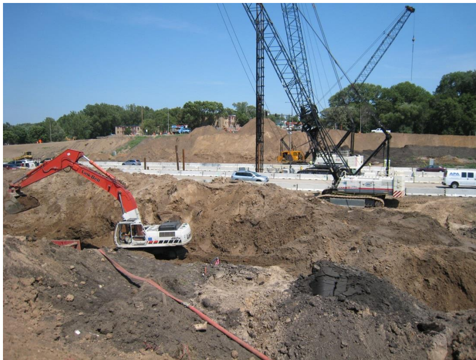
Figure 43. Photo. Earthwork (foreground) and pile driving (background) in preparation for constructing the abutments and midspan pier. Note the open traffic lanes on I-35E.
