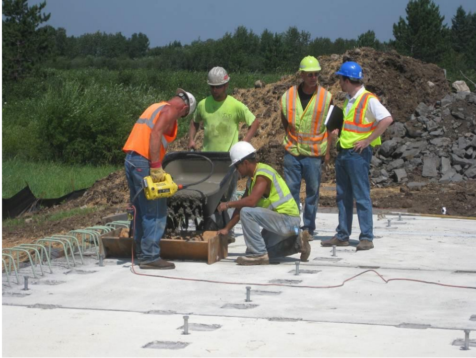
Figure 50. Placing the grout into the keyway joint and post-tensioning duct splice blockouts between the transverse deck panels.
