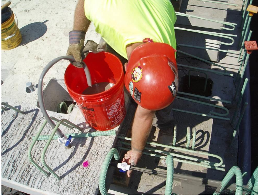
Figure 66. Grout pumped and continuously discharged at the anchorage and grout cap outlets.
