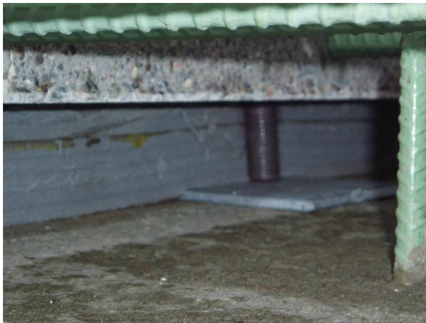
Figure 33. Leveling bolt resting on the steel plate on top of the girder.
