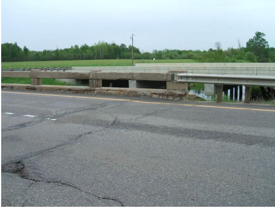
Figure 2. Deterioration of bridge 6603 surface and parapet walls.
