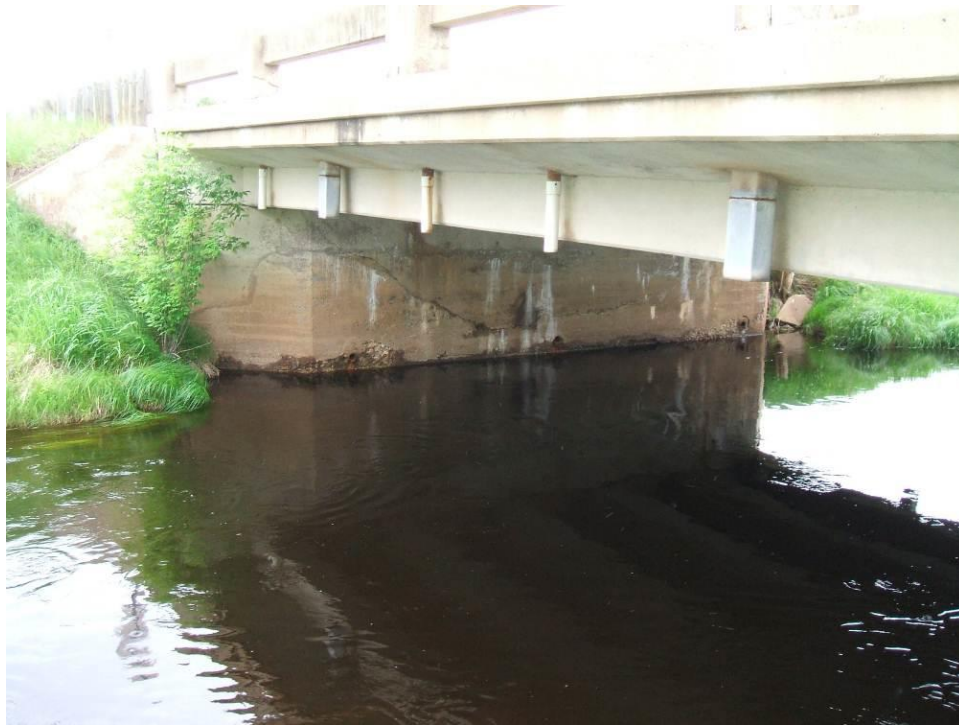
Figure 4. Deterioration of bridge 6603 north abutment wall.
