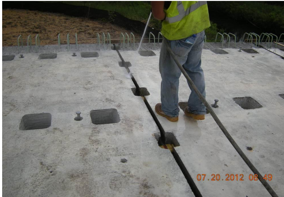
Figure 46. Cleaning the keyway joints and post-tensioning duct splice blockouts in preparation for pouring concrete.
