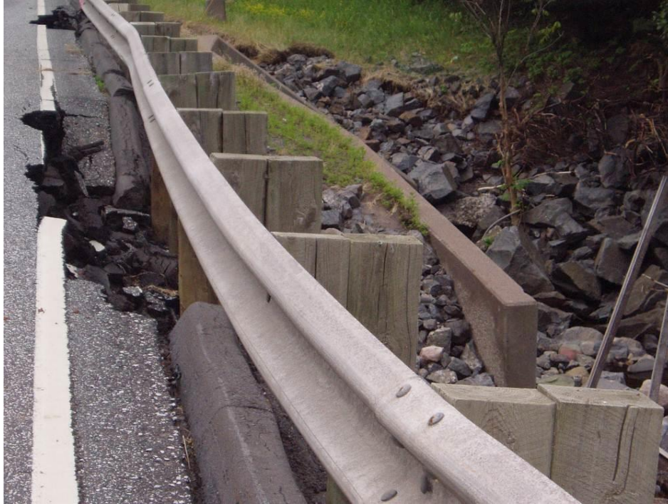
Figure 76. Small shoulders on the old bridge resulted in an increased chance of crashes and structural damage due to errant vehicles.
