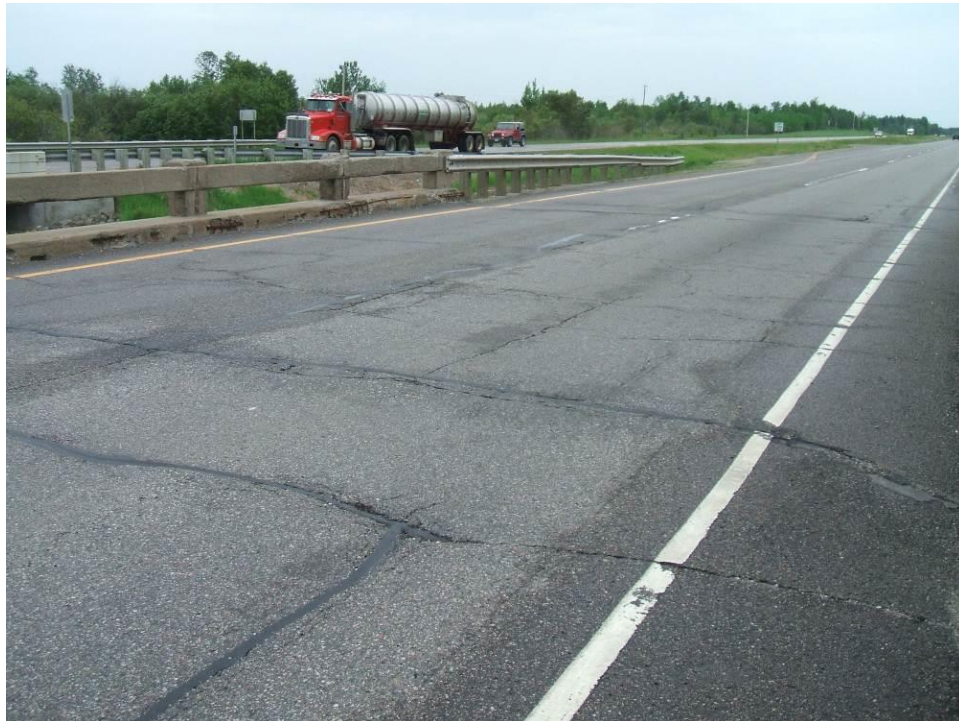
Figure 1. Deterioration of bridge 6603 surface and parapet walls.
