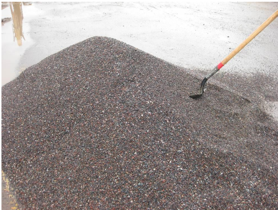
Figure 47. Aggregate used for extending the grout for the keyway joints and post-tensioning duct splice blockouts.
