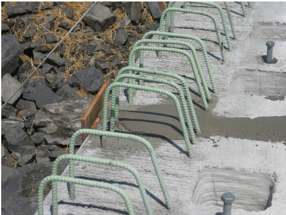
Figure 53. Forms at the edge of the transverse keyway joint between the deck panels to contain the grout.
