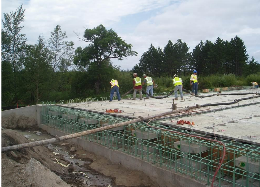
Figure 68. Grouting the haunches and the shear pocket blockouts by pumping extended grout through the shear pocket blockouts.
