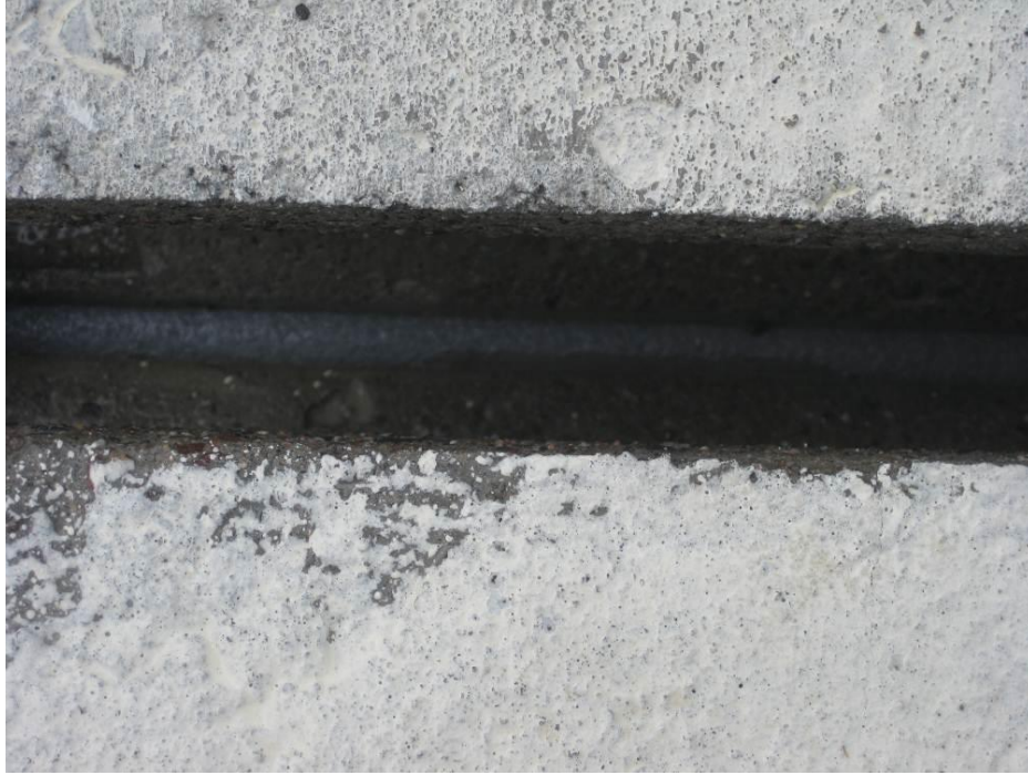
Figure 42. View of the backer rod from the top of the deck panels. The backer rod prevents the grout poured into the transverse joint keyway from escaping.
