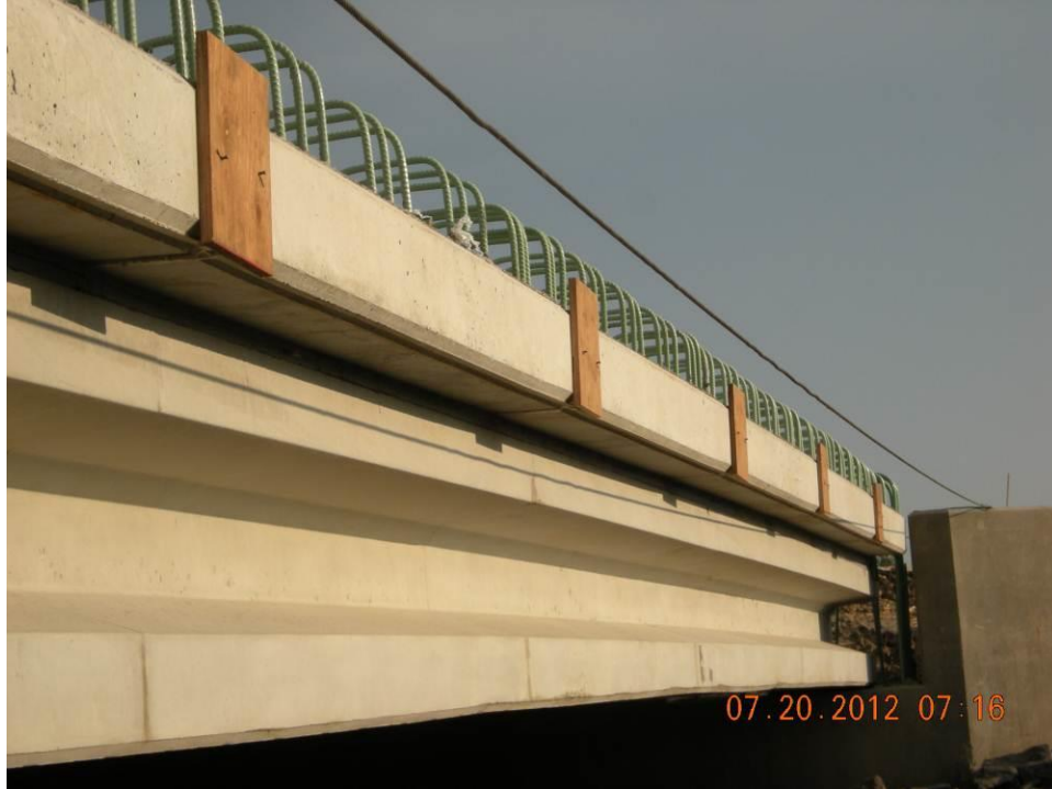
Figure 52. Forms at the edge of the transverse keyway joint between the deck panels to contain the grout.
