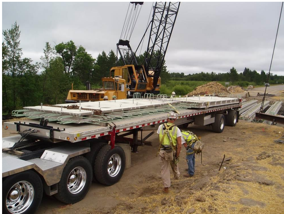
Figure 21. Precast deck panels tied to flatbed trucks on wooden supports for transportation to bridge site.
