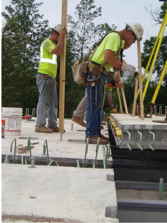
Figure 34. Placement of the second deck panel to align with the first deck panel.
