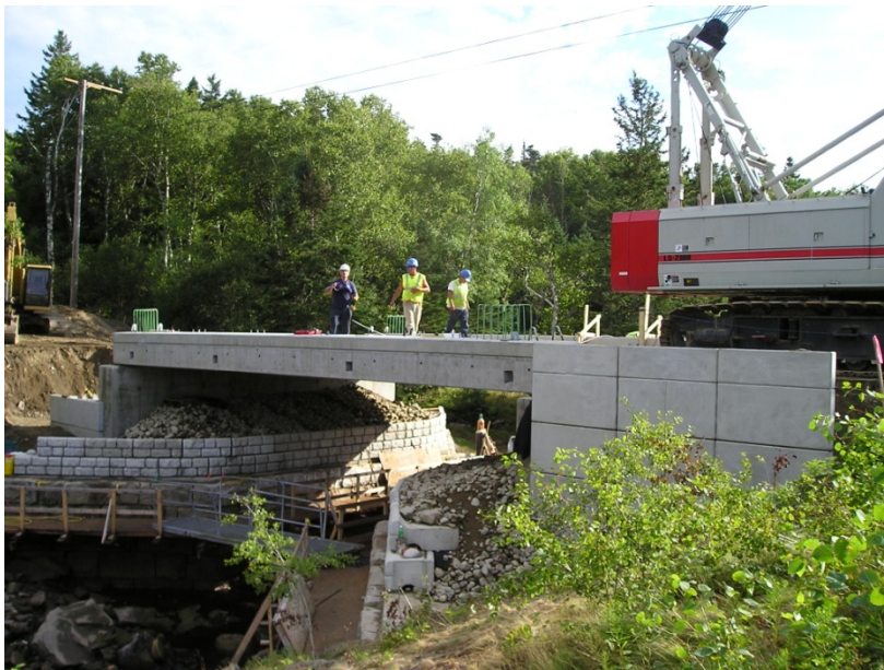
Figure 8. Looking westbound on the Lamson Bridge construction site. Note the precast concrete backwall, the precast, segmental retaining wall panels, and the post-tensioning duct pockets in the fascia beam.
